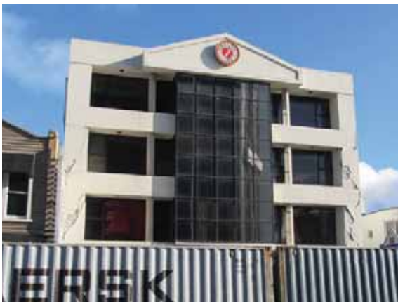
Figure 7: An Indicator Building in Christchurch after the February earthquake (source: draft ATC Reconnaissance Team report, 2012)
