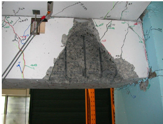
Figure A-8: Spalling of support ledge in cover concrete in a plastic hinge (Lindsay, 2004)
