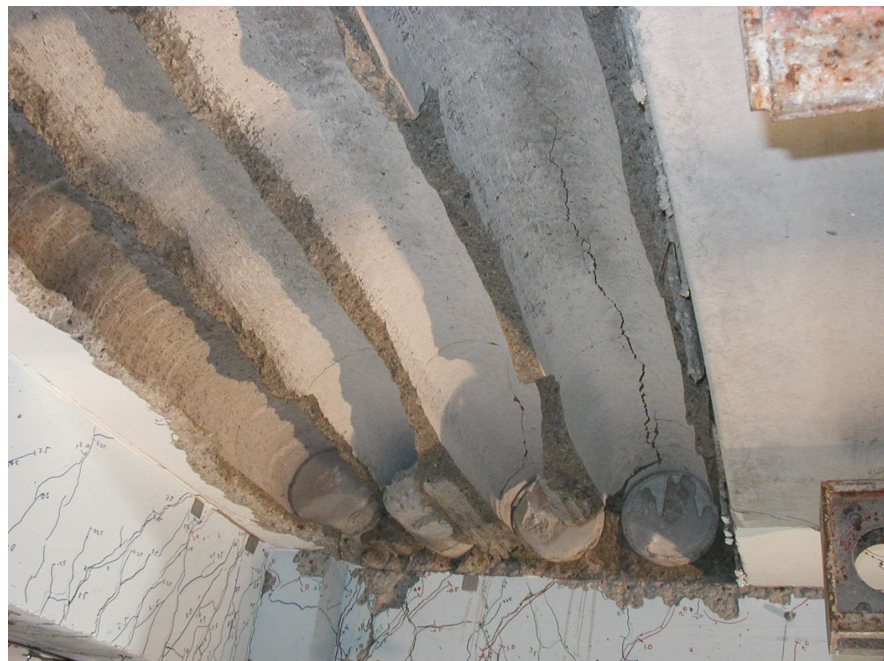
Figure A-29: Web splitting seen after failure of lower portion of hollow-core unit [Matthews, 2004]
