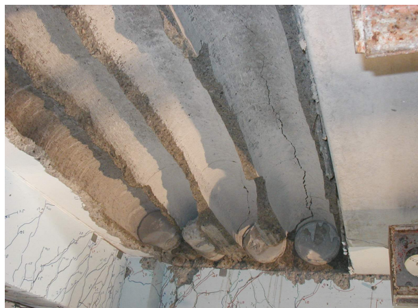
Figure 5-13: Splitting of webs due to differential displacement between a beam and adjacent hollow-core unit (Photo from reference 9)
