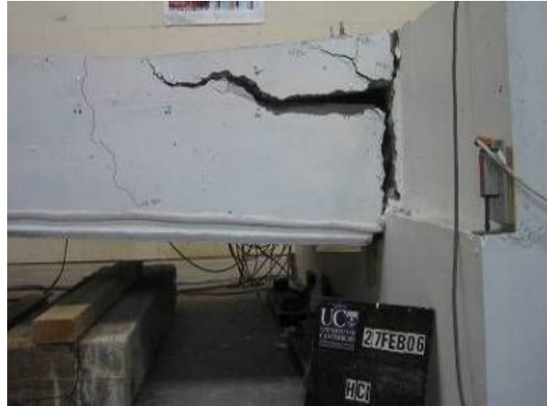
Figure A-12: Separation of insitu concrete topping and hollow-core unit when support reaction is transferred to topping concrete.
