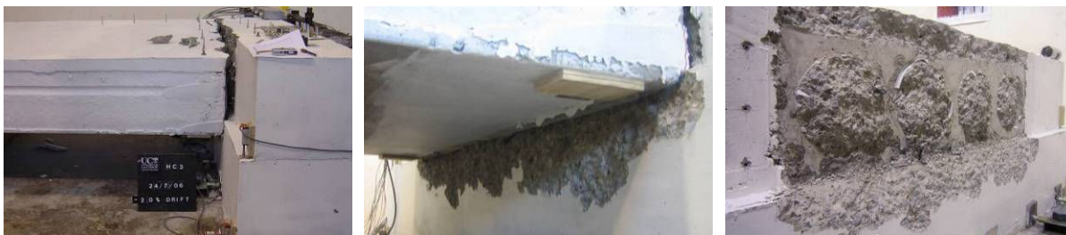
a) Collapse of HC3 at -2.0% drift b) Underside of HC3 test specimen c) HC3 seating beam post test
