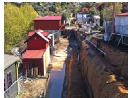
Cunningham Terrace, Lyttelton: the retaining wall is being rebuilt using ground anchors to increase its strength.
