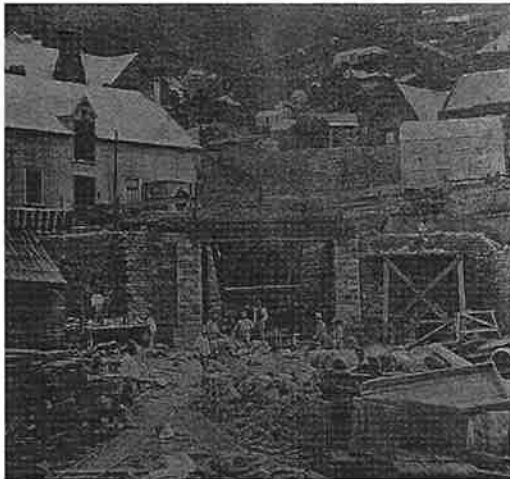
Figure 7. The portal of the Lyttelton rail tunnel during construction, in February 1867. Edward Dobson, Provincial Engineer, is the figure with the white top hat, centre right. The rail link made Lyttelton a suburb of Christchurch and became the economic lifeline of Canterbury Province. D. L. Mundy photograph, CM 9200
