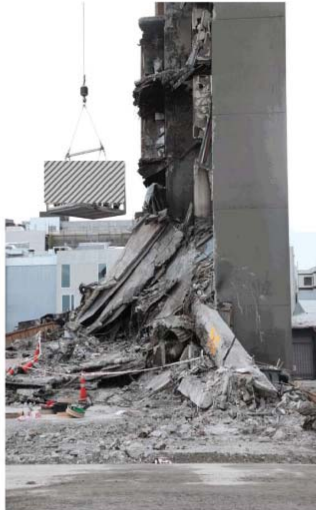
Figure 165 - North Core slabs leaning against the North Core showing that their collapse occurred after collapse of the Line 3 frame
