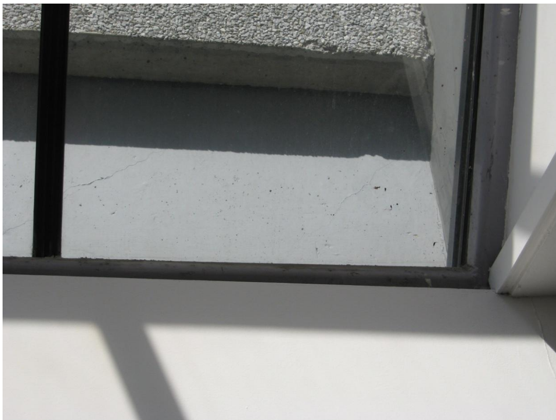
Photo 5 Cracking in first floor beam north elevation over entry.
