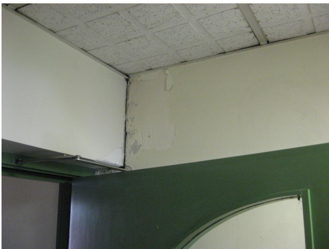
Photo 10 Partition lining damaged at junction with concrete beam.
