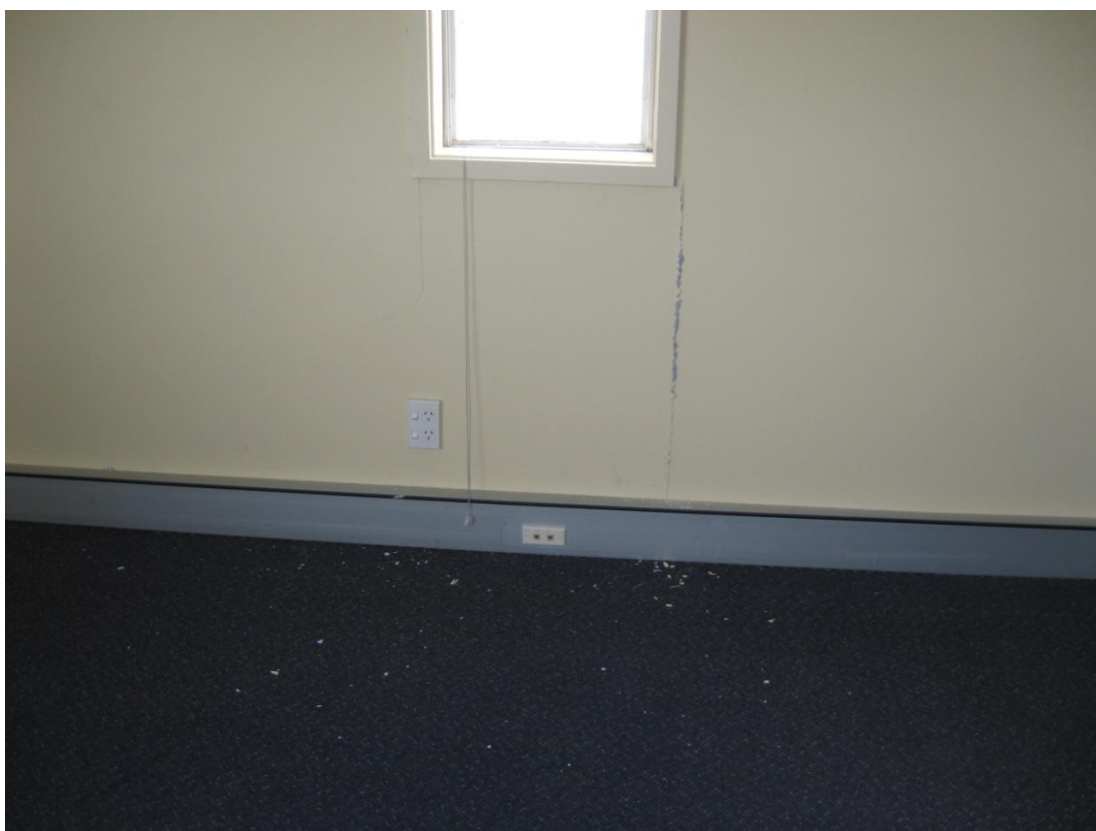
Photo 12 Crackling in linings under window.
