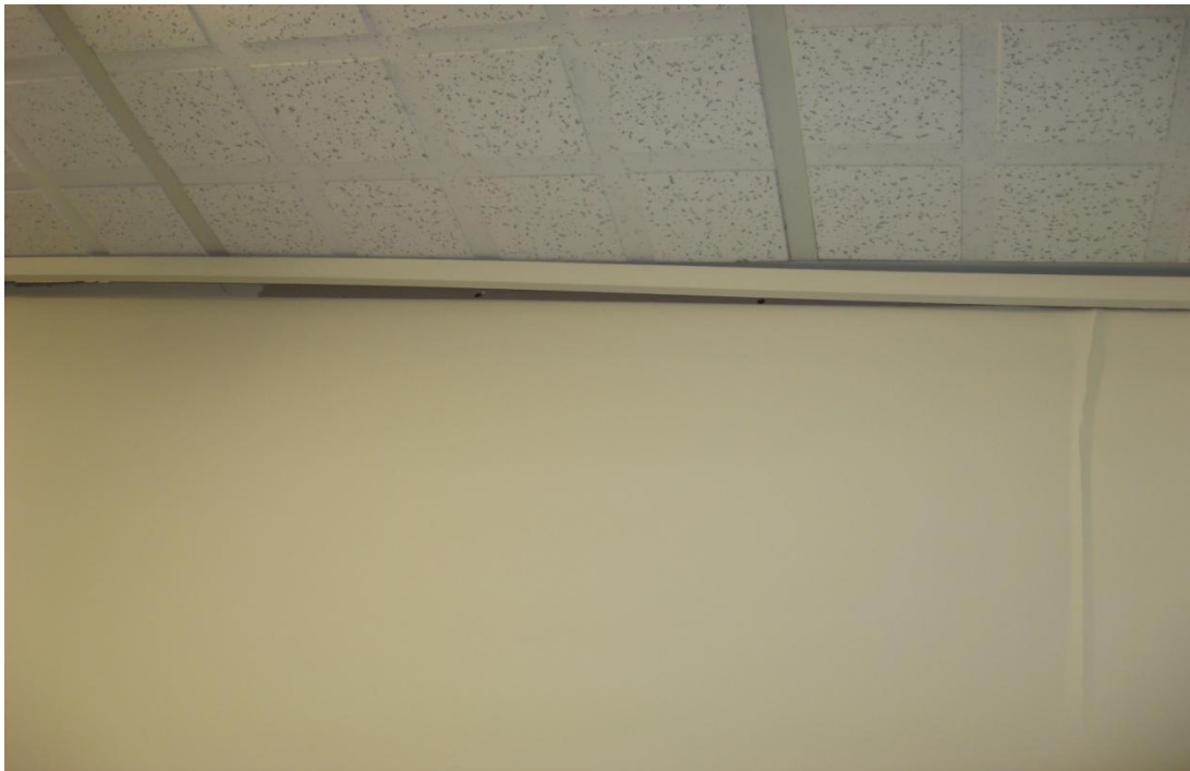
Photo 14 Cracked wall lining and damaged ceiling coving.
