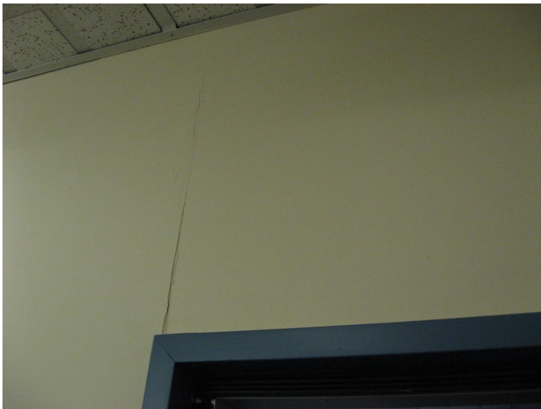
Photo 11 Cracking in linings over door head
