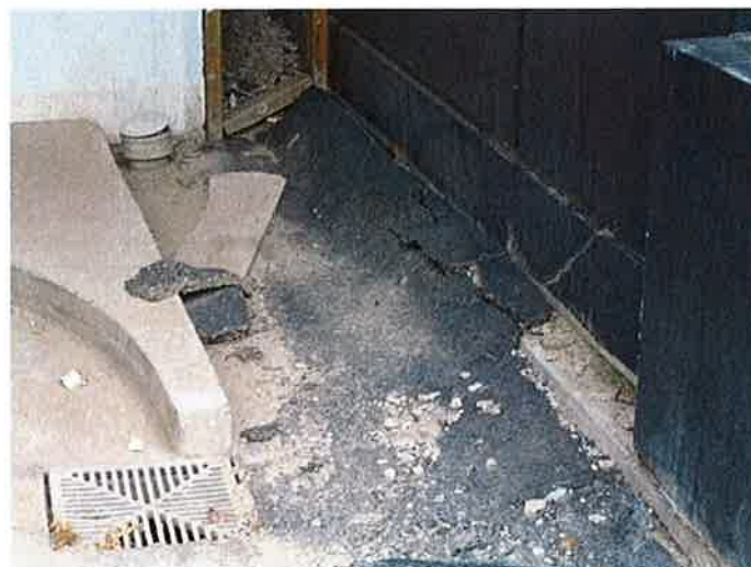
Damage to ground adjacent to the building at 100 Armagh Street
