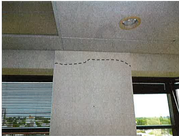
Horizontal crack to column typical above level 7
