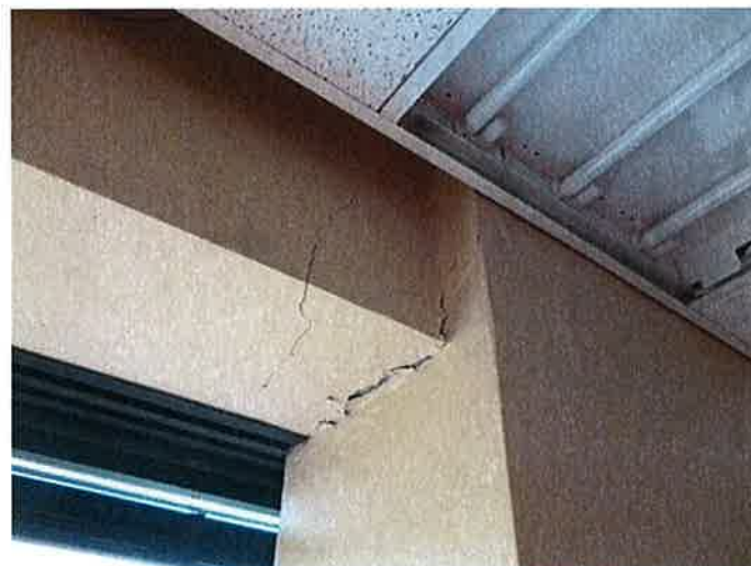
Typical single crack to beam column joint
