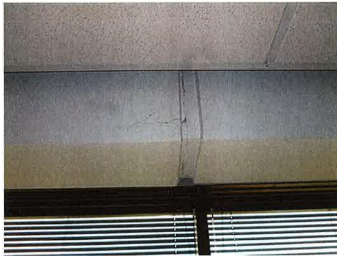
Cracking at insitu splice to beam
