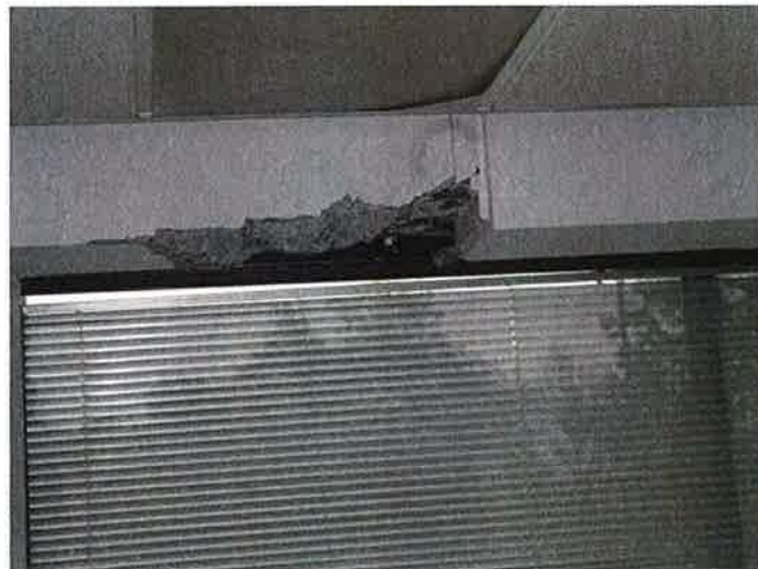
Spalled concrete to insitu splice of beam
