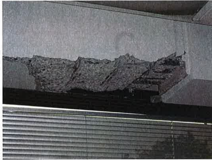
Spalled concrete to in-situ splice of beam
