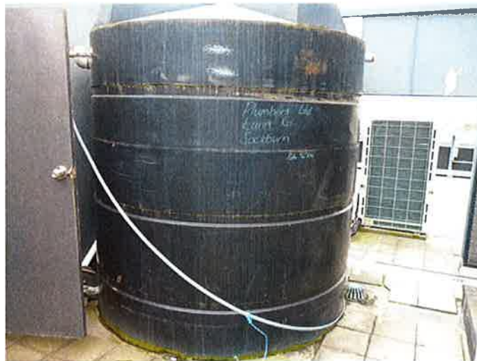
Strapping to water tank to roof loose
