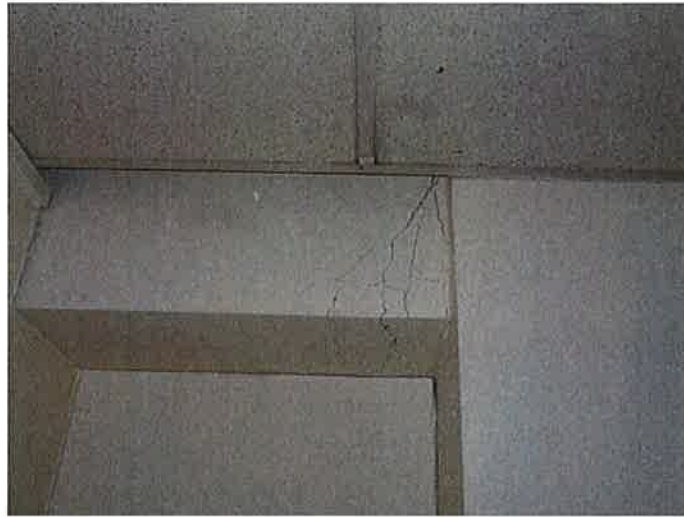
Fan cracking to beam adjacent to column
