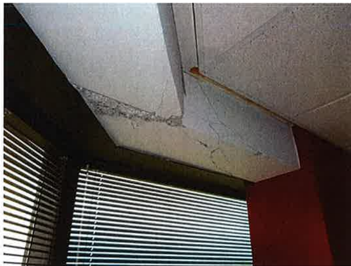
Damage to corner beam
