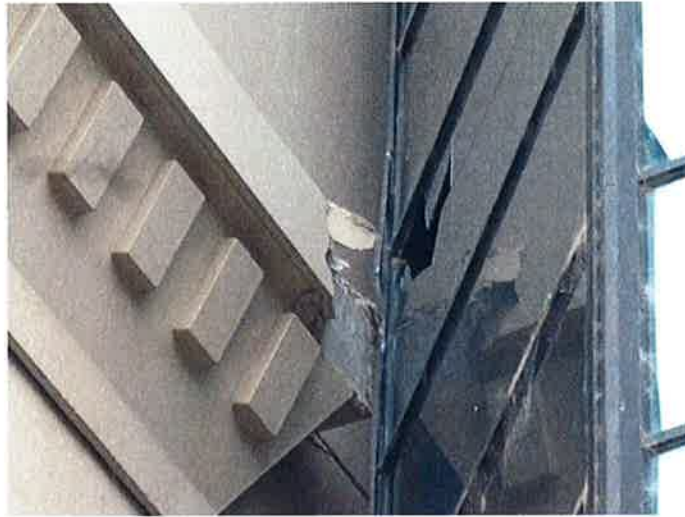
Close view of pounding damage
