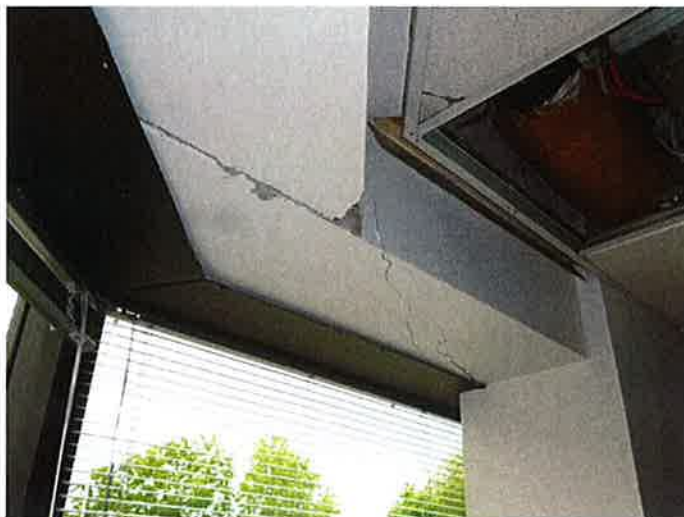
Damage to corner beam
