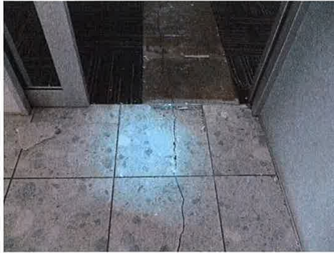
Floor diaphragm crack
