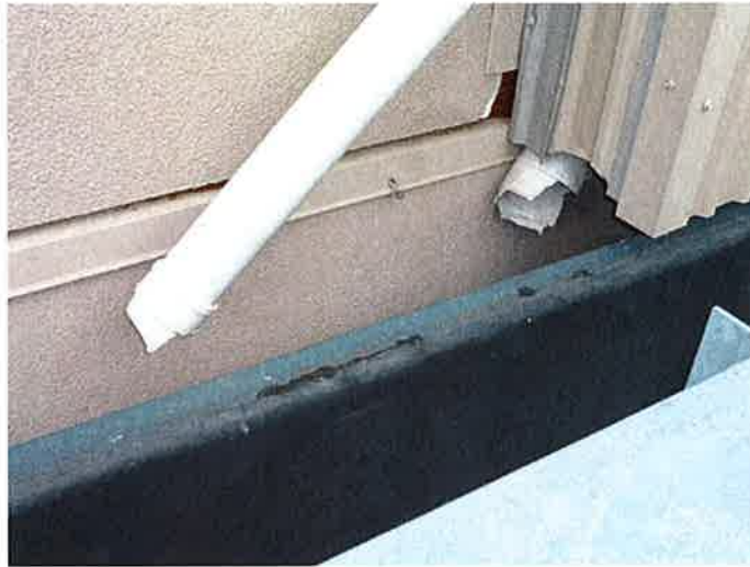
Broken drainage pipe to building at 100 Armagh Street due to pounding
