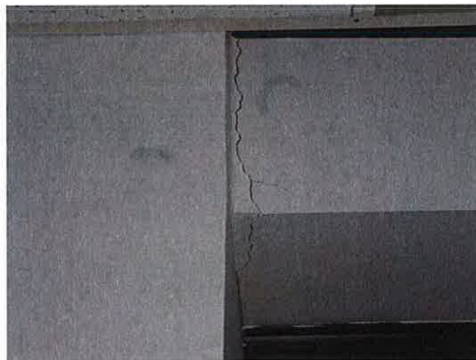
Typical single crack to beam column joint
