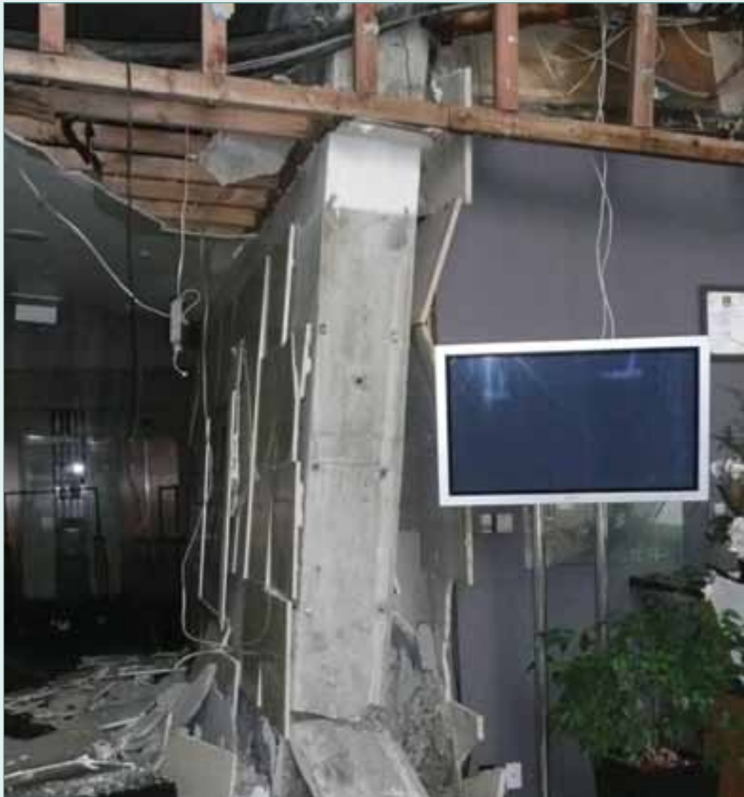
Figure 7.4: Shear wall D5-6 base failure (in the hotel foyer)
