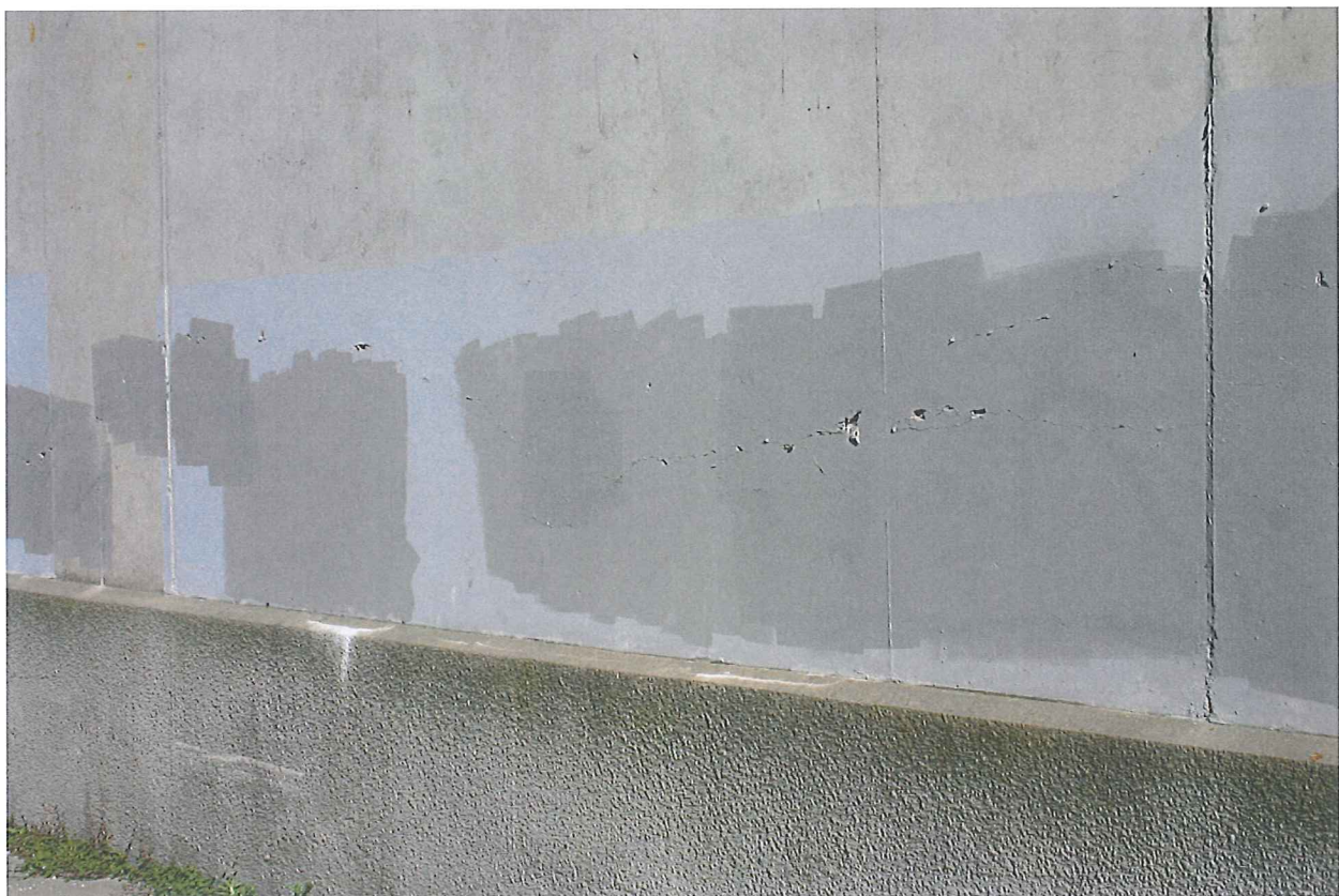
Damage to east wall panels
