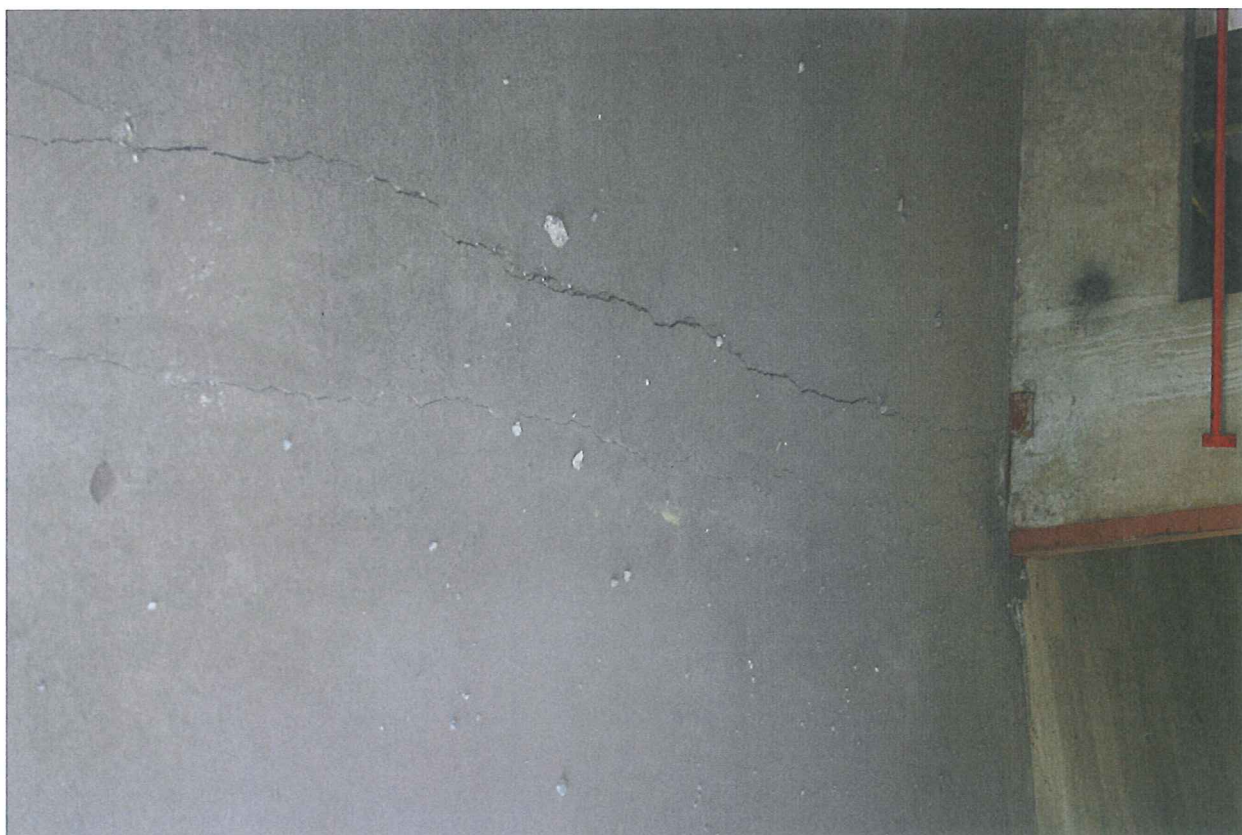
Damage at ramps
