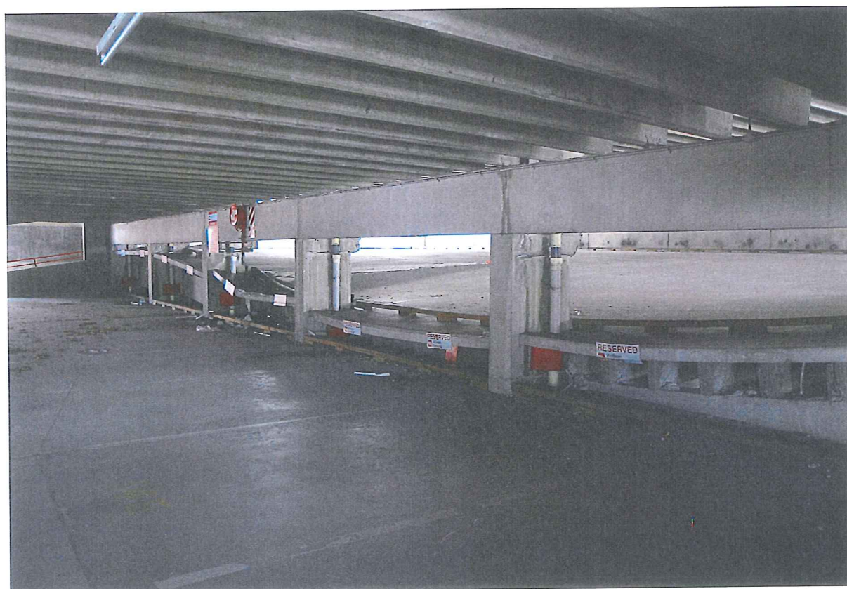
Failure of level 3 floor, viewed from level 2
