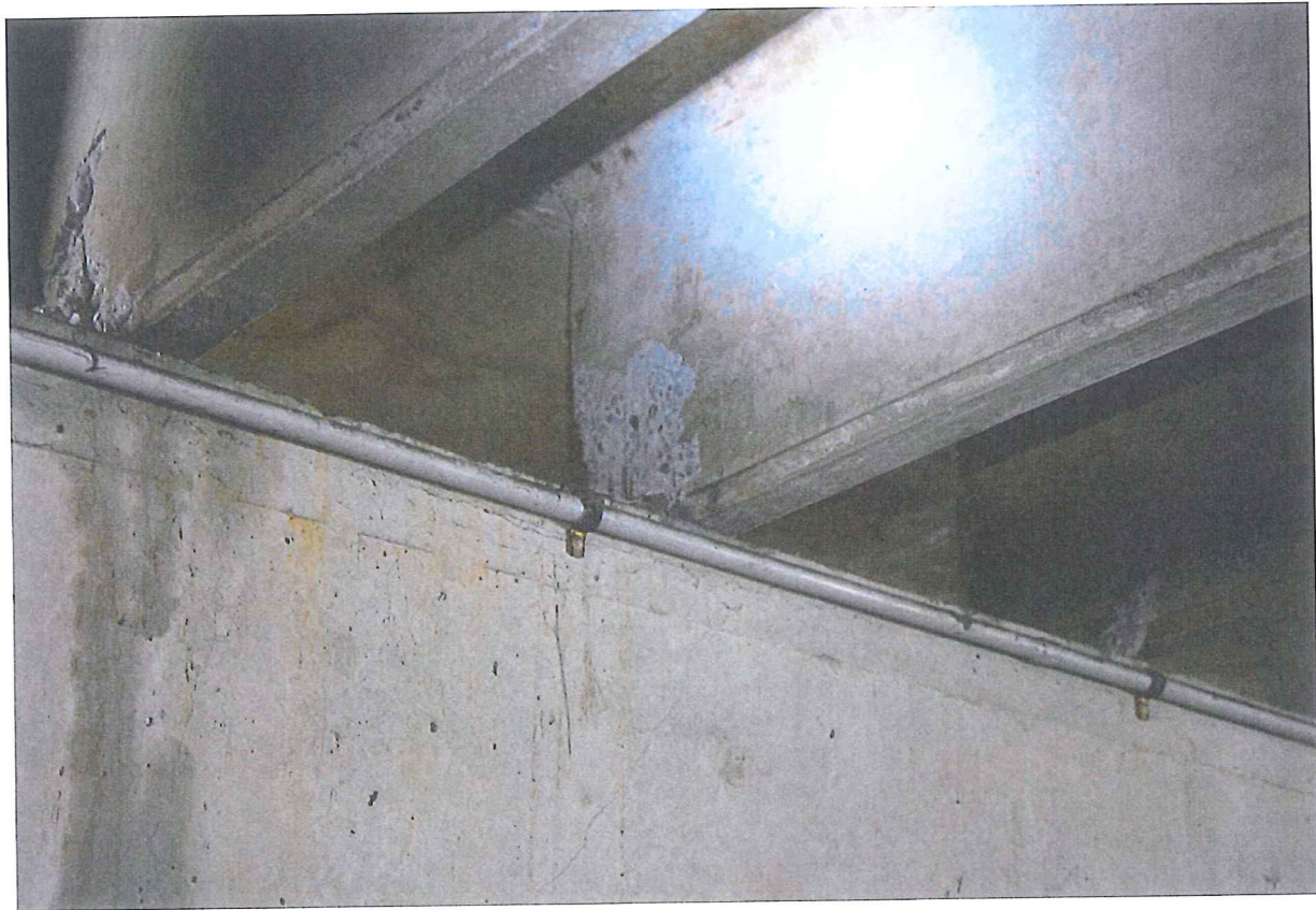
Damage to Double Tee flooring units
