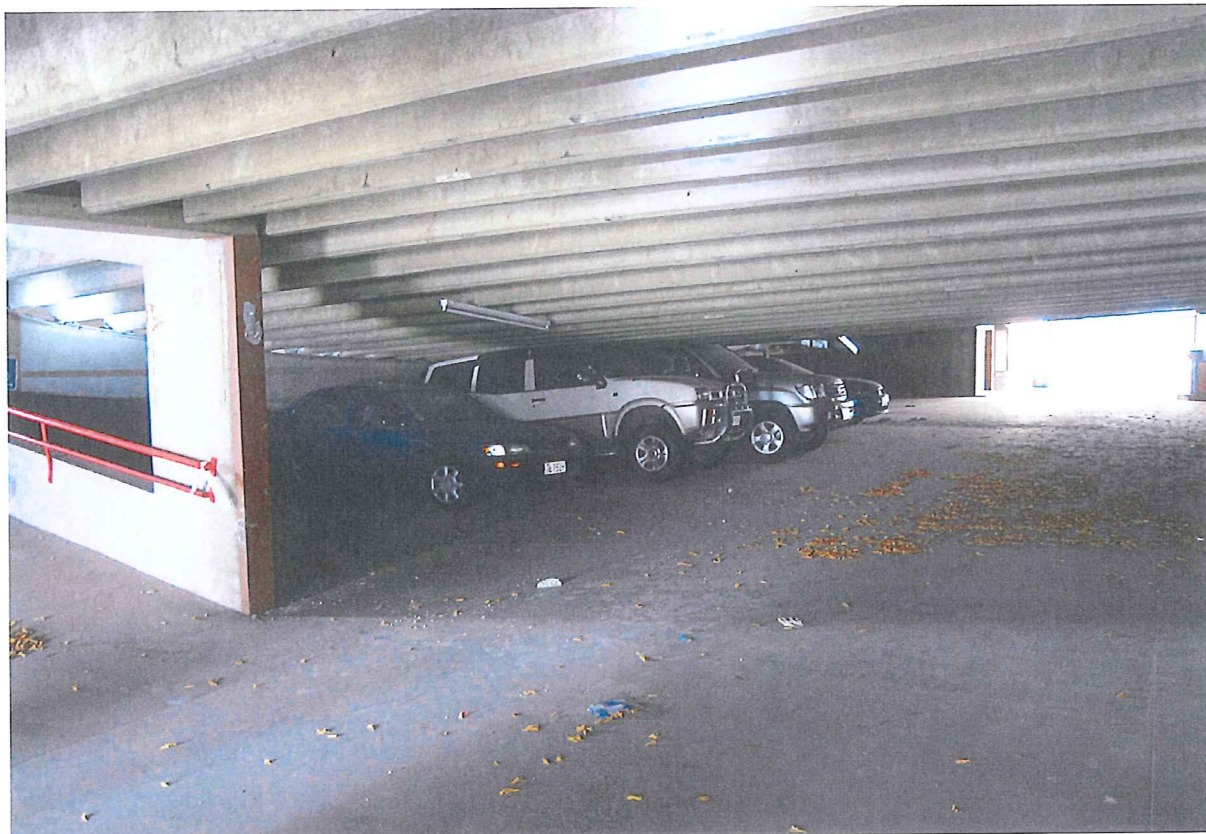
Failure of level 3 floor, viewed from level 3
