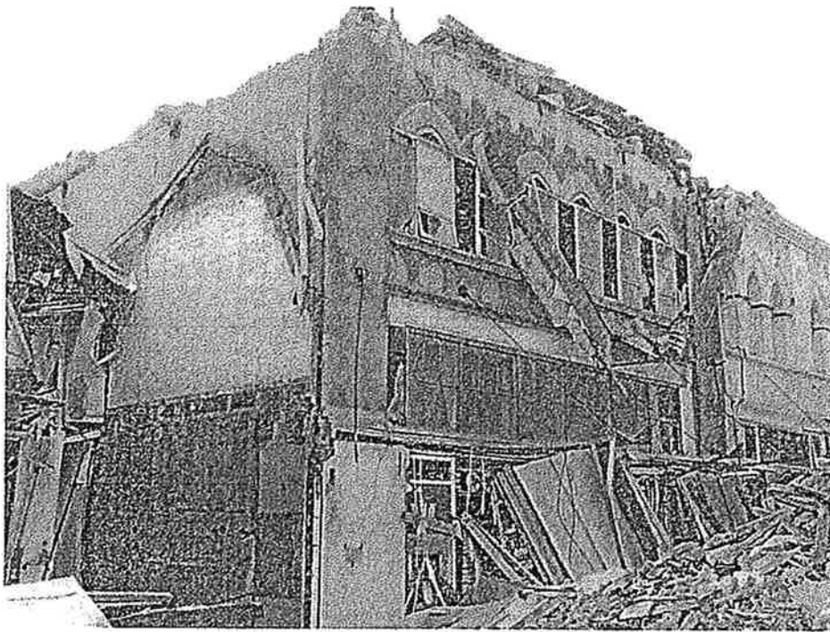
Photo 1: Southwest corner of building show loss of 3rd floor, façade glazing and canopy.
