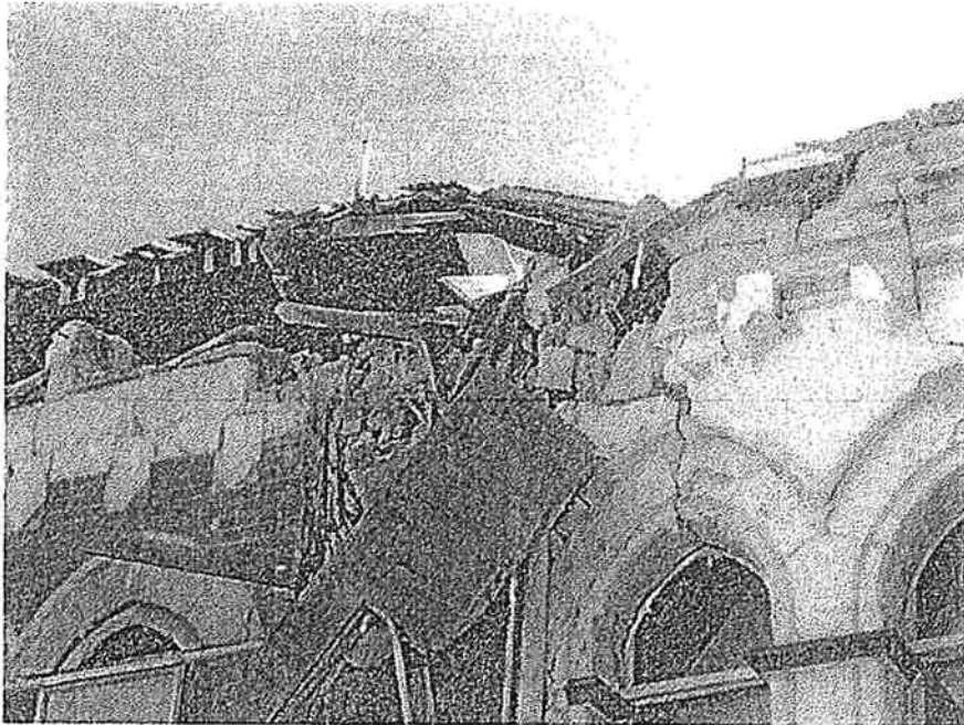
Photo 3: Pounding damage with adjacent building at 2nd floor
