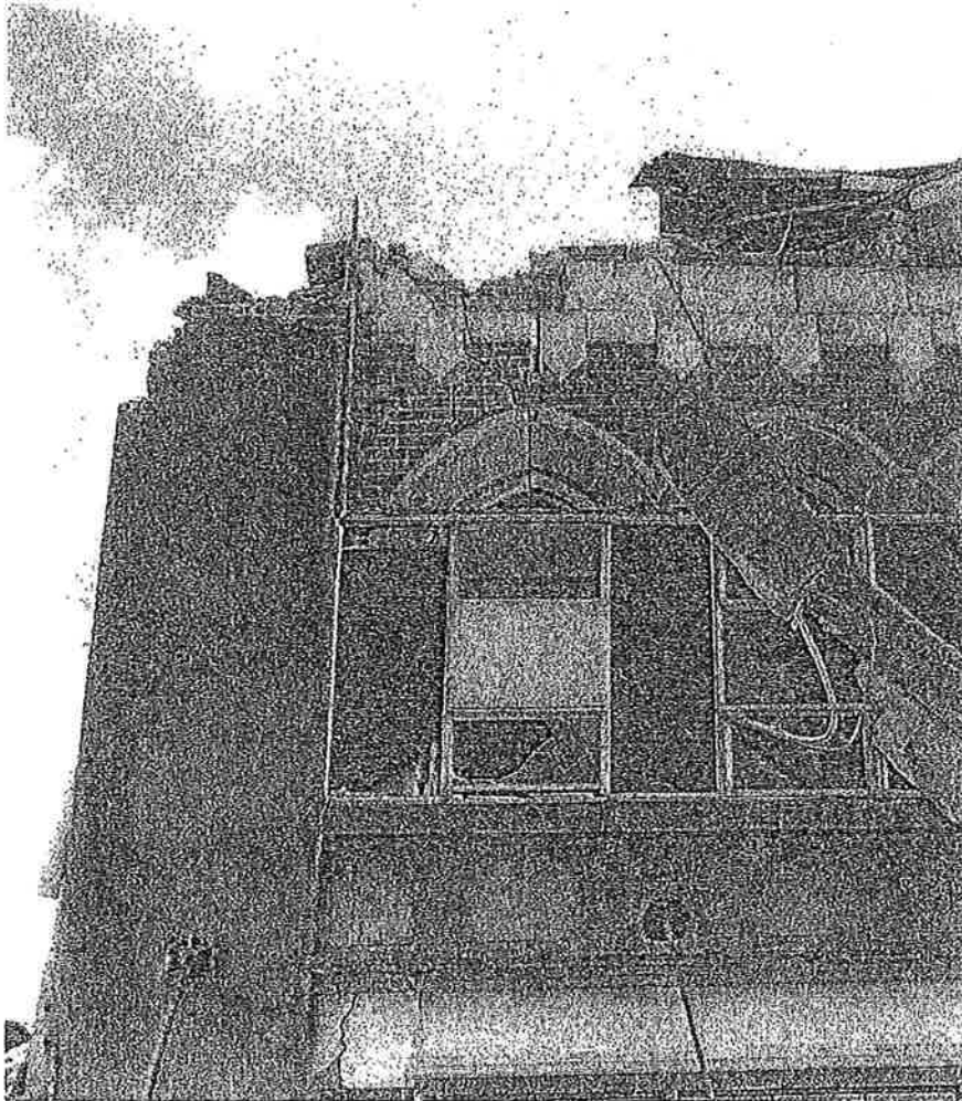
Photo 4: Damage to 1st floor and 2nd floor spandrels
