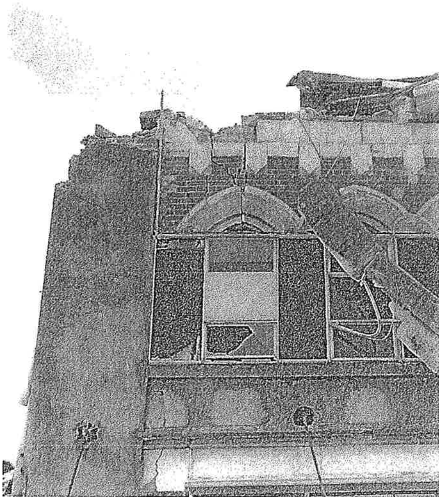
Photo 4: Damage to 1st floor and 2nd floor spandrels
