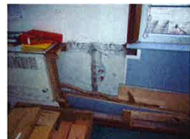
Damaged to Internal Wall showing original brickwork
