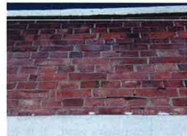
North Elevation detail of weathered brickwork
