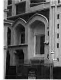
Service Bay Ground Floor Door and Window
