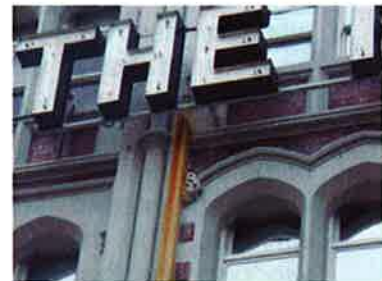
Rusting connections behind 'The Press' Sign
