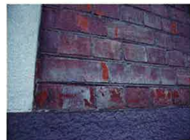
Detail showing milky coating on brickwork
