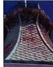
Tower Roof and Crows Nest showing rusting on copper cladding
