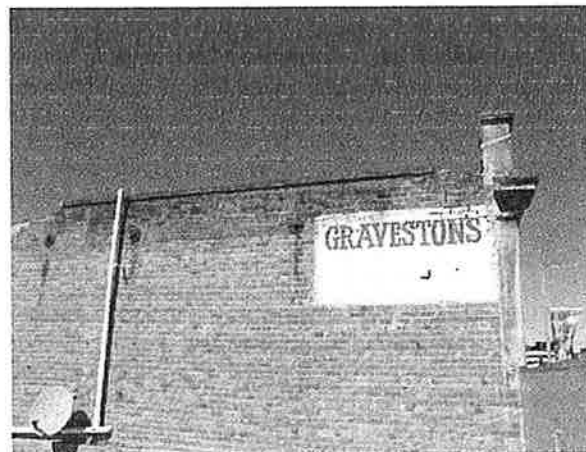
Figure 2: Damage to brickwork.
