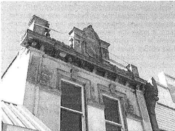
Figure 1: View of ornate parapet that has been damaged.
