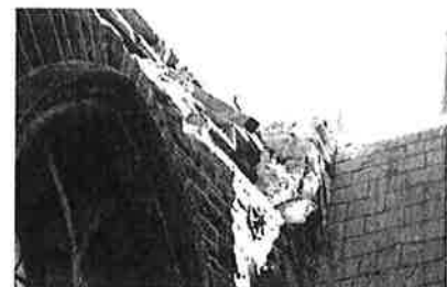
Hall east wall damage
