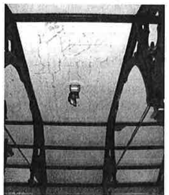
Cracked ceiling in auditorium
