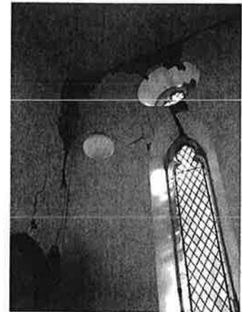
damage to auditorium stair walls, east end
