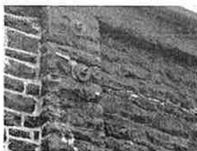
crack along west wall
