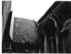
damaged entry roof & collapsed east wall
