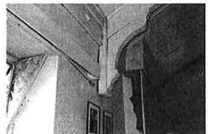
Annex west wall displaced from Truss
