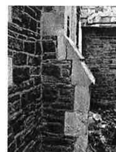
Displaced stones to east wall buttress
