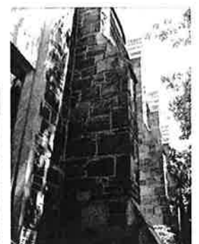
north wall cracked buttresses
