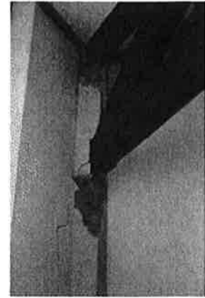
Spalling of stone around gallery beams in Auditorium
