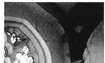
side wall & Tower wall spalling plaster
