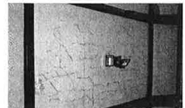
cracked lath & plaster ceiling
