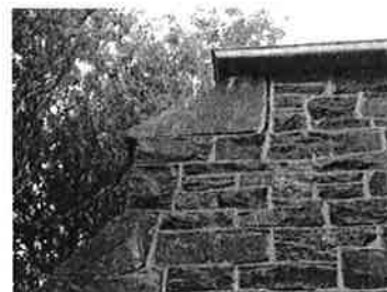
North wall buttress displaced stone
