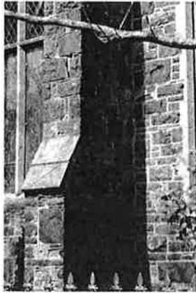
Cracks to mortar joints in Auditorium buttresses
