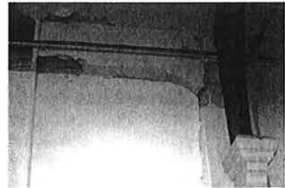
Cracks to the infill stone walls in Hall
