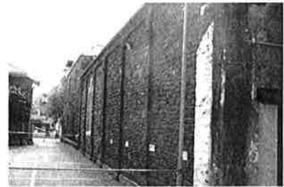
west wall of Hall leans out
