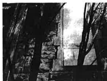
Damaged stone to north tower window
