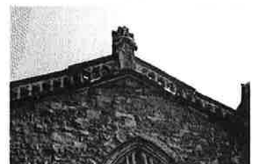
dislodged east gable parapet & finial
