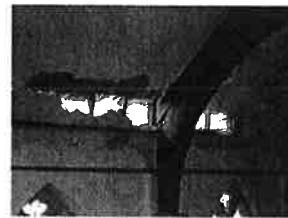
damaged ceiling & bulkhead
