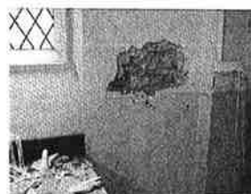
horizontal crack east wall 1250mm above floor
