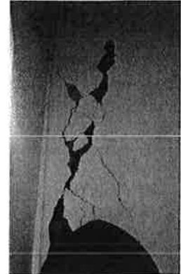
cracked & spalling plaster north tower
