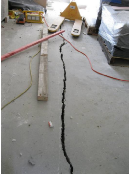
Figure 9: Floor tearing caused by frame elongation
