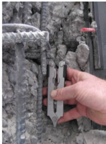
Figure 6: Fractured bars in lightly reinforced wall
