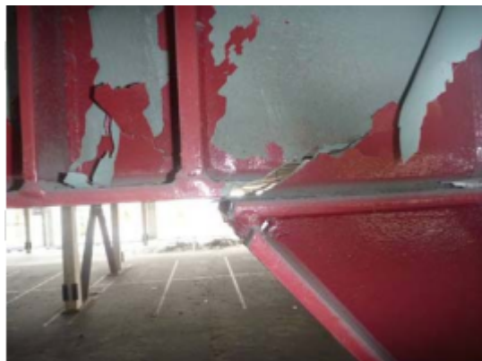
Figure 10: Fabrication eccentricity causing fracture of EBF
