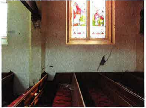
Mezzanine floor support and cracked North Wall
