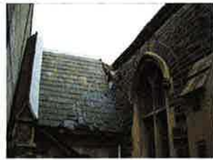
damaged entry roof & collapsed east wall
