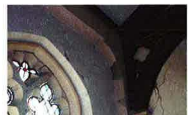
side wall & Tower wall spalling plaster
