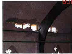
damaged ceiling & bulkhead
