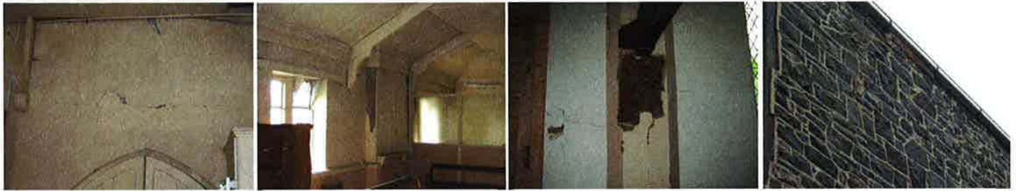
cracks to back of west wall gable
