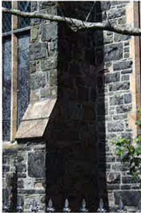
Cracks to mortar joints in Auditorium buttresses
