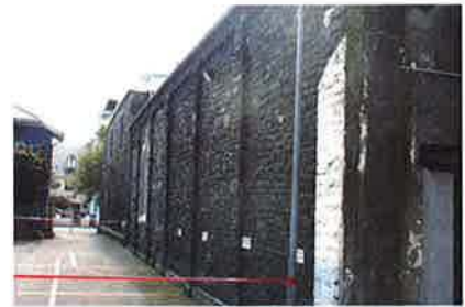
west wall of Hall leans out
