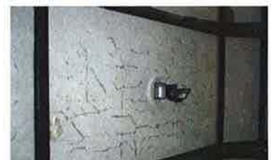
cracked lath & plaster ceiling
