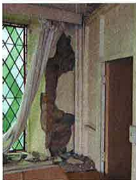
Annex north wall spalling plaster around window
