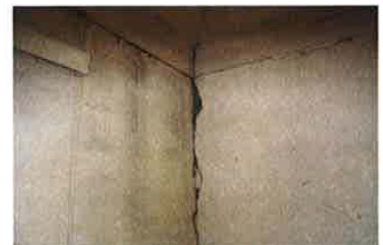
Crack formed in north wall corner of Annex
