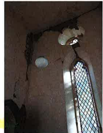
damage to auditorium stair walls, east end
