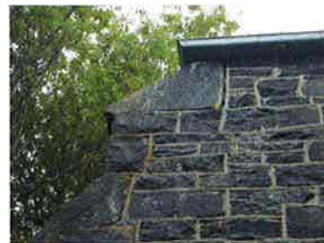
North wall buttress displaced stone
