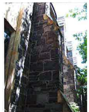
north wall cracked buttresses
