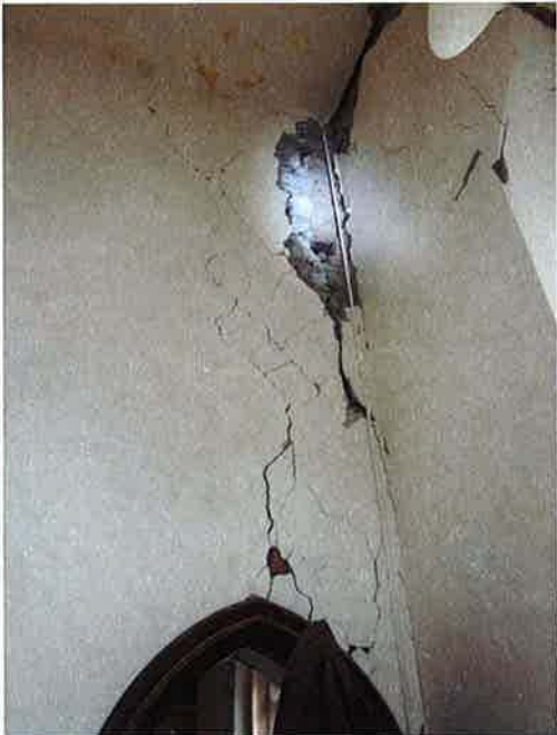
Damage in the East tower
