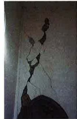
cracked & spalling plaster north tower
