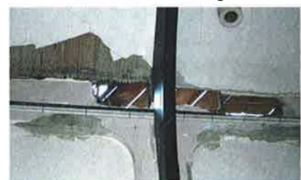
damage at truss locations in Hall
