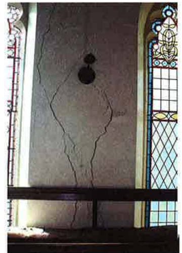
east wall damage
