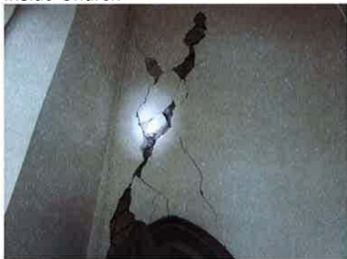
Damage in the East tower
