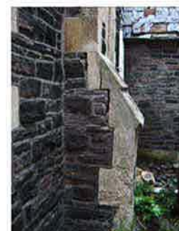
Displaced stones to east wall buttress
