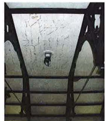
Cracked ceiling in auditorium
