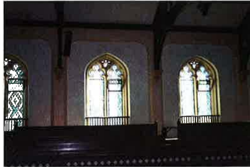
Side walls of Auditorium in good condition with some cracking above windows
