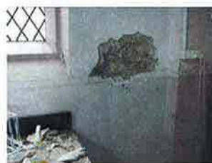
horizontal crack east wall 1250mm above floor
