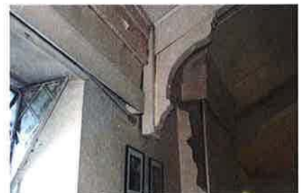
Annex west wall displaced from Truss
