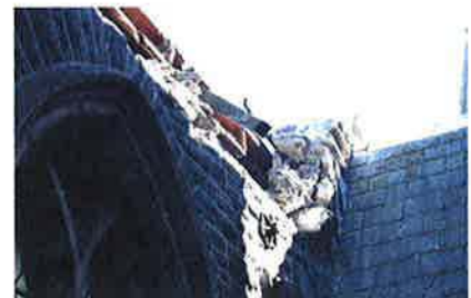
Hall east wall damage
