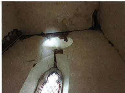
Damage in the East tower
