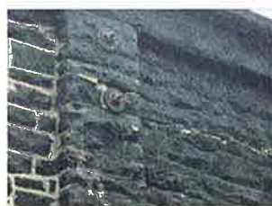
crack along west wall
