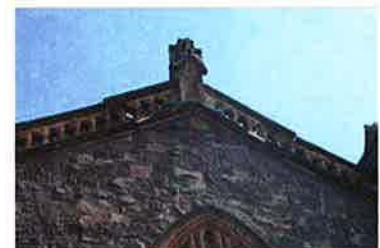
dislodged east gable parapet & finial
