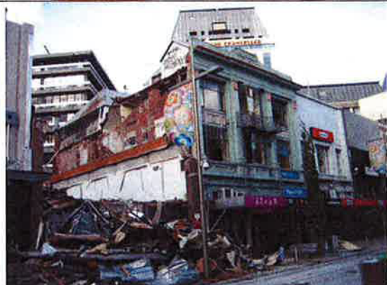
2 – High Street facade on right and north west side wall on left
