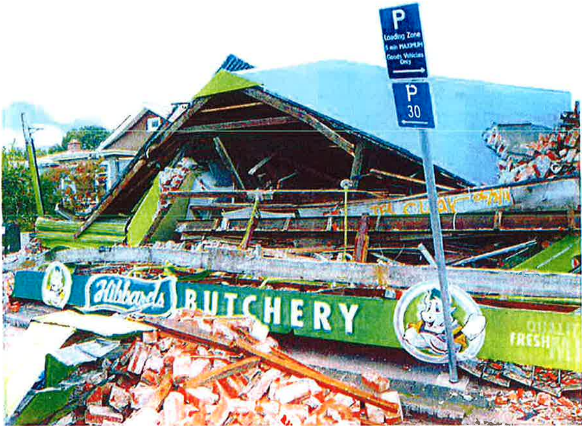
Photo 5 : Collapsed Butchery shop (end of Worcester St. block of shops)
