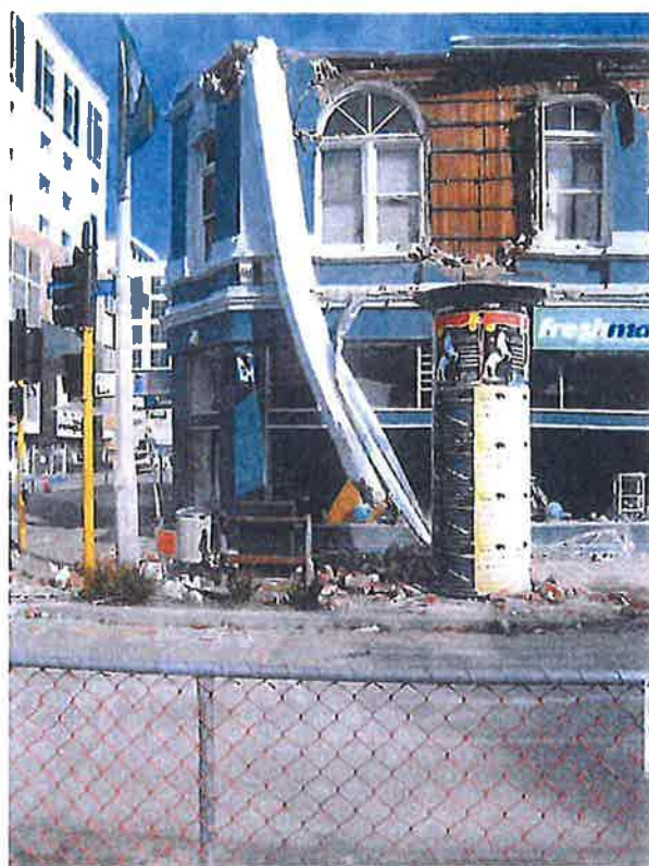
Photograph 2: Corner of the building, showing collapse of the reinforced concrete parapet.
