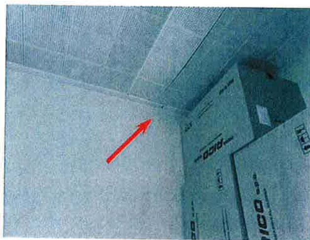
Photo 16. Ceiling NE popped
