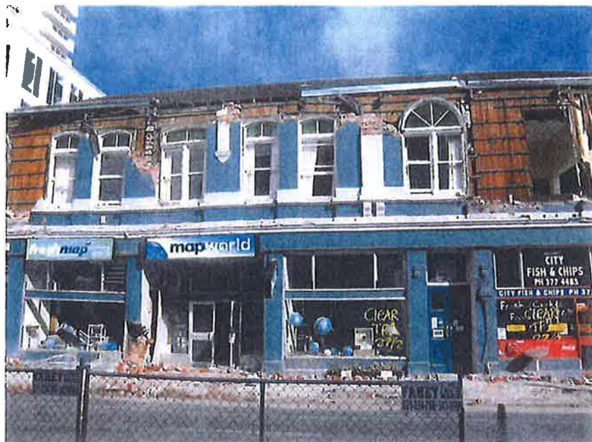
Photograph 1: Manchester Street elevation, showing damage to unreinforced masonry wall and columns and misalignment of the floor.
