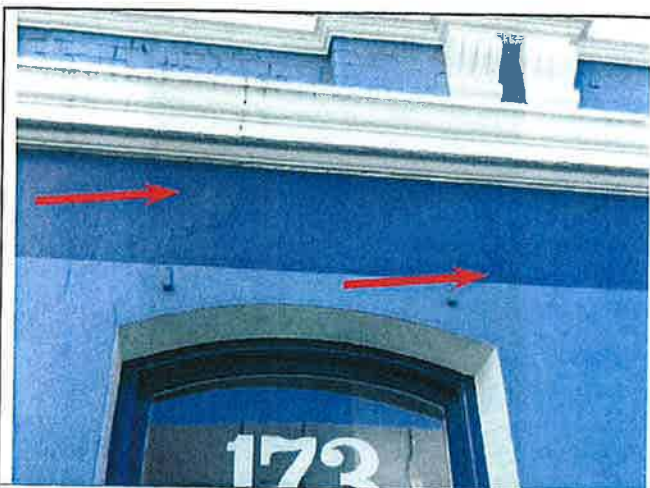
Photo 11. Cracks to Facade
