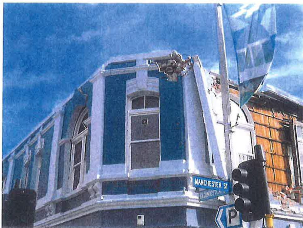
Photograph 3: Corner of the building – detail: Observe less severe damage to unreinforced masonry along the Gloucester Street facade
