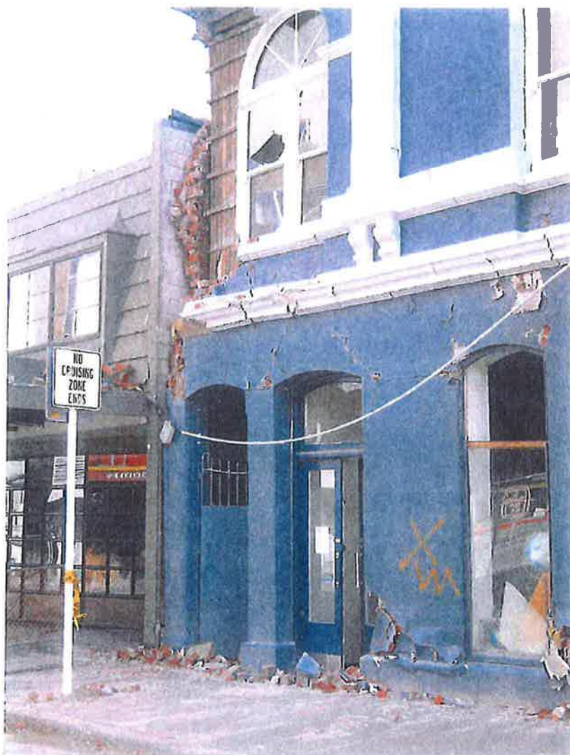
Photograph 5: Gloucester Street Elevation – west end: Damage to the first floor corner – likely due to the pounding with the West neighbour's building.
