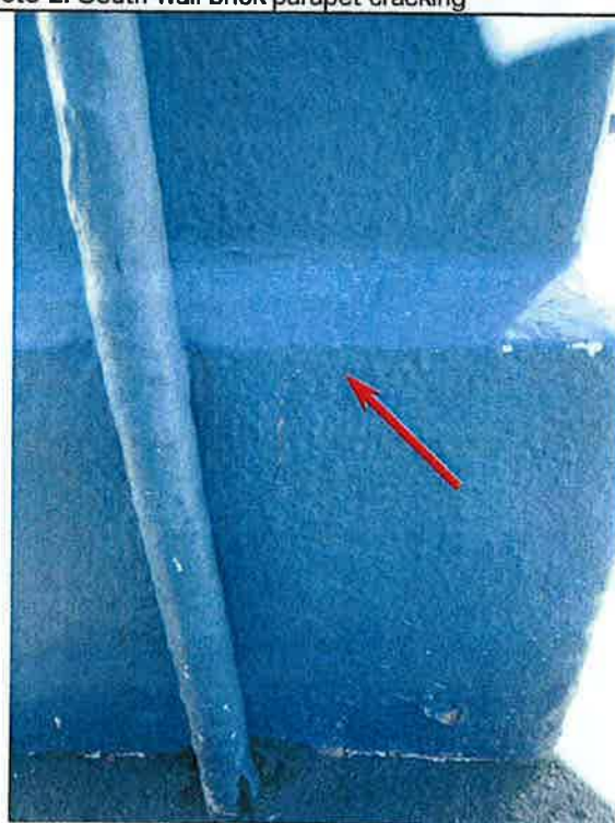
Photo 4. Cracking to foundation
