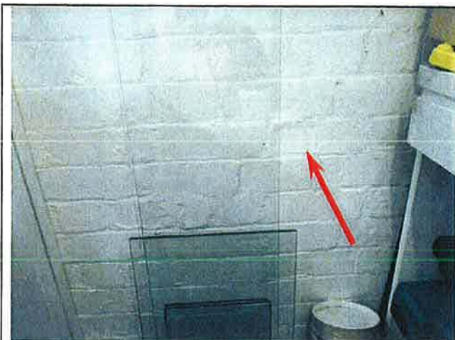
Photo 17. Cracks in internal lining
