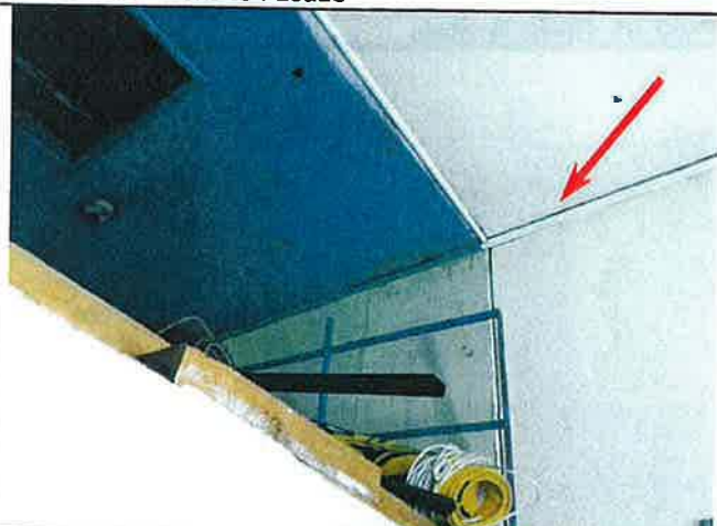
Photo 13. Slight movement to internal linings of 10mm to back wall
