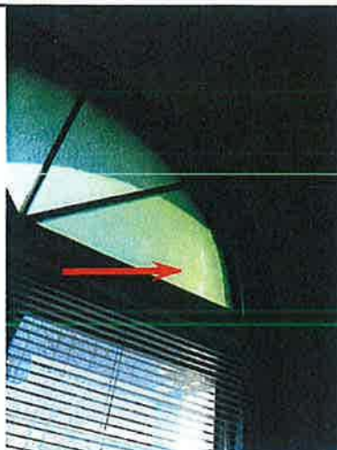
Photo 18. Cracks to glass
