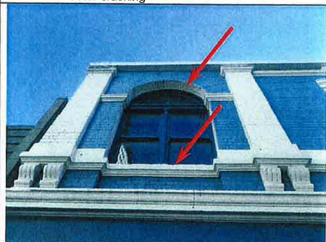
Photo 9. Cracks to Facade
