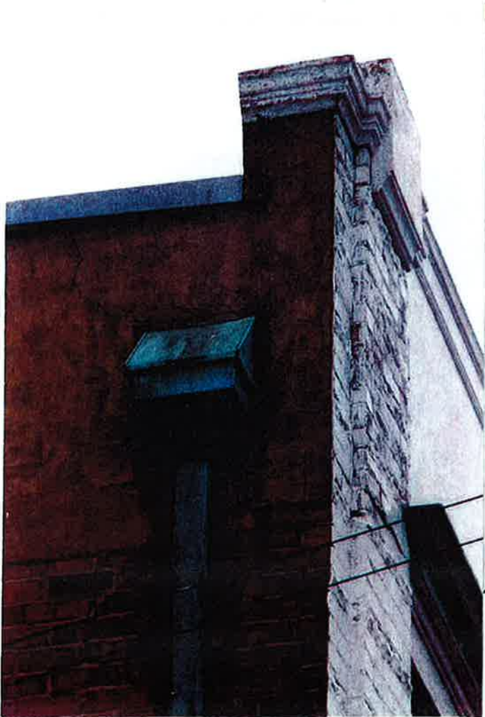
GRACKS DOWN FROM CAP, THROUGH MORTAR TO FRONT ELEVATION
