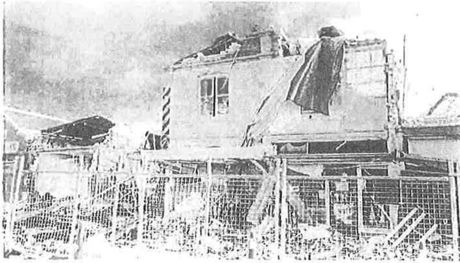
Photo 3 : After the Feb 22, 2011 quake.
