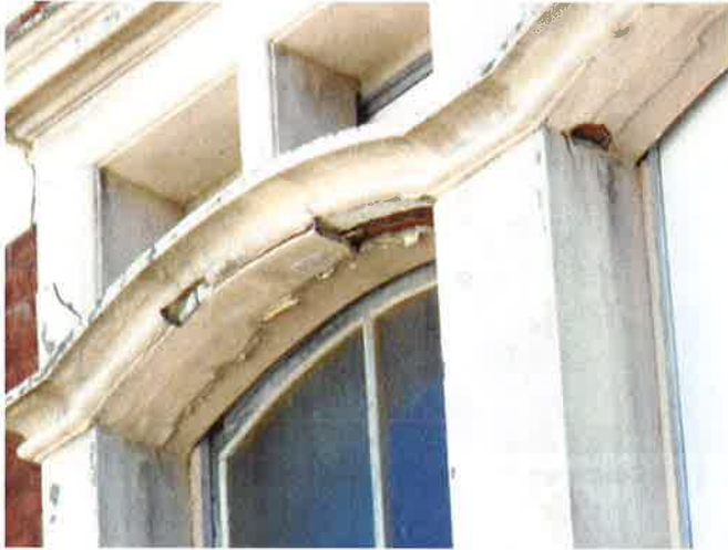
Figure 10 - 603 Window head deterioration, 9th September 2010
