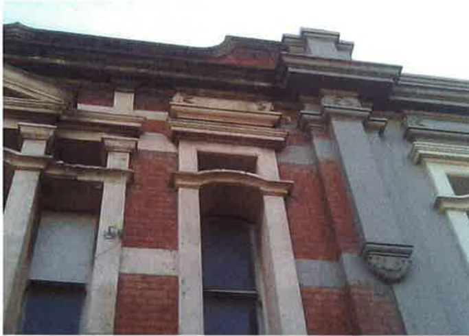
Figure 4 - 1st Floor Junction 603 & 605 Colombo Street, 15 th September 2010
