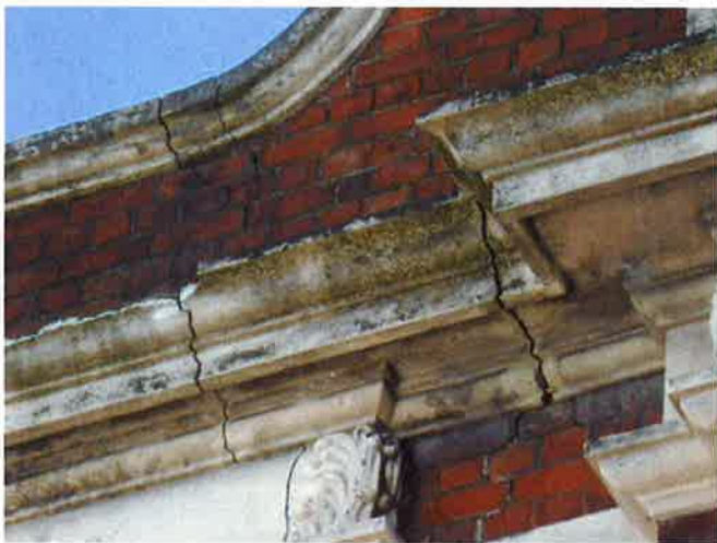
Figure 12 - Cracking generally old, 9th September 2010
