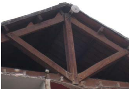
(a) Gable end wall failure despite anchor (see also Figure 13a).
