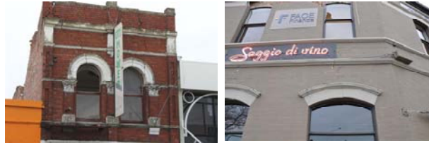
(a) Extensive vertical cracking above window openings
