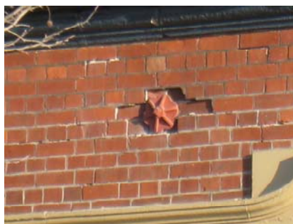
(a) Wall-roof anchorage failure
