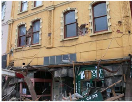
(a) Anchorage failure
