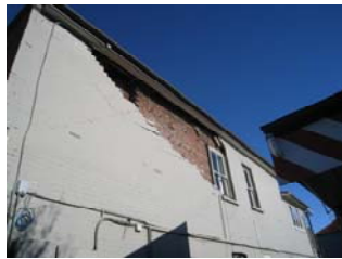
(c) Butterfly wall ties still intact
