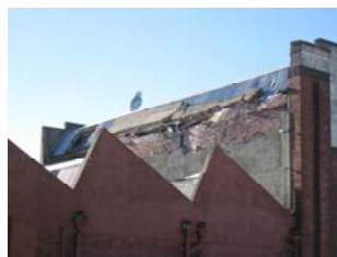
(c) Side wall parapet collapse onto roof.
