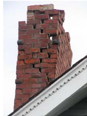
(b) Unstable damaged chimney
