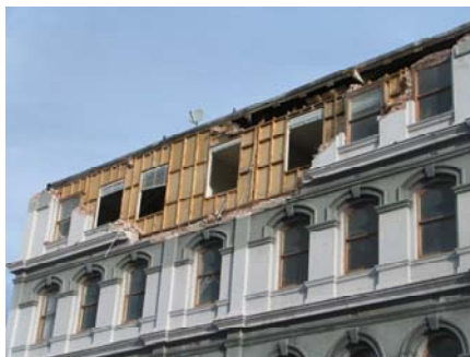
(a) Wall damage at 140 Linchfield Street
