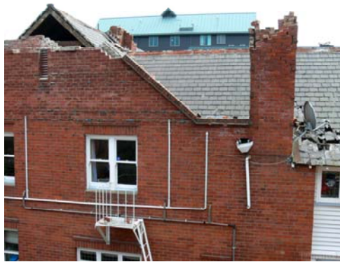
(a) Two damaged chimneys and gable wall
