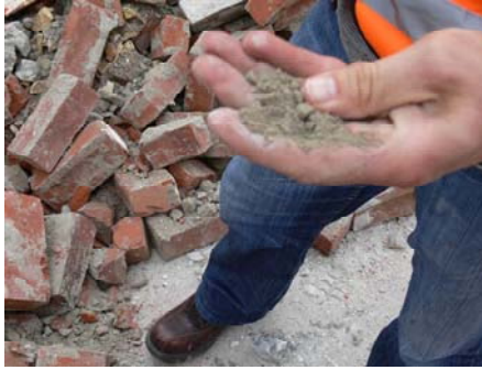
(b) Weak mortar crumbles between fingers
