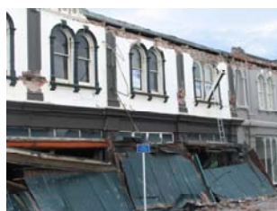
(a) Multiple front wall parapet failures
