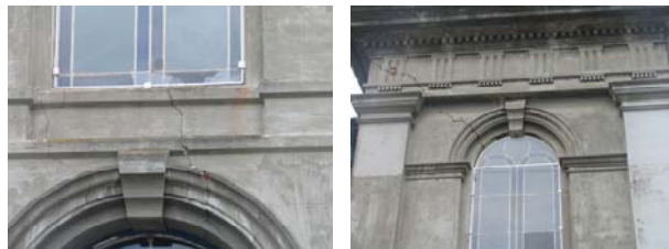
(c) Vertical crack through spandrel
