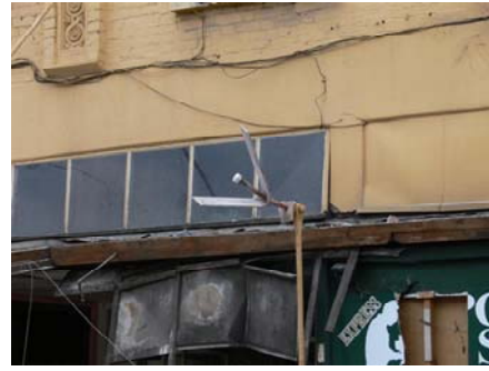
(b) Close-up of failed anchorage detail
