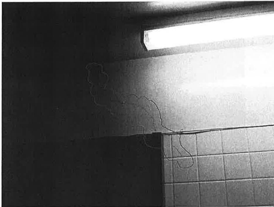
Cracking in un-reinforced unfilled concrete block partition walls to toilets in basement
