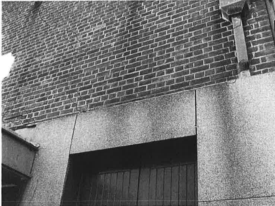
Cracking to brick gable
