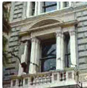
Below: The challenges of heritage conservation where extensive earthquake damage has occurred - Excelsior Hotel, corner Manchester and High Streets and St Lukes Church, Kilmore Street.
