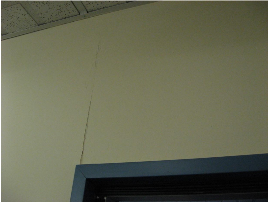
Photo 11 Cracking in linings over door head
