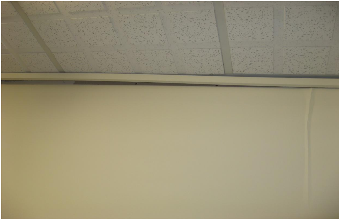
Photo 14 Cracked wall lining and damaged ceiling coving.
