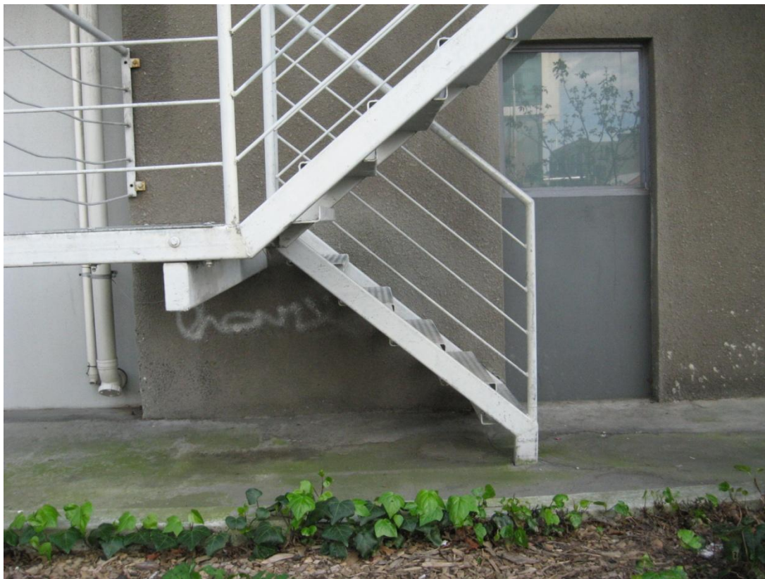
Photo 2 Cracking in south shear wall (not visible in photo) under fire escape landing
