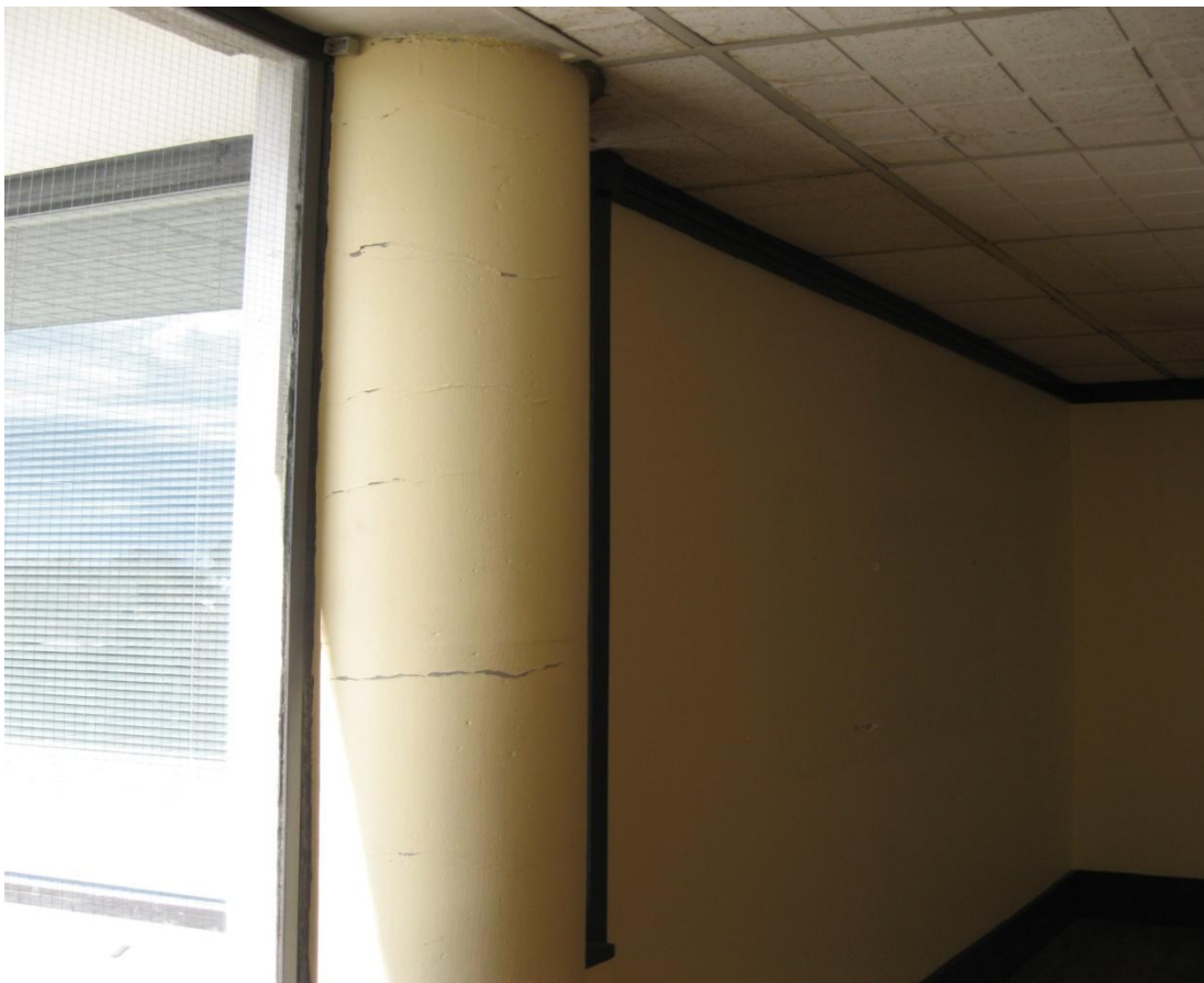
Photo 4 Cracking in top storey column adjacent to lift lobby.
