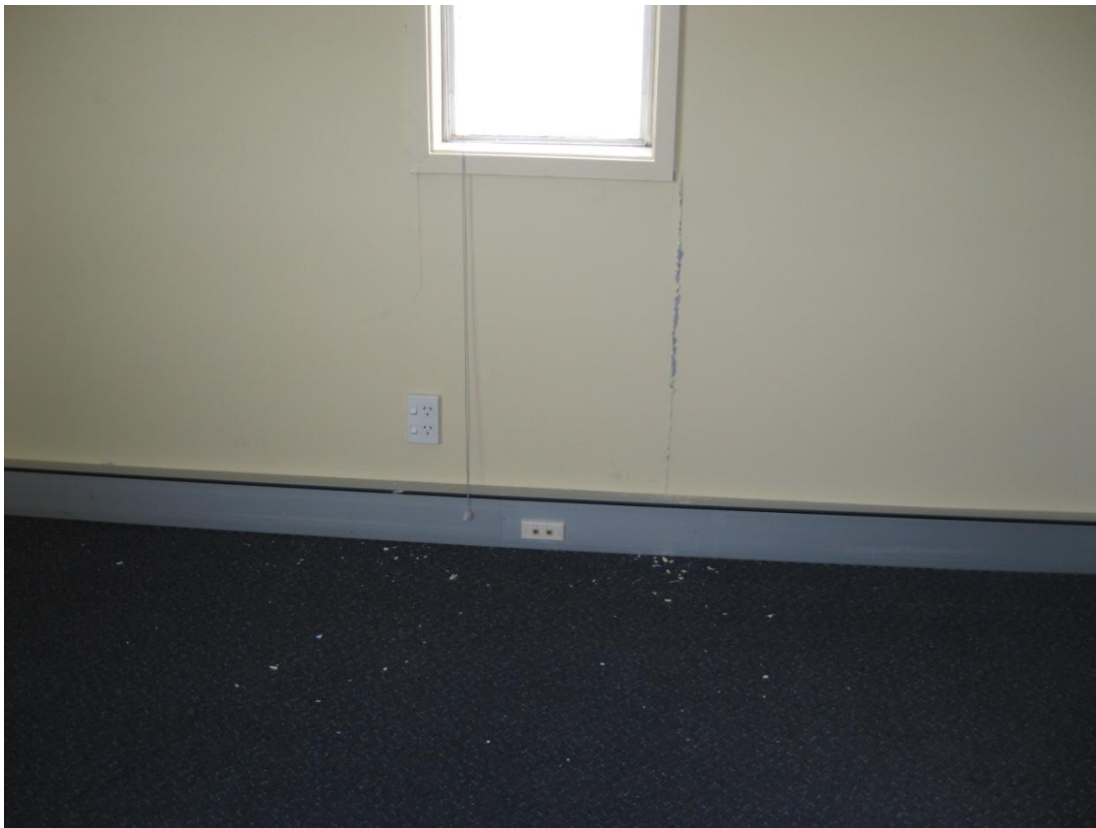
Photo 12 Cracking in linings under window.
