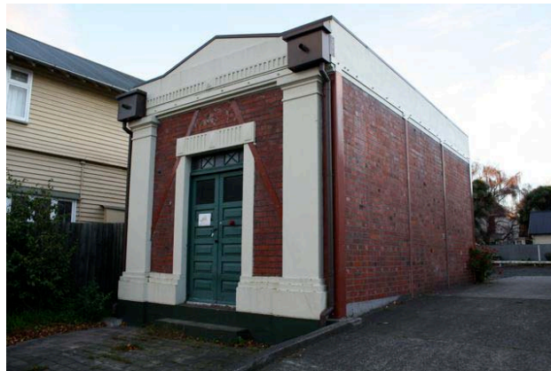
Figure 9: Orion Local Substation. Constructed in unreinforced brick masonry that has been strengthened with a steel perimeter frame (Photo Win Clark)
