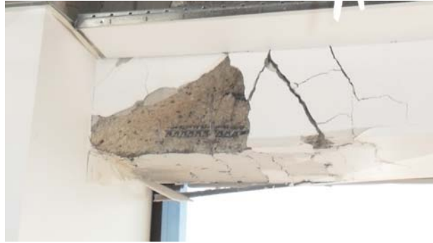
Figure 1: An energy absorbing (ductile) beam hinge in a reinforced concrete building after an earthquake. As these ductile elements yield they absorb energy without loss of strength that would lead to collapse of the building. While some of the cover has fallen off, none of the reinforcing has broken, and the concrete inside the reinforcing cage is intact, so this beam can still carry load.
