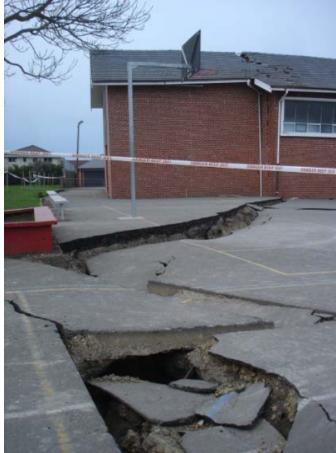
Figure 8 Lateral spread crack running through the courtyard and building at St. Paul's church, Dallington, Christchurch, New Zealand (September 2010) 6
