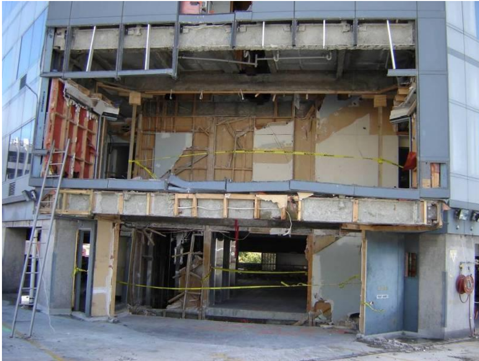
Figure 13 - Access into stairwell from Level 1 and 2 used for removal of stair remnants
