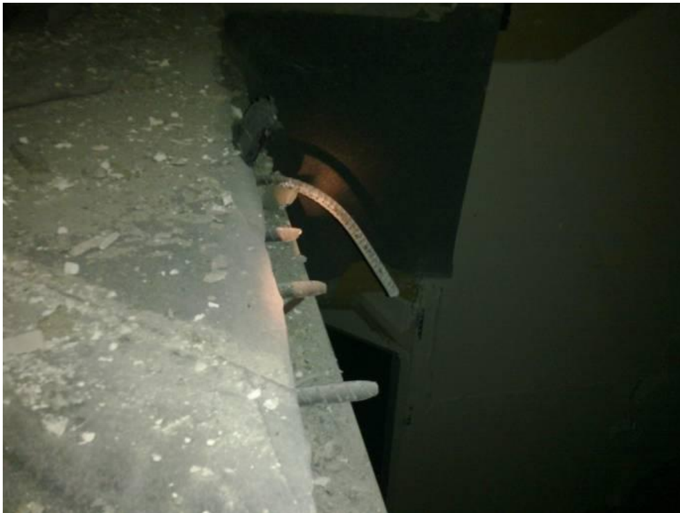
Figure 7 -Level 12 Northeast Exit L12 to L11 stair flight upper support with one de-bonded bar and five fractured D20 bars extending out from the support beam. The 381 x 102 RSC steel channel is undamaged and continues over to the L12 to L13 lower support.
