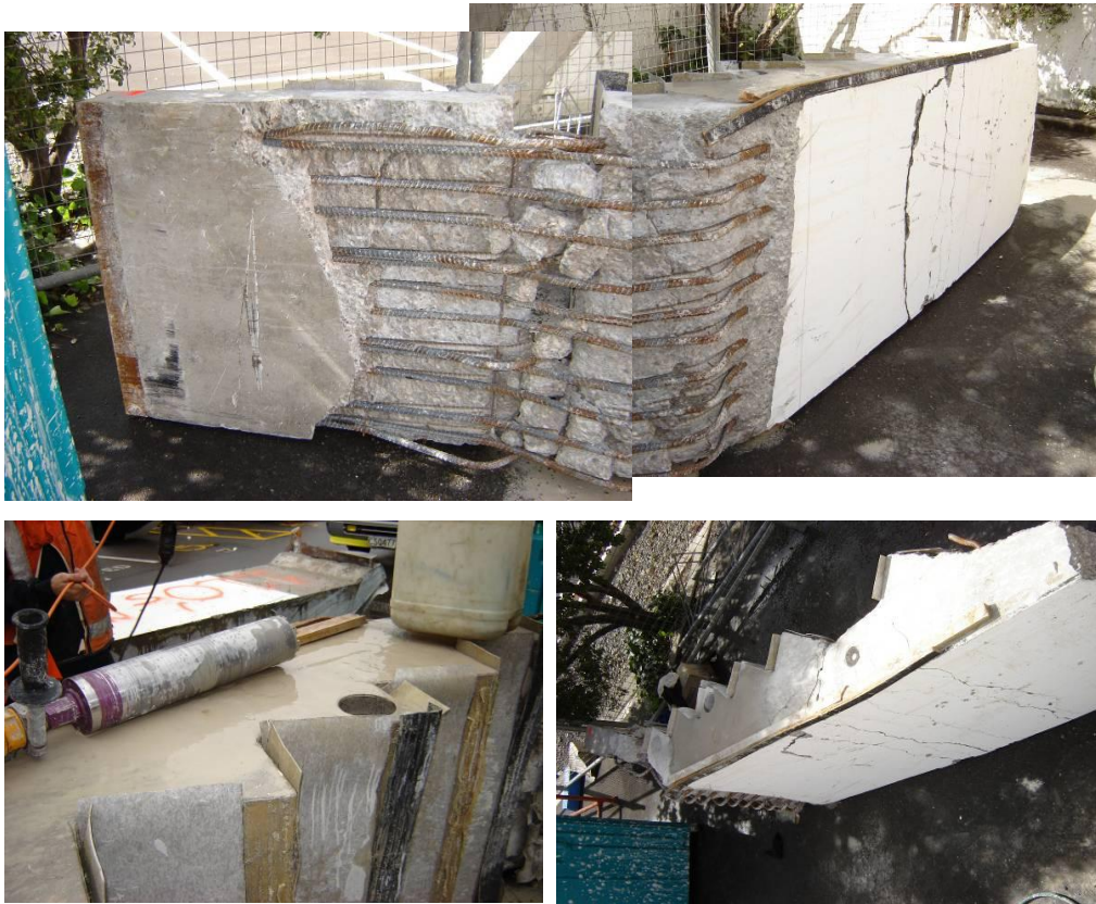
Figure 16 - Unit 1 (clockwise from top): (a) Flexural damage at underside of lower landing; (b) Flexural cracks in underside above lower landing; (c) Concrete core test location in tread.
