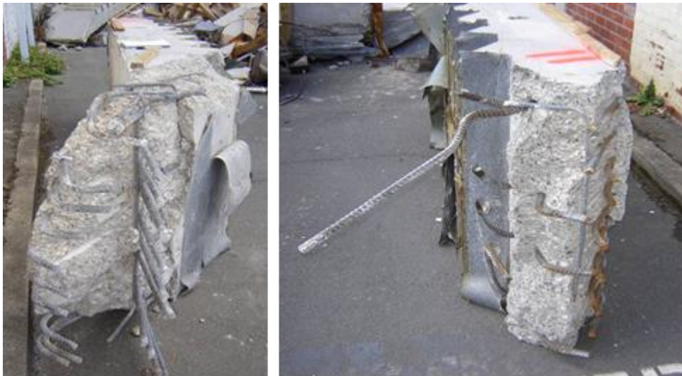
Figure 26 - Unit 11 (left to right): (a) Damaged mid-height landing with hooked bottom bars (bars not gas cut); (b) Bottom rebar gas cut at lower landing junction to first riser.
