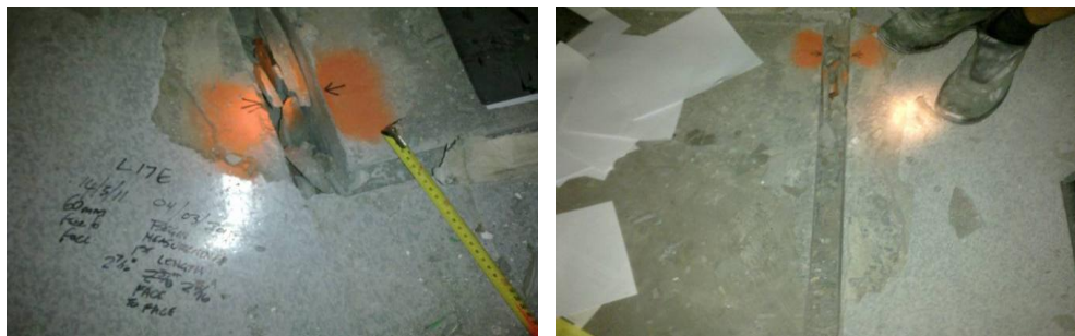
Figure 11 - Level 17 Northeast Exit (left to right) (a) L17 to L18 stair flight seismic gap measurement where a portion of the mortar strip had been removed previously by other parties; L17 to L16 stair flight in foreground. (b) Extent of remaining mortar filling of seismic joint of L17 to L18 stair flight.
