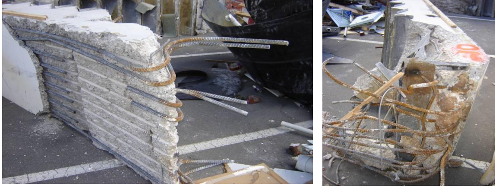
Figure 25 - Unit 10 (left to right): (a) Underside near mid-height landing where D20 reinforcing steel samples were extracted for testing; (b) Damaged lower landing.
