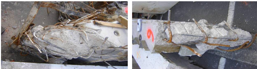
Figure 24 - Unit 9 (Left to right): (a) Damaged upper landing; (b) Damaged mid-height landing with crushed concrete and de-bonded reinforcing.
