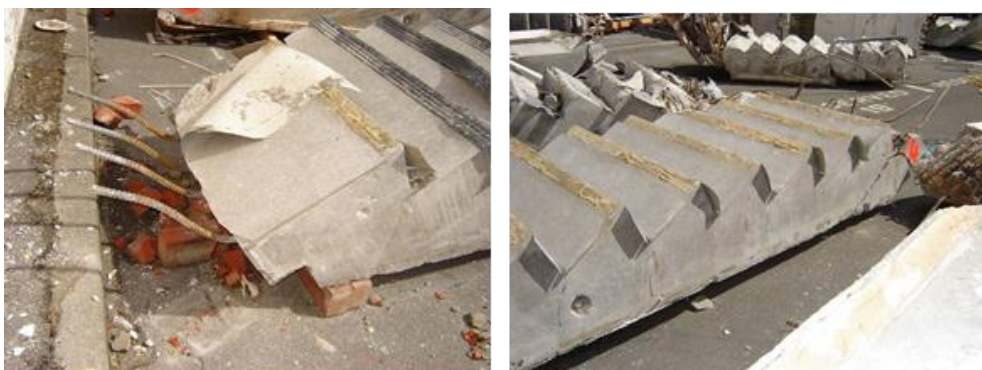
Figure 19 - Unit 4 (left to right): (a) De-bonded top landing bars (possibly from Level 2); (b) Cracks across stair throat at toes of risers.
