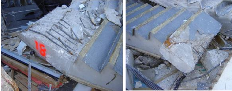
Figure 33 - Unit 18 (Left to right): (a) Gas cut bars at mid-height landing. No construction joint apparent in side face indicating stair was precast as one unit; (b) Cut support bars at upper landing.
