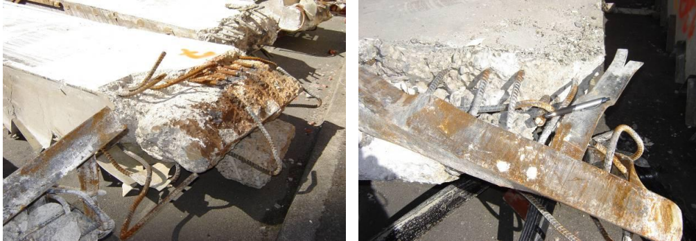
Figure 22 - Unit 7 (left to right): (a) Gas cut mid-height landing bars. Cracks across throat at toe of risers; (b) Damaged upper landing steel seating angle.
