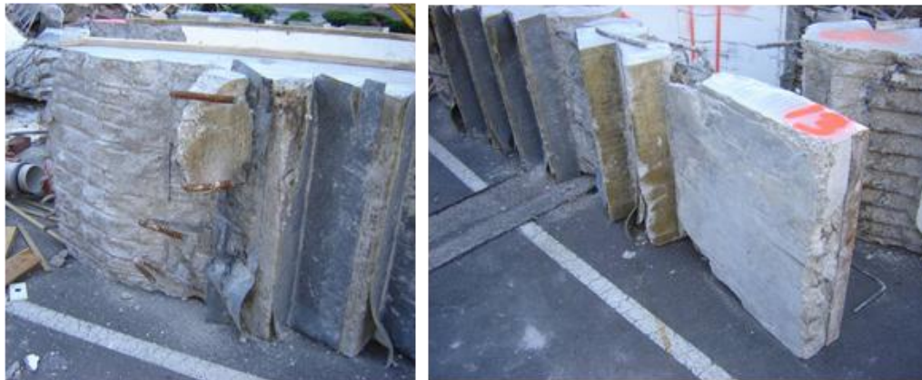
Figure 28 - Unit 13 (left to right): (a) Mid-height landing; (b) Lower landing 600-700 mm long with flexural damage at first riser
