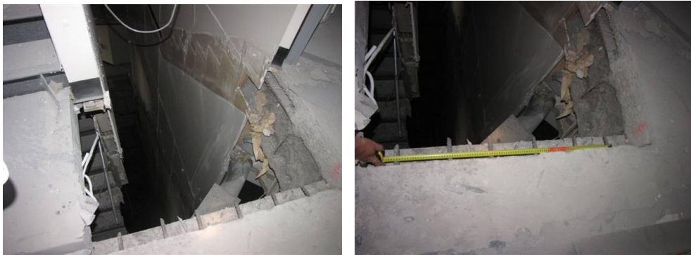
Figure 10 - Level 15 Southwest Exit: (photos from left): (a) Remaining Level 15 Southwest Exit L15 to L16 stair flight lower landing with the remaining Level 14 Southwest Exit L14 to L15 Stair Flight able to be seen directly below. All flights below and including the Level 15 Southwest Exit Level 15 to 14 stair flight have fallen away; (b) Fractured reinforcing remnants at upper support of the Level 15 Southwest Exit L15 to L14 flight which has fallen away.
