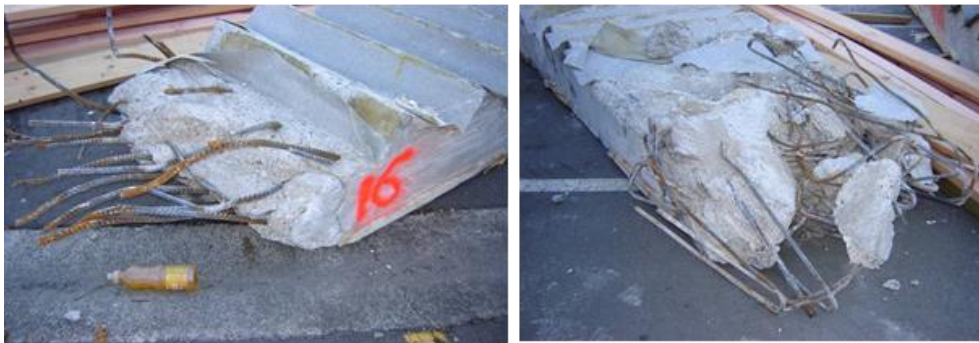
Figure 31 - Unit 16 (left to right): (a) Mid-height landing bars gas cut; (b) Damaged upper landing.
