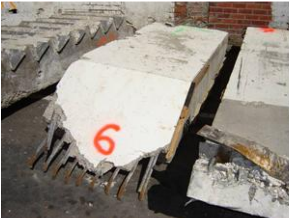
Figure 21 - Unit 6 broken up and gas cut landing. 30 to 50 mm cover to ten D20 reinforcing at underside of lower landing. The Unit 7 upper landing is at the right.
