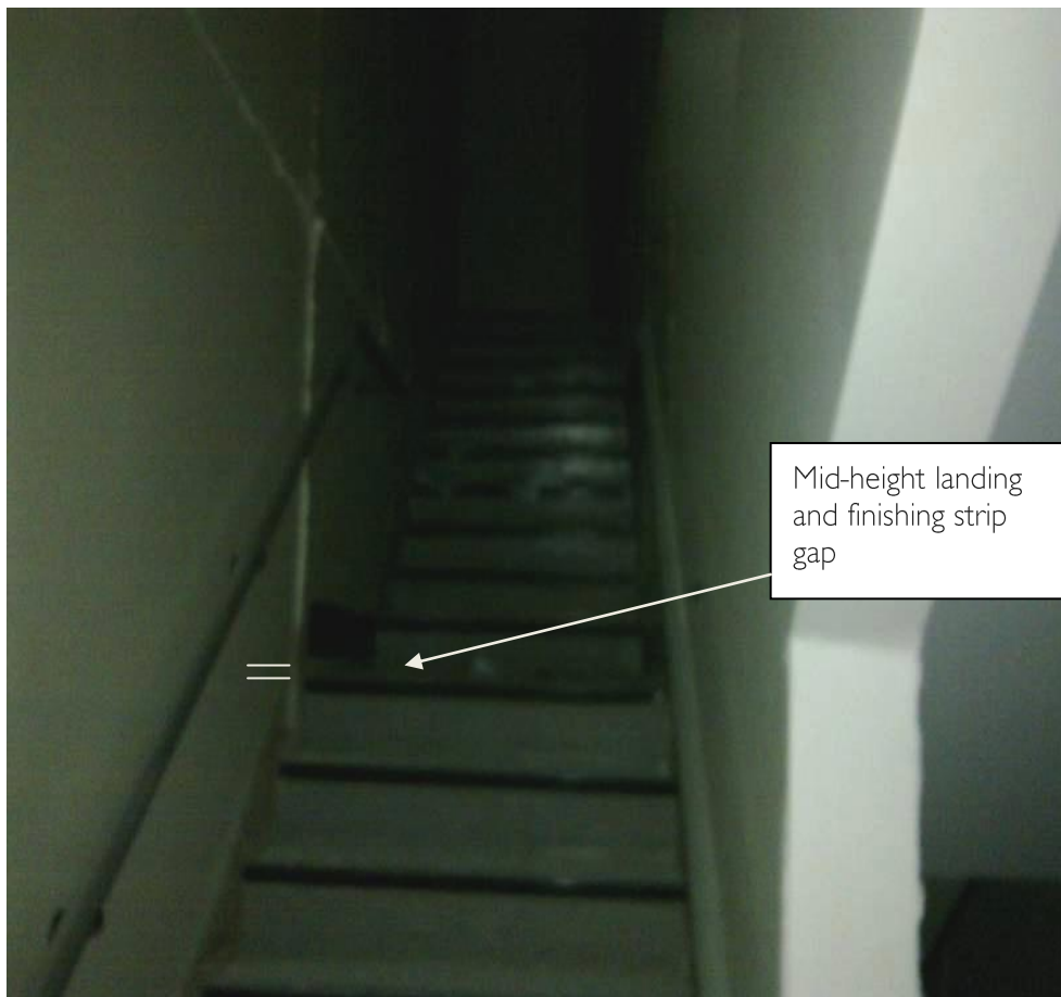
Figure 9 - Level 15 Northeast Exit L15 to L16 Stair Flight showing vertical displacement at mid-height landing relative to black finishing strip.
