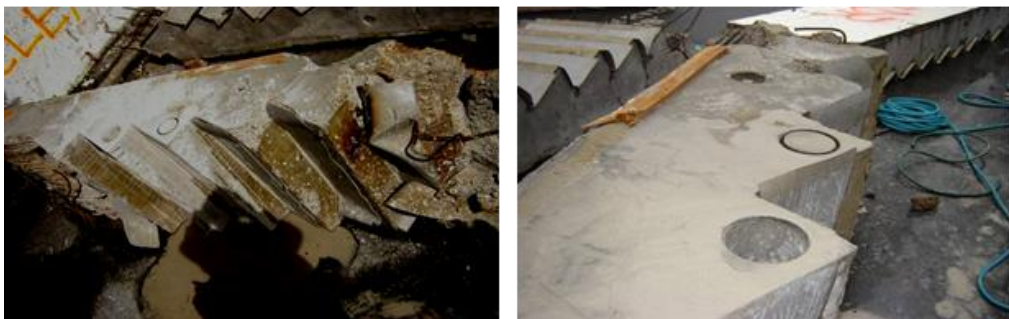
Figure 17 - Unit 2 showing concrete core test locations on the sides of treads
