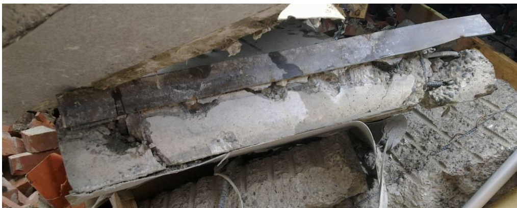
Figure 15 - Upper landing reinforcing steel fractures matching those seen in the stairwell supports. The steel seating angle to the underside and end of the stair flight landing is visible at the top
