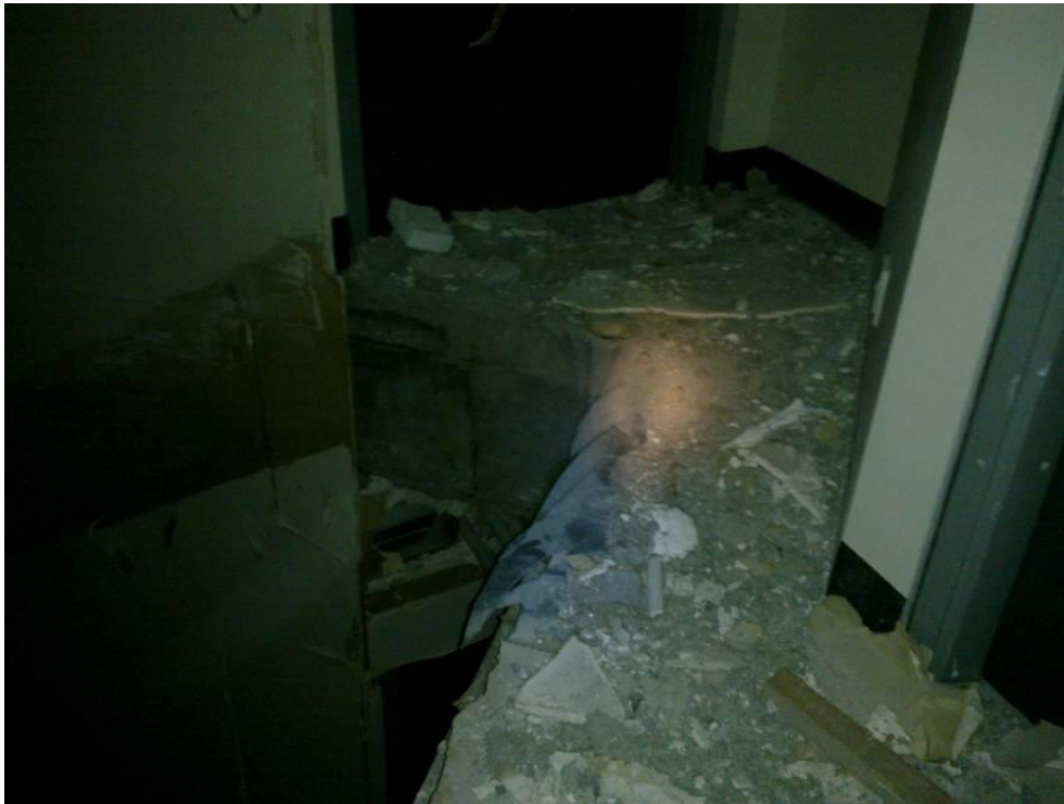
Figure 6 - Level 9 Southwest Exit L9 to L8 Stair Flight upper support with fractured D20 reinforcing and lino that appears to have been torn by stairs falling from above
