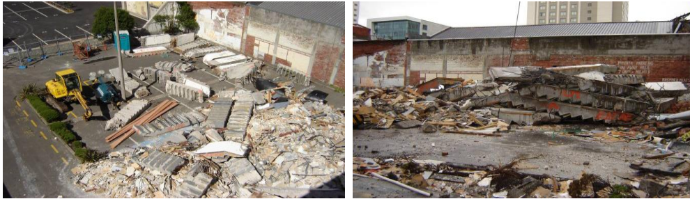
Figure 12 - Stair remnant debris in car park behind Forsyth Barr building after their removal from the stairwell.
