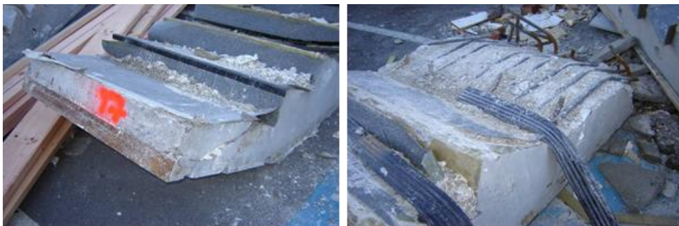
Figure 32 - Unit 17 (Left to right): (a) Lower landing with compression support lateral impact shear cracking and saw cut end; (b) Mid-height landing ten D20 bottom bars bent and developed to underside of second riser below landing exposed, four D20 top bar stubs visible.
