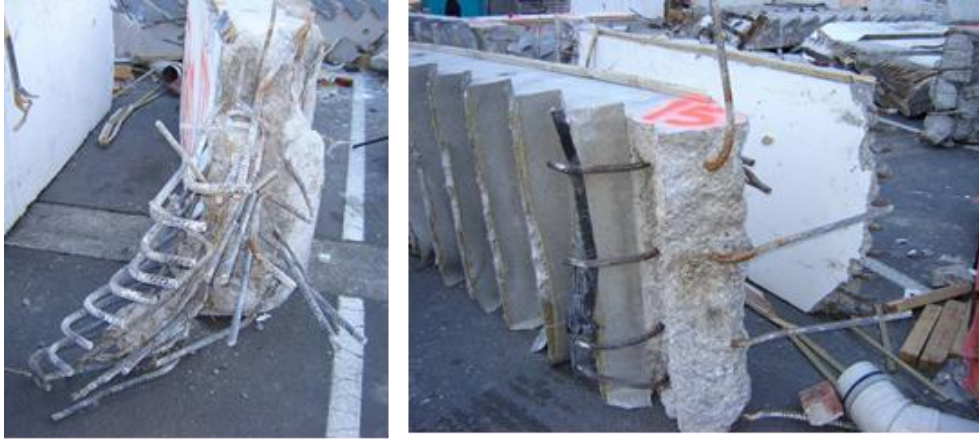
Figure 30 - Unit 15 (Left to right): (a) Damaged mid-height landing with hooked bottom bars; (b) Gas cut bars at lower landing which has broken away near first riser.
