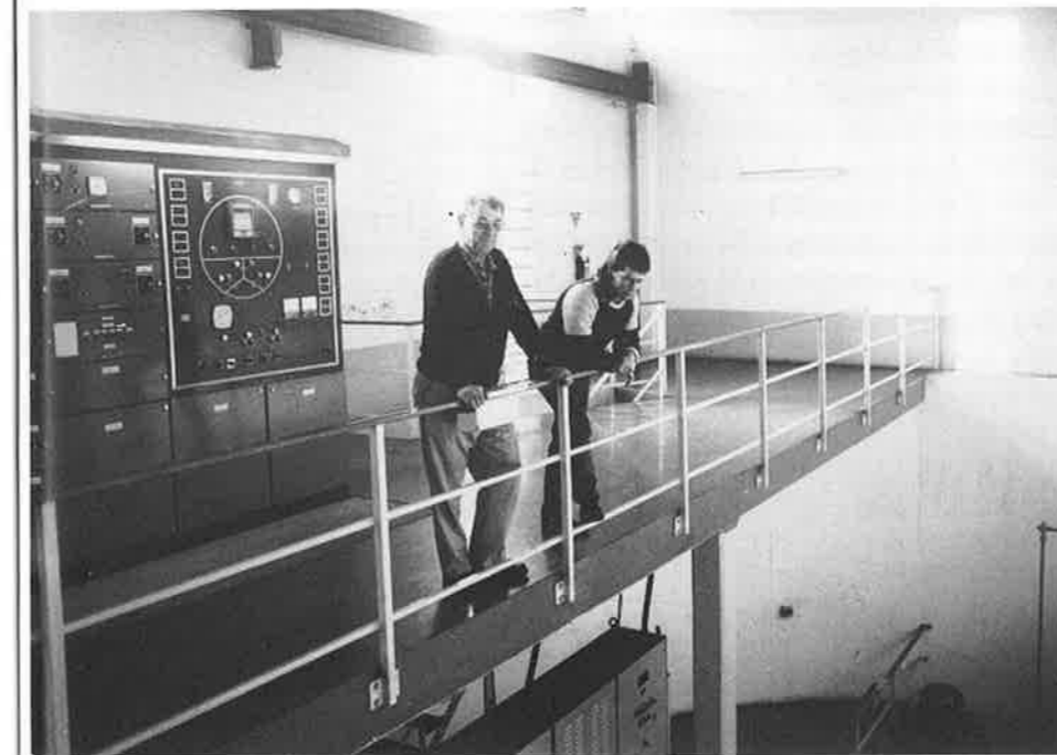
Above left: Two Drainage Board employees inside the Number 15 Pumping Station.
