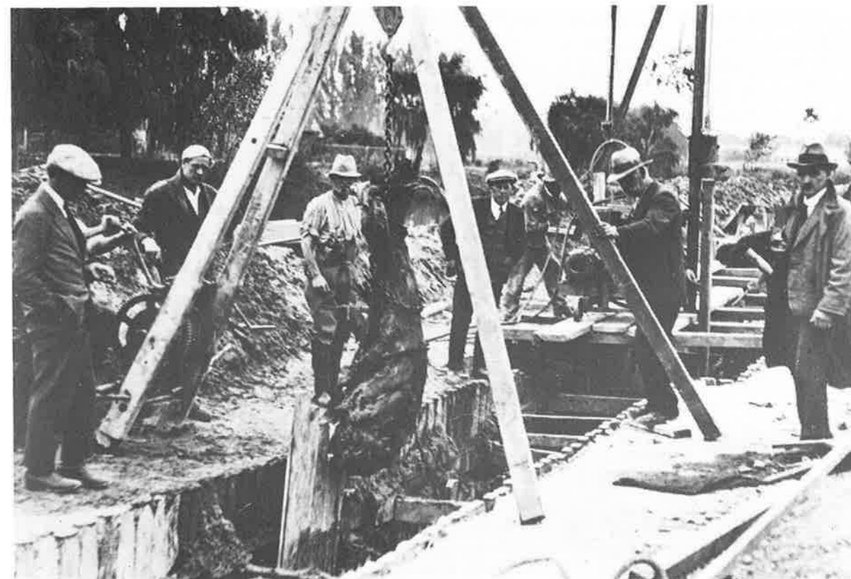
Below: Construction, by contractors, of the Number 8 sewer along Retreat Road in the 1920s. Drainage Board
