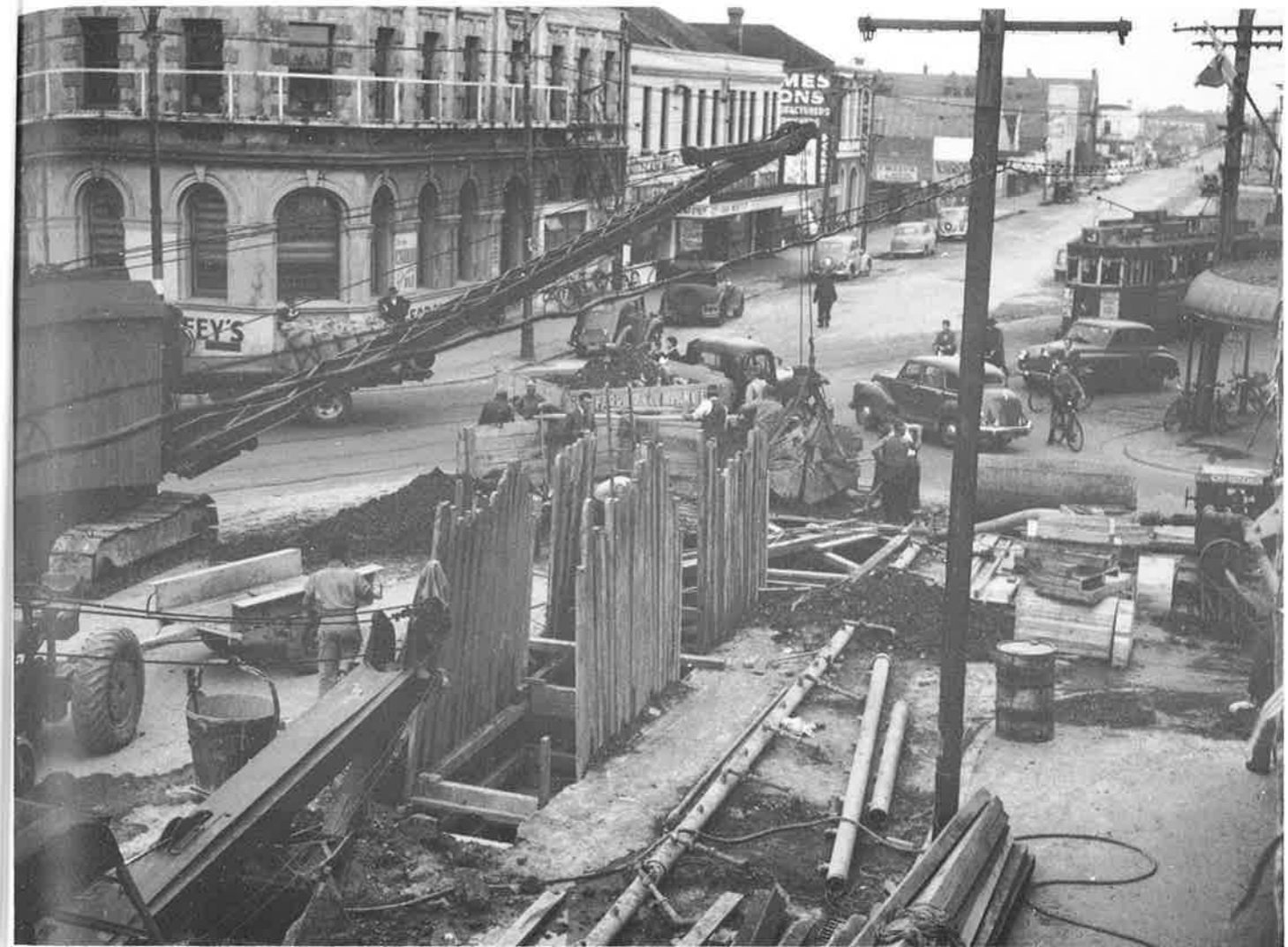
Construction work on the southern relief sewer, 1950, at the corner of Madras and St Asaph Streets. Drainage Board
