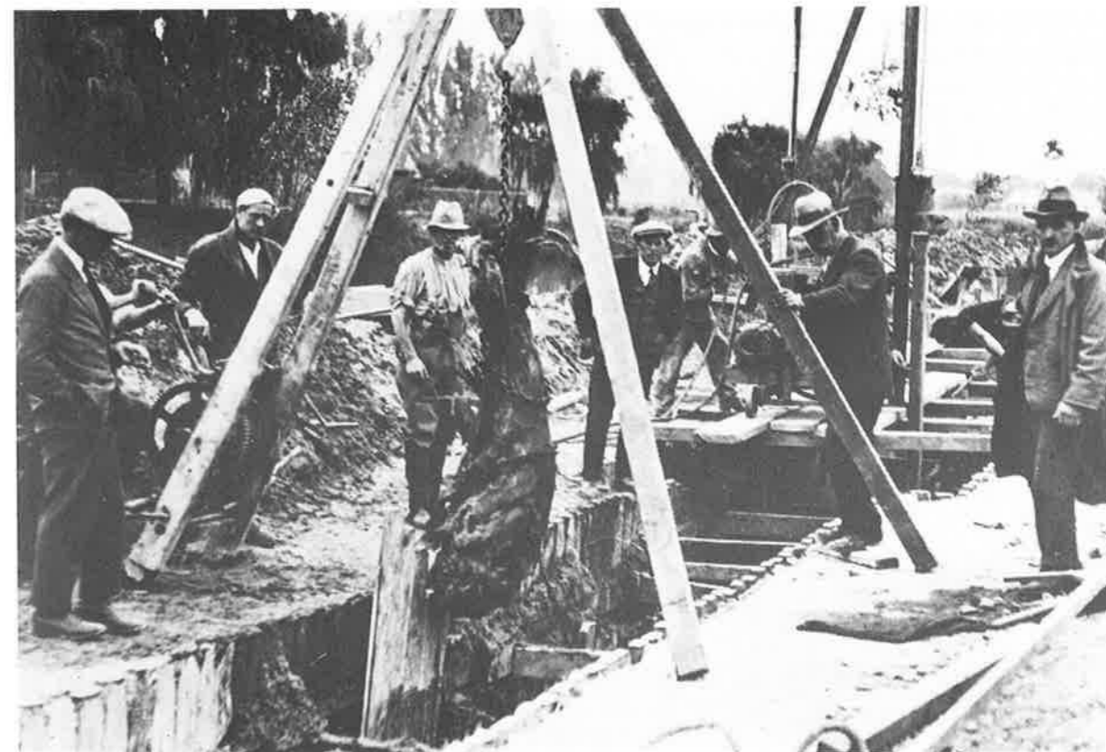
Below: Construction, by contractors, of the Number 8 sewer along Retreat Road in the 1920s. Drainage Board
