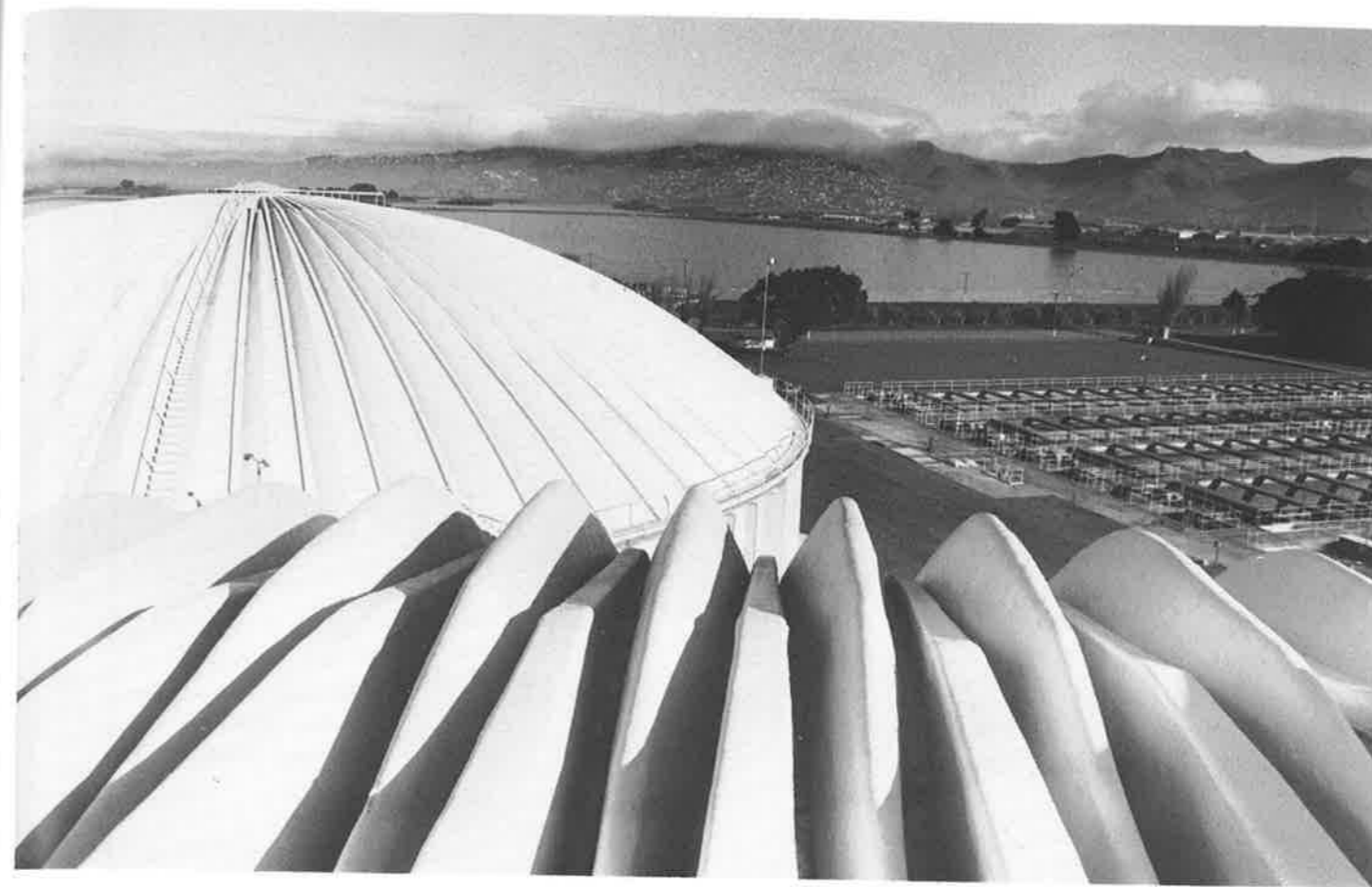
Looking from the top of one of the covered trickling filters across to the oxidation ponds. The second covered trickling filter is to the left. The ribs in the foreground are at the top of the fibreglass cover of the filter. Ash Spice
