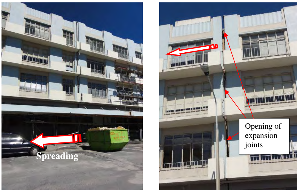
Figure 20. Stretching of foundations due to lateral spreading resulting in opening of the expansion joints
