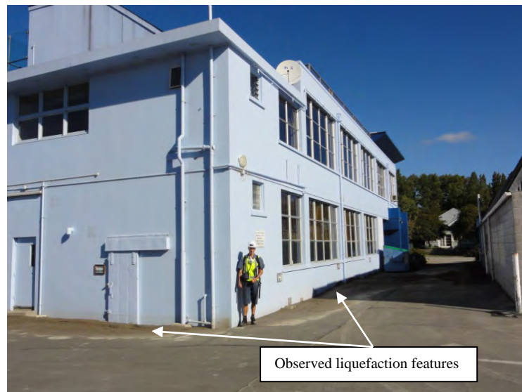
Figure 17. Punching settlement of a building in liquefied soils
