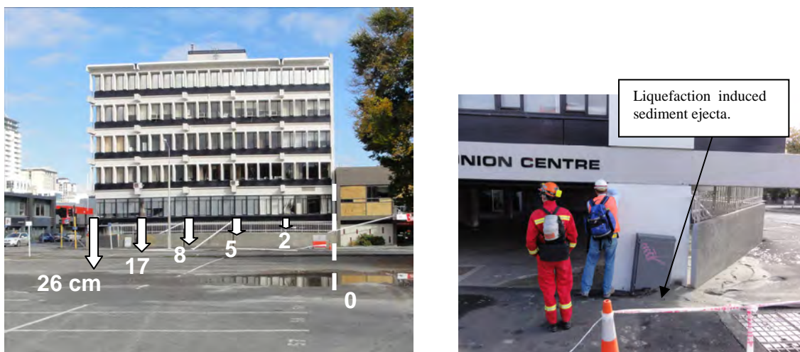
Figure 16. Liquefaction-induced differential settlement of a six storey building
