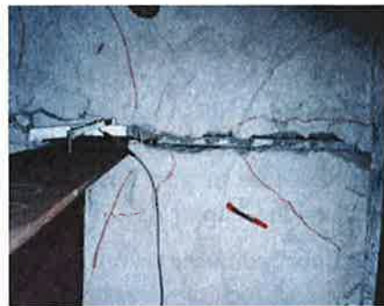
Figure 6.8. Slab damage in a post-tensioned steel beam subassembly (Clifton, 2005).
