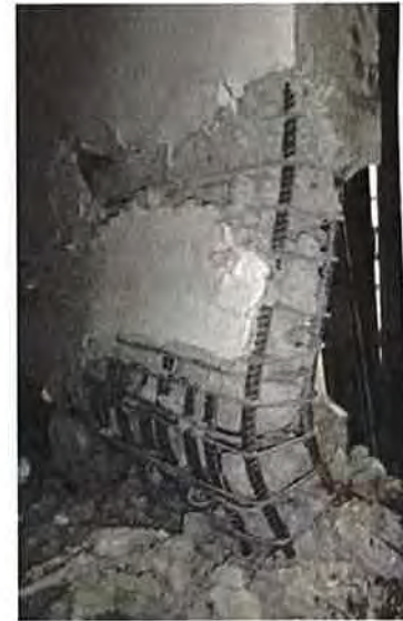
(b) Severe damage to reinforced concrete wall, with local buckling at the toe of the wall.
