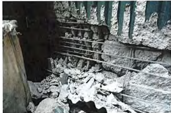
(b) Severely damaged end of structural wall.
