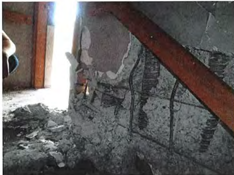
(a) The system for joining precast concrete wall panels fails through insufficient confining reinforcement.
