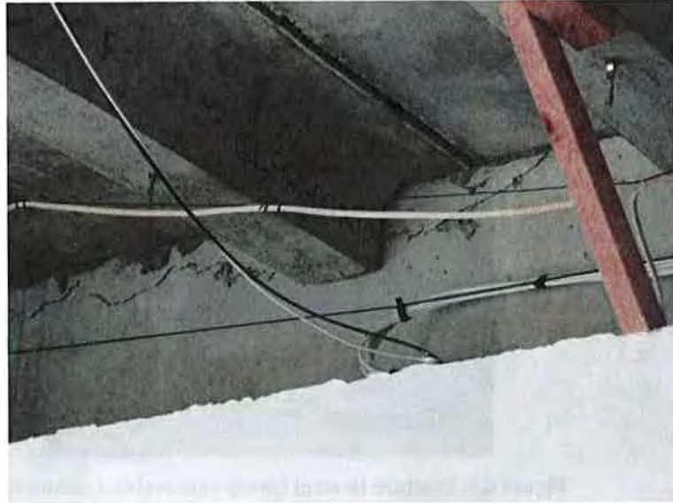
Figure 4.6. Spalling of concrete ledge supporting the flange-hung Tee units.
