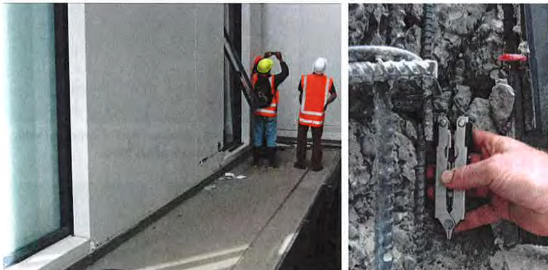
(a) Small crack in base of a tall wall. Note the minor damage at far end of wall.
