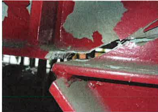
Figure 4.7. Fracture in steel frame near welded connection.
