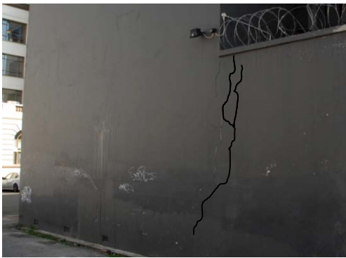
(c) Highlighted crack location at the rear of building
