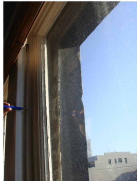
(b) facade wall pulled away from the side walls
