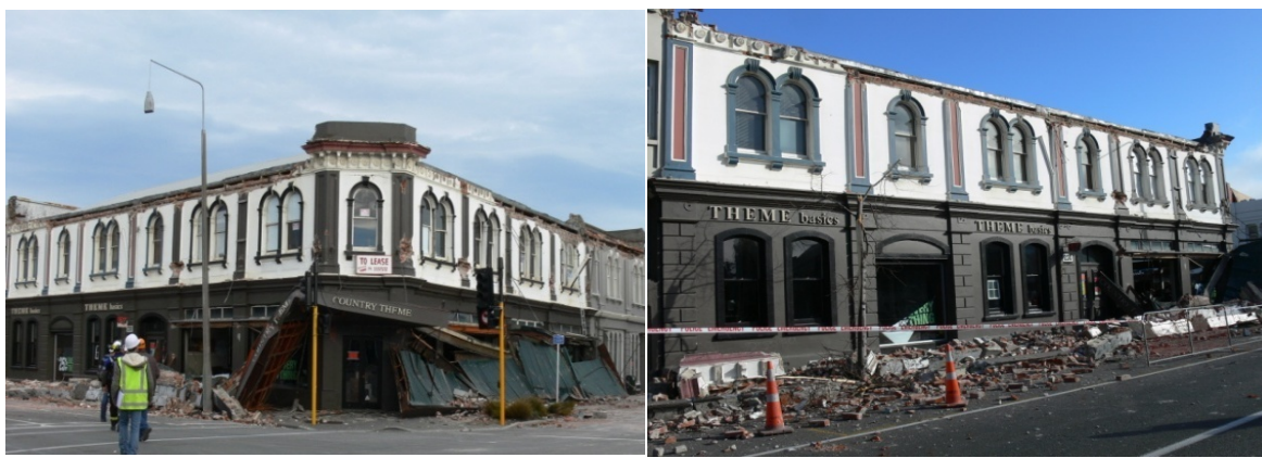
(a) Corner view showing parapet collapse
