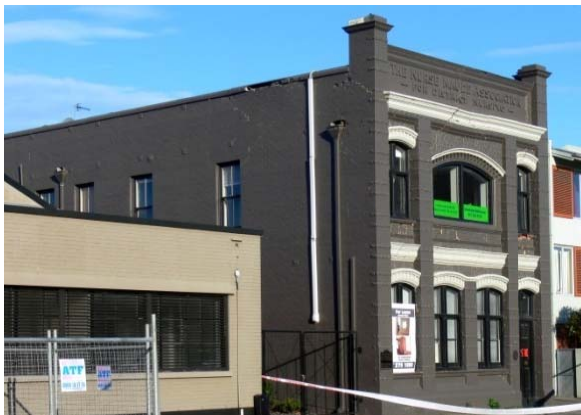
(a) cracking through top spandrel
