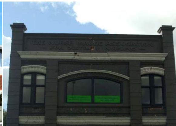
(b) in-plane diagonal cracking through top spandrel
