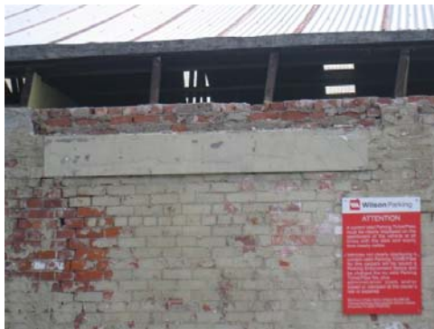
(b) Side-view of tilted joists
