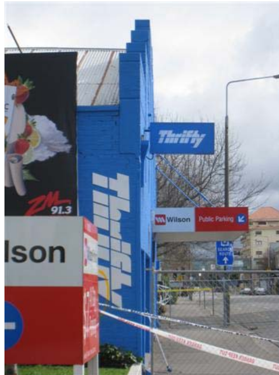
(c) Front wall curvature
