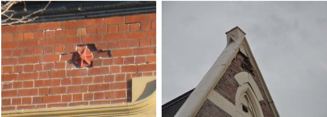
(a) Wall-roof anchorage failure
