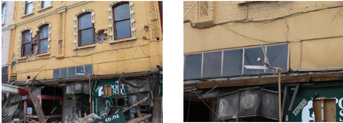
(a) Anchorage failure
