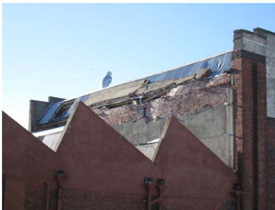
(c) Side wall parapet collapse onto roof.
