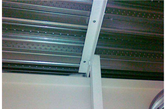
Missing floor anchors at L2 east wall at top of ramp
