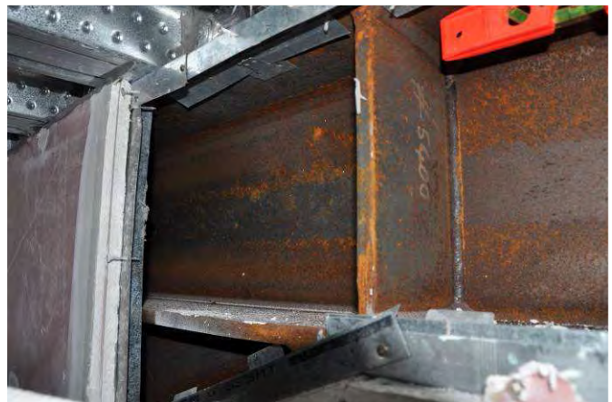
L6, Grid C4(west), brace connection
