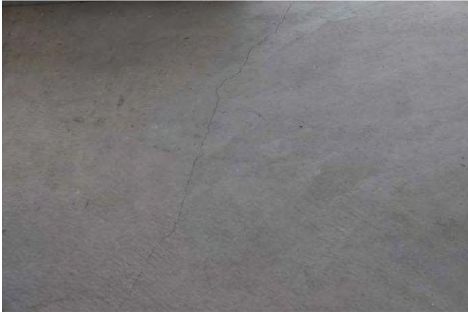
L22 crack to floor diaphragm (from stairwell to NE)
