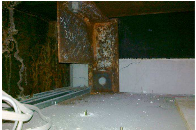
L11, Grid C2, damaged panel fixing
