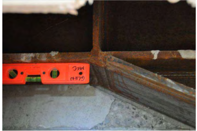
L7, Grid F5, active link and brace connection
