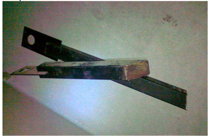
Fractured carstacker top lateral restraints
