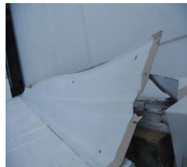
6th Floor Deck Flashing Cover Broken
