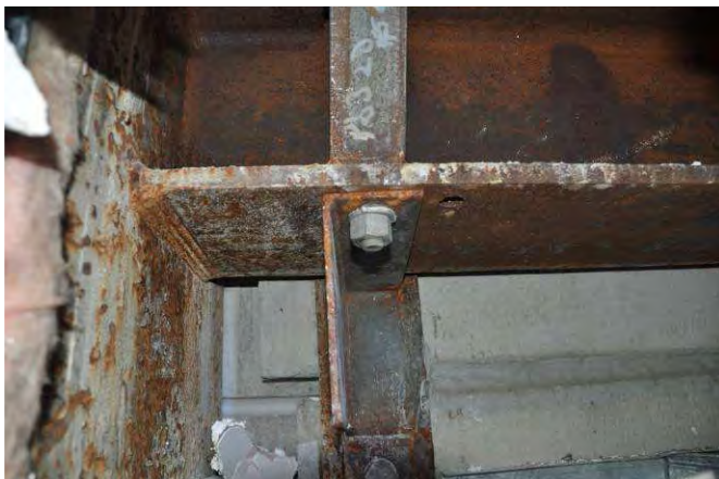
L6, Grid C2, column weld
