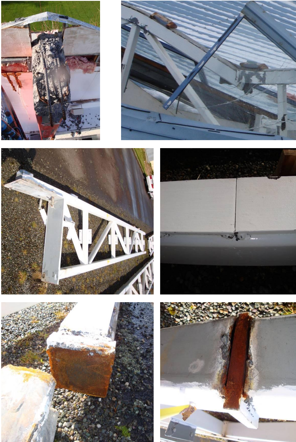
Figure 24 - Truss T2 (Clockwise from top left) (a) Sheared head of column C12; (b) Mid span failure of top chord; (c) End butting of side plates without the specified complete penetration butt weld; (d) Typical top chord fit up at packer plates with 3-sided bearing at quarter point splice; (e) Top chord packer plate at mid span showing no evidence of the specified complete penetration butt weld; (f) Truss T2 in salvage yard with TCM still attached to column C12 end plate.
