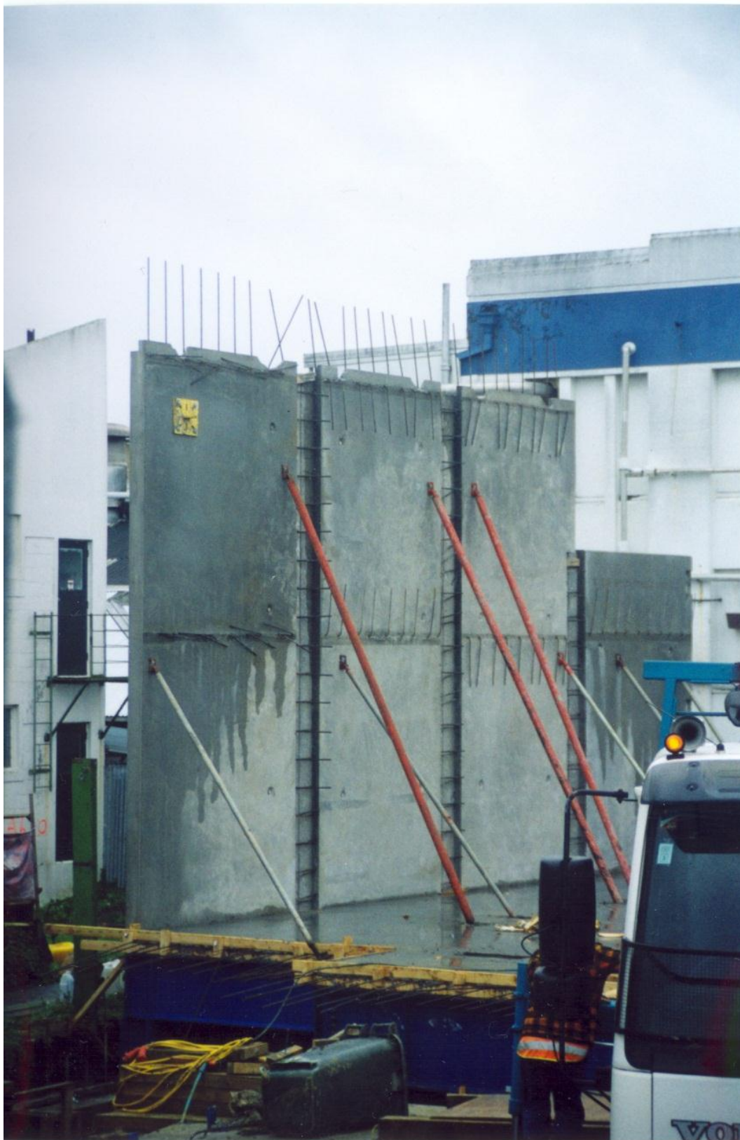
Illegal Construction – Auckland – 2004
