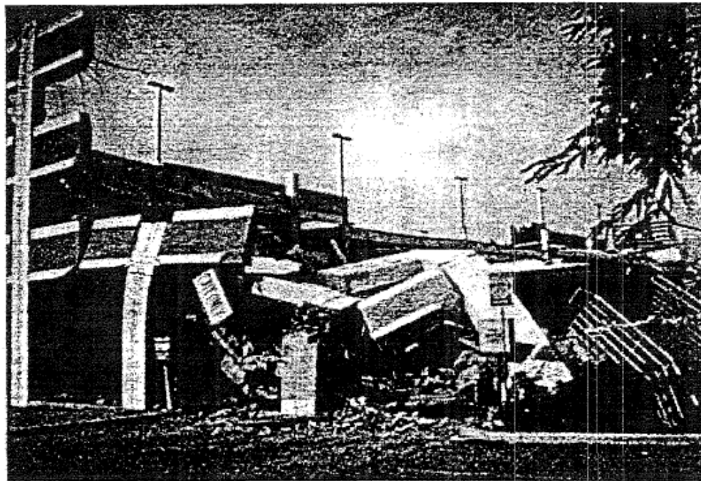
Fig. 1. Collapsed parking structure of the California State University Northridge [Papazoglou and Elnashai, 1996].
