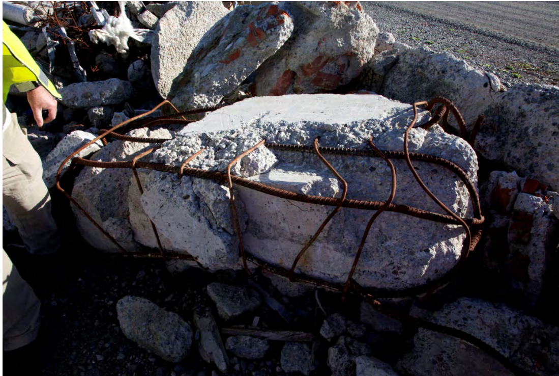
(a) Overview of edge beam showing shell beam broken away from the infill concrete
