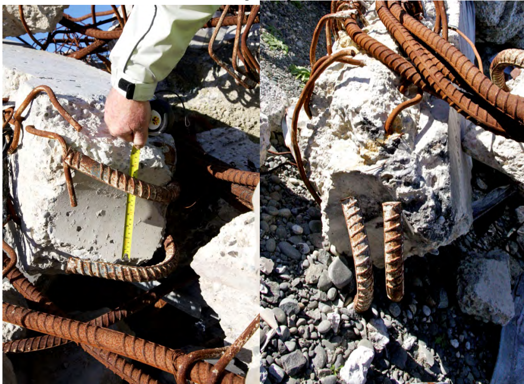
(b) Examples of internal beams with broken "wings"
