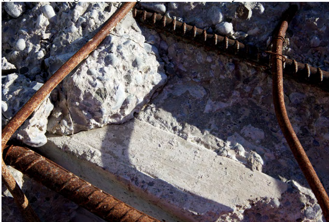
(b) Close-up of smooth and rough surfaces of infill concrete. The concrete of the shell beam had been broken to reveal the shell beam reinforcement.
