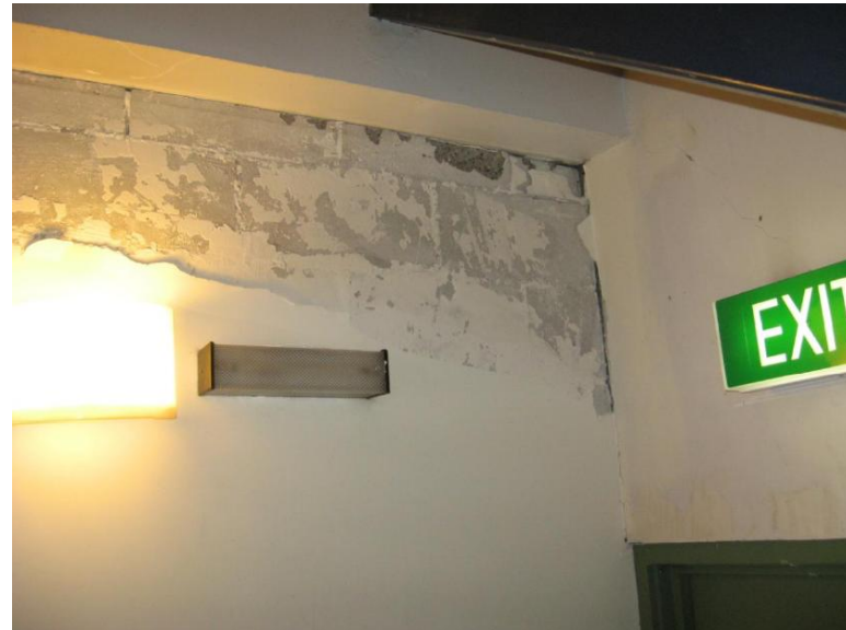
Spalling plaster at masonry wall
