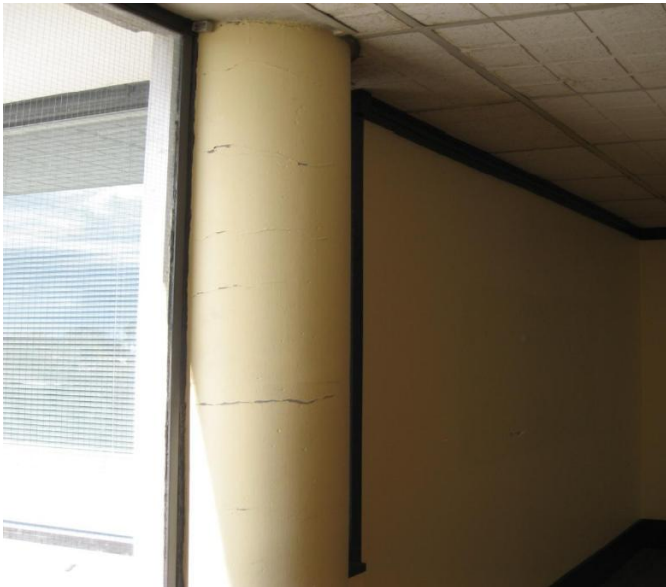
Column cracking Level 6
