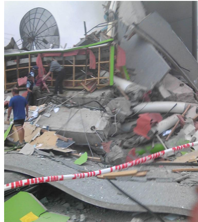
View from east at Line 4 North Core immediately after the collapse at 1:00 pm
