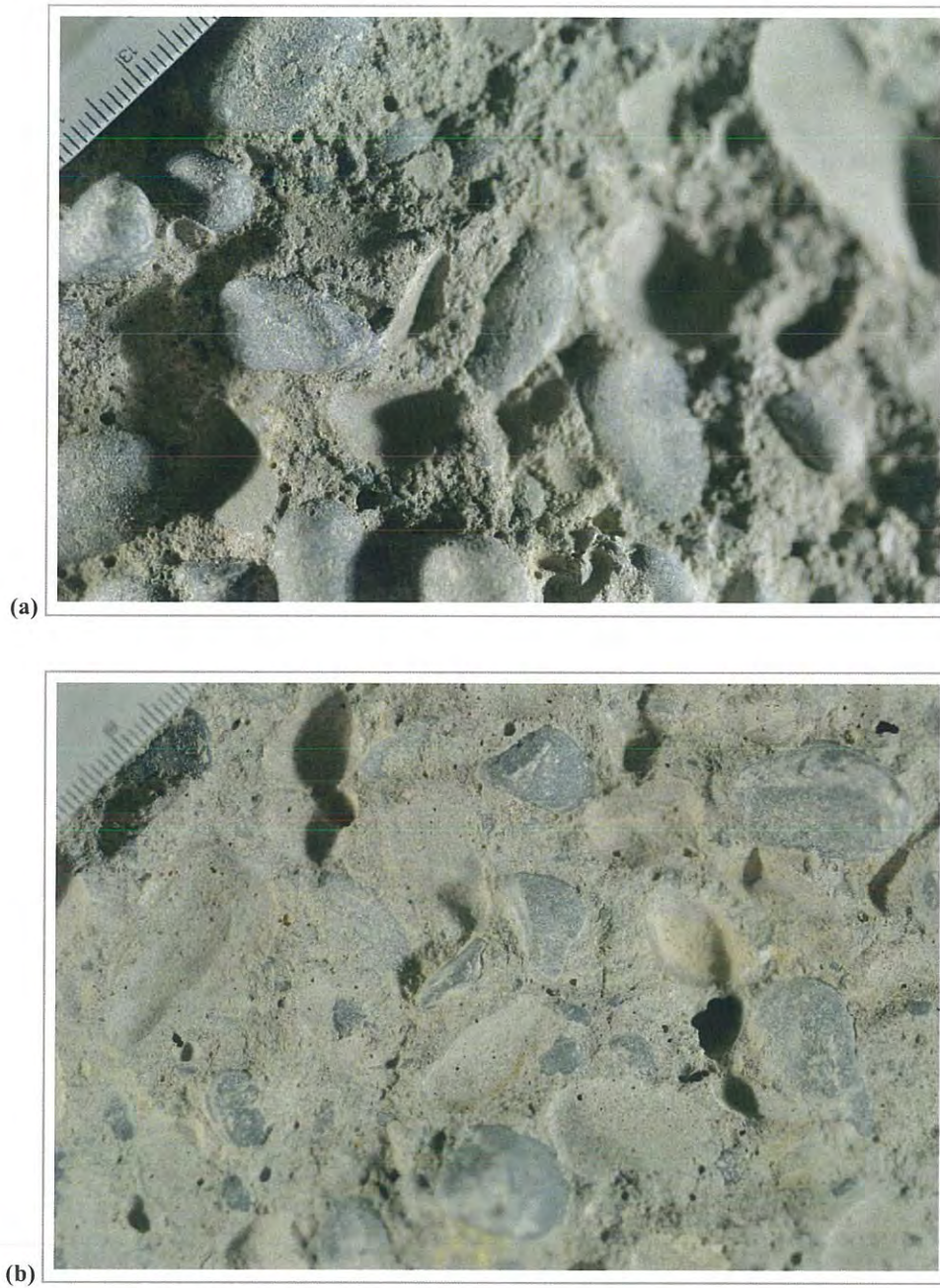
Figure H3. Photographs showing the as-received fracture surface that separated the core into two pieces. The bottom fracture surface of the top piece is shown in (a) and (b) shows the top fracture surface of the bottom piece. Scale in millimeters in both photos.
