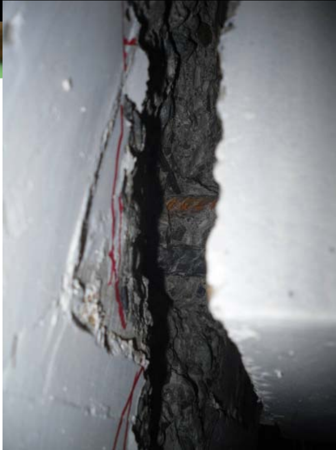
Exterior joint strain penetration
