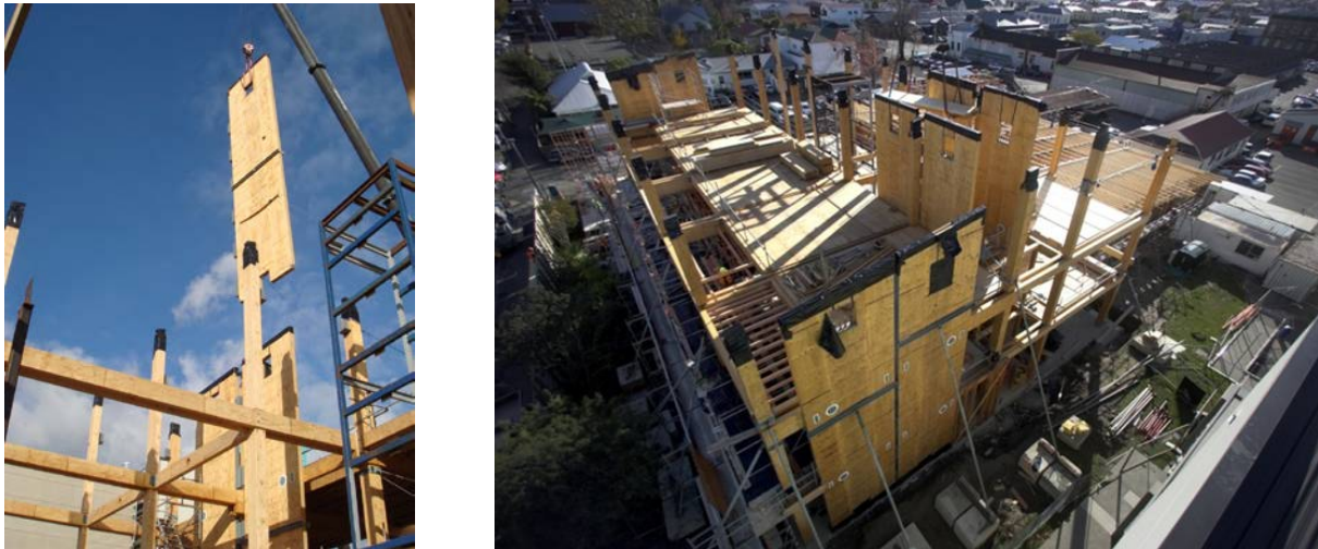
Figure 3. Photos taken during construction and installation of LVL post-tensioned and coupled shear panels.
