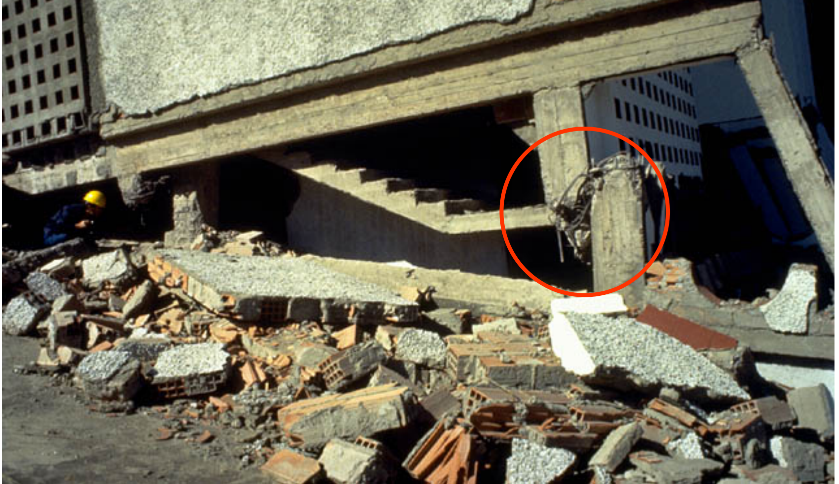
Structural interference - Short Column Effect El Asnam Earthquake, Turkey 1980 [EERC archive, UC Berkeley].
