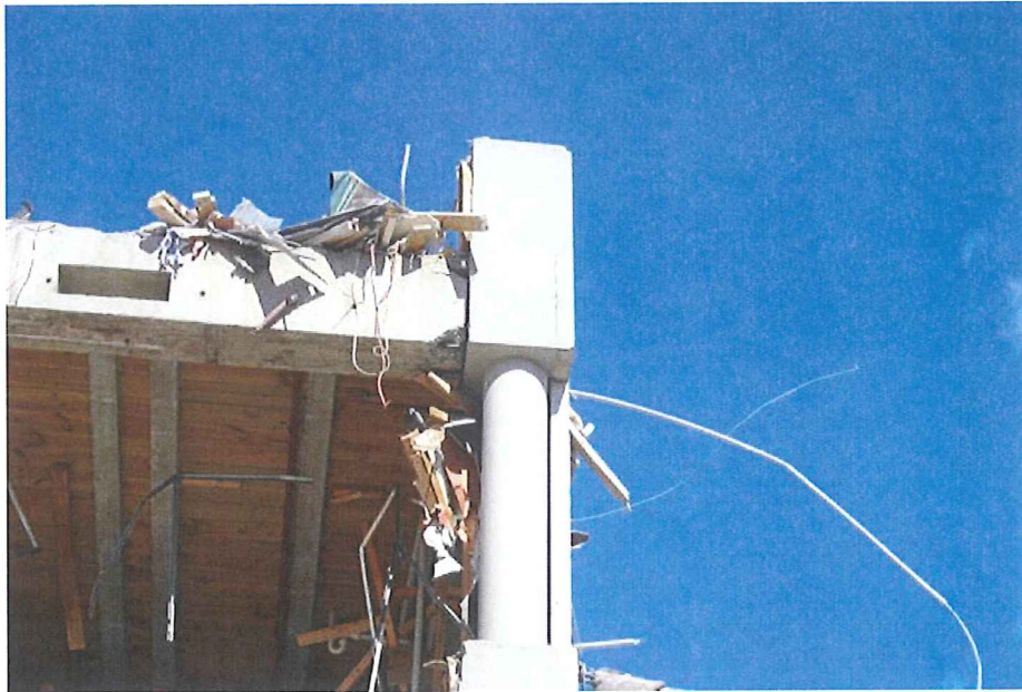
Damage to west end of north wall frame - upper levels
