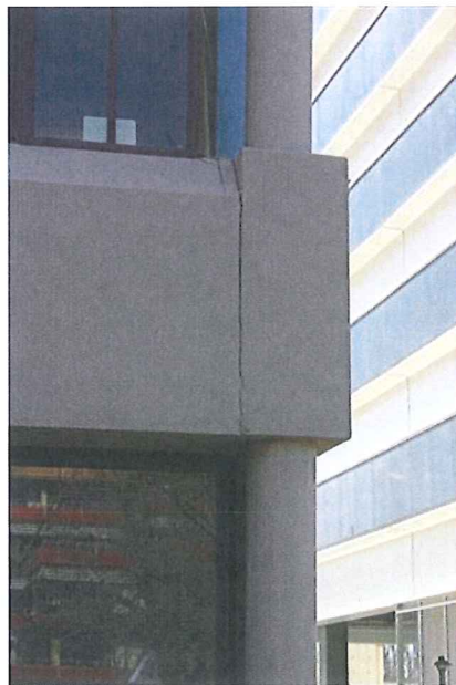
Damage to east end south wall frame
