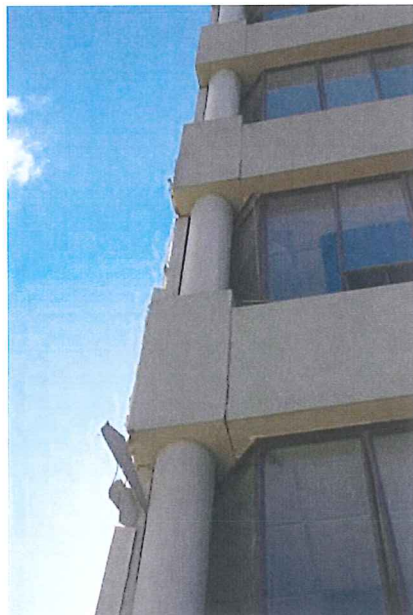
Damage to south wall frame
