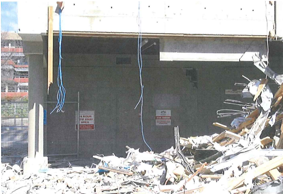
Damage to east end north wall – ground floor
