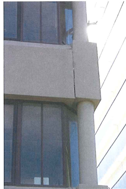
Damage to east end south wall frame
