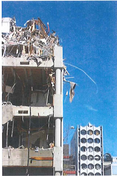
Damage west end north wall frame - upper levels
