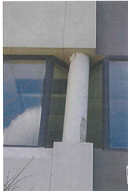
Damage to south wall frame
