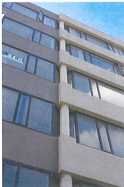
Damage to south wall frame
