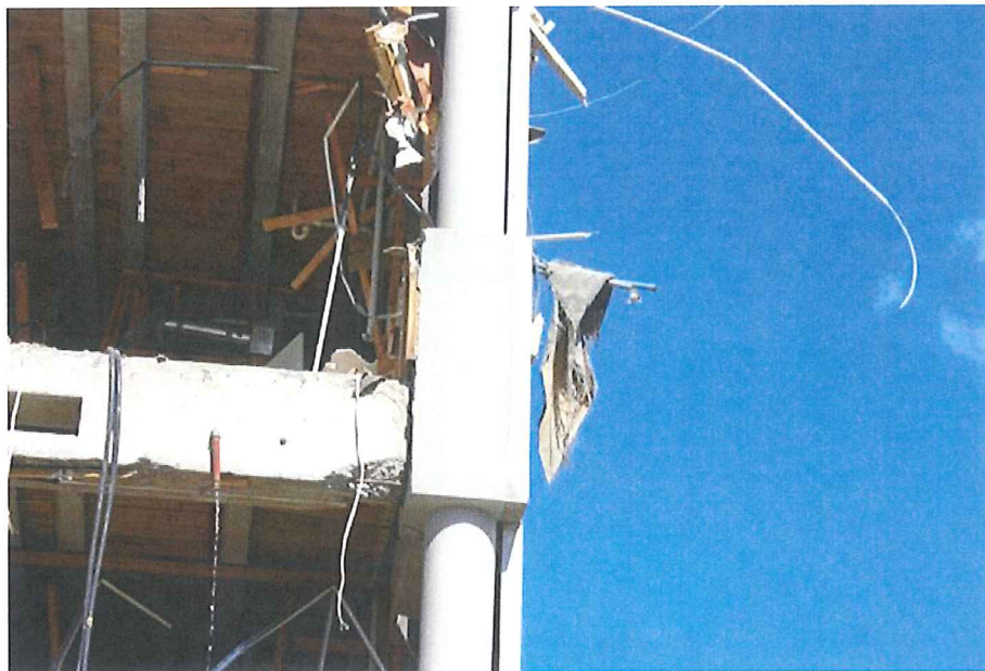
Damage to west end of north wall frame – lower levels
