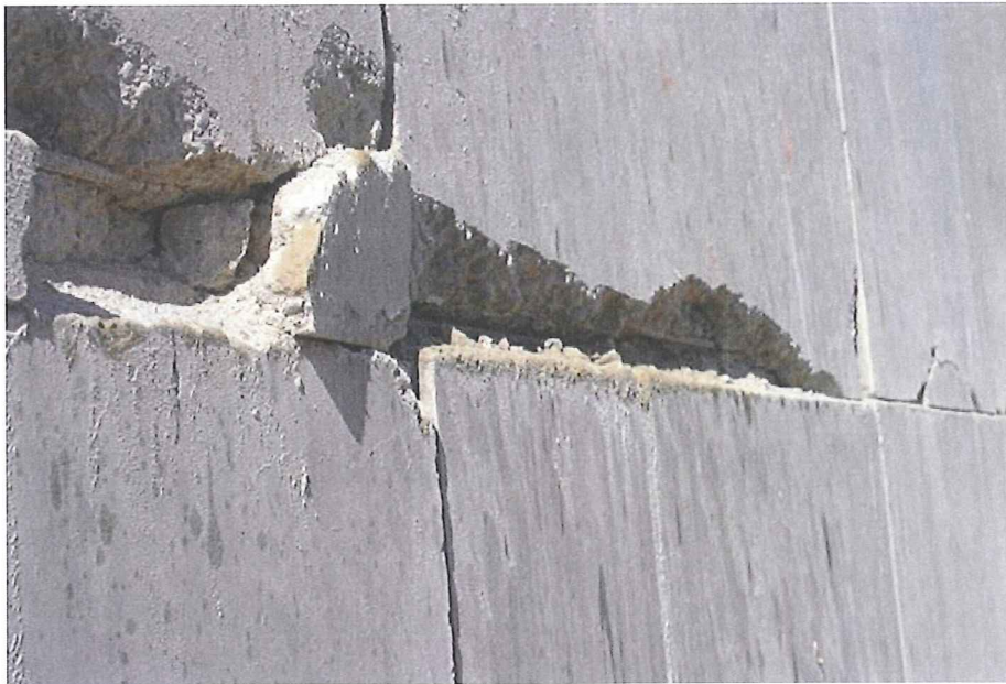
Damage to precast panels – west wall
