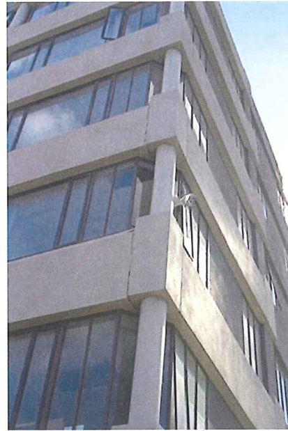
Damage to east end south wall frame
