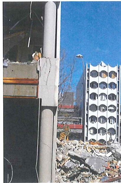
Damage east end north wall frame – lower levels
