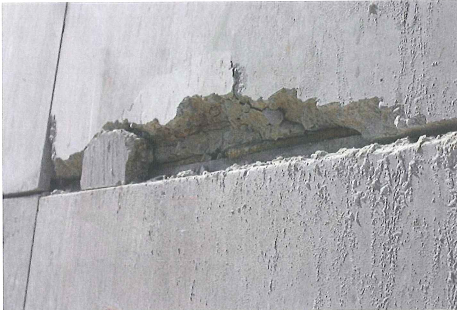
Damage to lower level of precast panels
