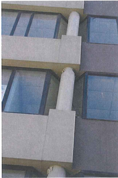
Damage to south wall frame
