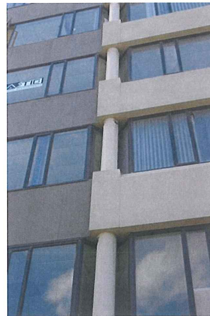
Damage to south wall frame
