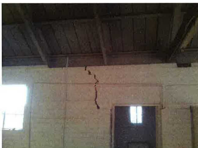
Figure 3 - Crack west wall, 15th September 2010
