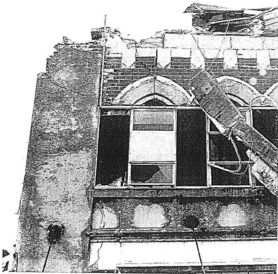
Photo 4: Damage to 1st floor and 2nd floor spandrels
