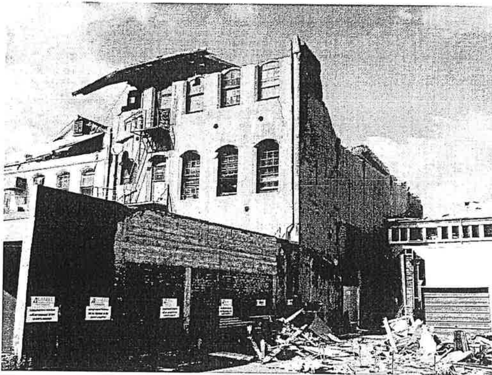
Photo 2: Northwest corner of building showing only remaining 3rd floor walls and roof.
