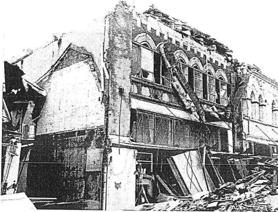
Photo 1: Southwest corner of building show loss of 3rd floor, façade glazing and canopy.
