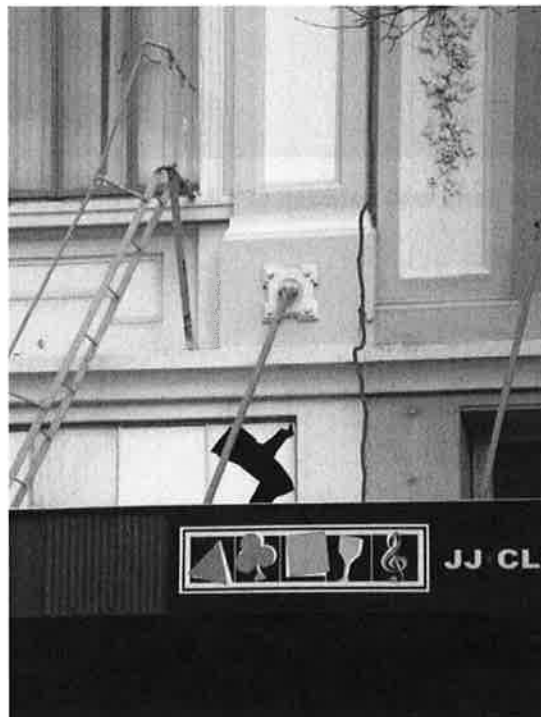
Photo 4: Crack between buildings
