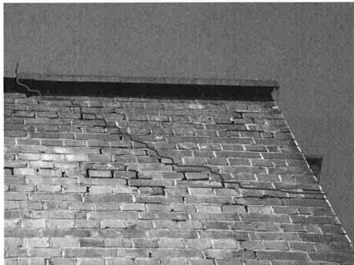
Photo 9: Masonry crack at NW parapet
