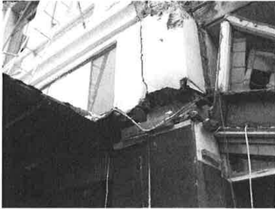
Photo 5- Crack at party wall interface.
