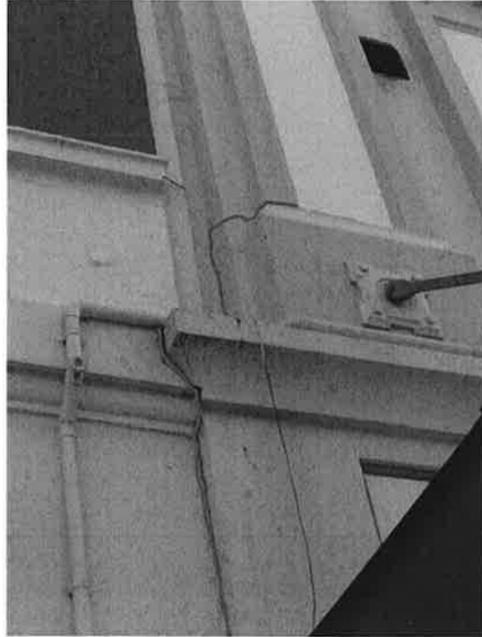
Photo 7: Cracking at joint between 617 Colombo Street & 143 Tuam Street
