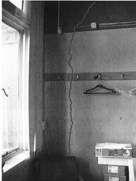
Photo 5: Crack in first floor party wall between 623 & 627 Colombo Street (taken within 627)
