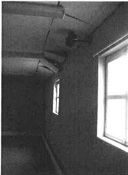
Photo 8 – Damaged tiles from fallen debris
