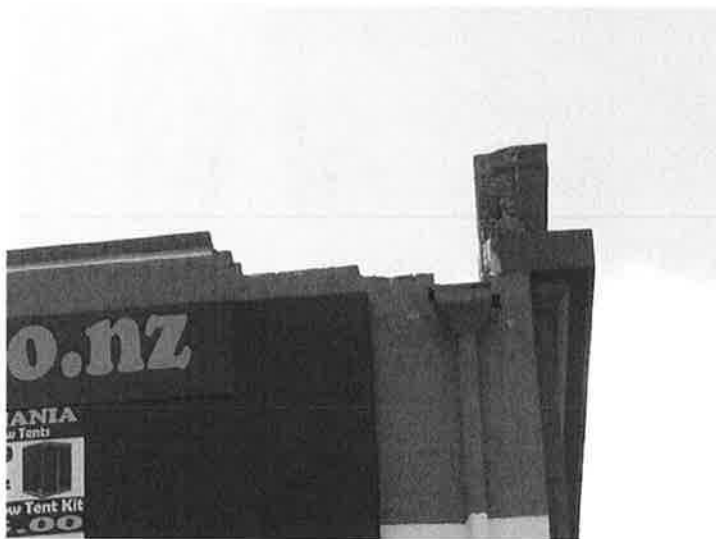
Photo 11: Partial collapse of SW parapet following aftershock
