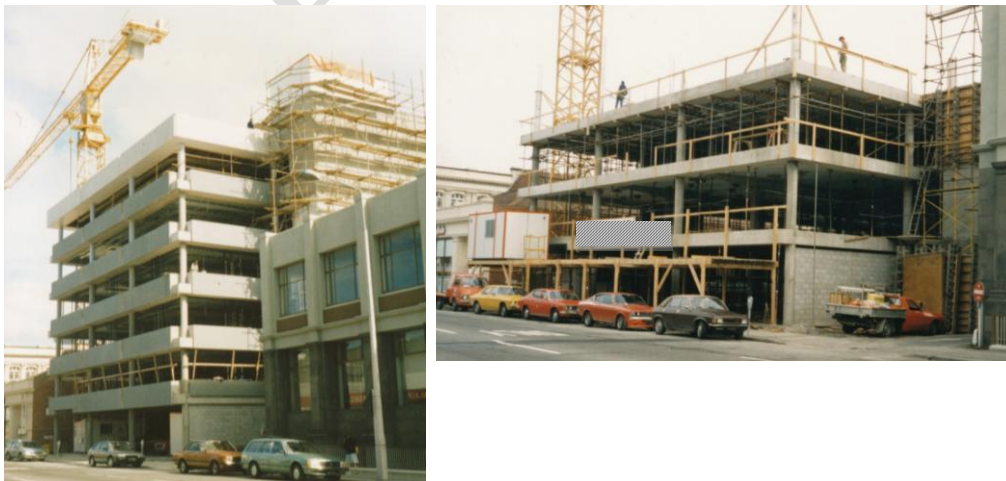
Figure 64 Building from Madras Street during construction showing spandrel panels on Line F and 4 fitted in between columns above floor levels
