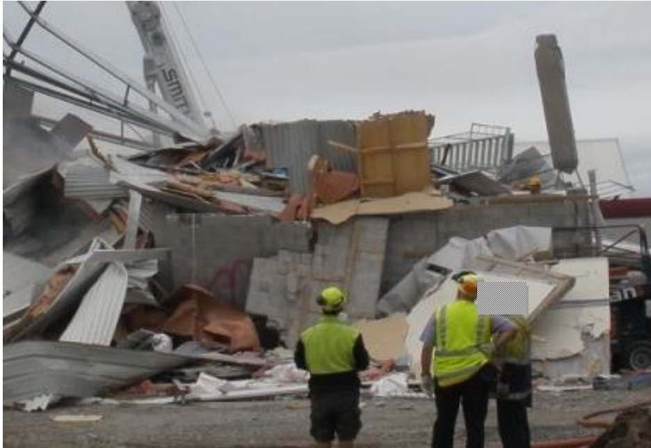
Figure 83 West wall shortly after collapse. The corner Grid 1/A column is still standing and the wall panels have broken free in panel sections in places. The edges of the panel section are square consistent with the design drawings
