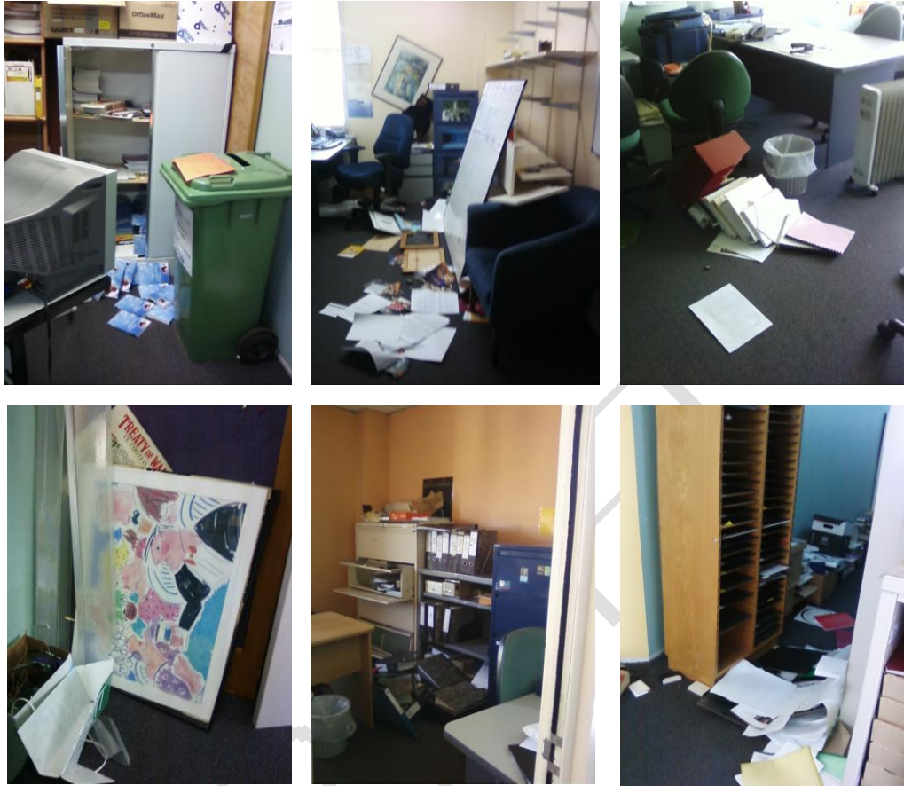
Figure 13 Damage after 26th December , 2010 after-shock on Level 6 of CTV Building (clockwise from top left) a) Cabinet door had opened but hadn't fallen over though not attached to the wall (Line 3/B-C); b) As it was except that the filing cabinet had been stood back up (Line 2/A-B); c) Oil heater had been righted. Two filing cabinets had fallen to the floor; (Line 1/B-C) d) The cubby-hole unit had not emptied of papers in the earthquake on 4 th September. However in December it had fallen against the corridor wall towards Cashell Street. It had been righted before the photo was taken (Line 2/B-C) E) The shelves and filing cabinets had gone down, but had been righted before the photo was taken (Line 4/A-B). F) The painting had fallen from the wall. (Line 1/A-B).
