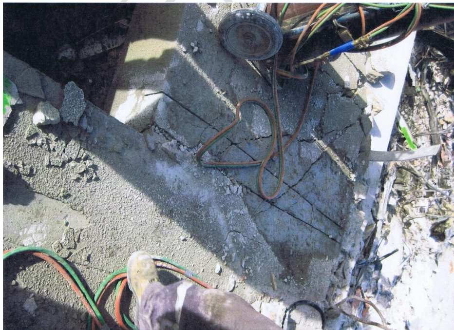
Figure 75 Line 1 shear wall at Level 4 being prepared for cutting and removal. Shear cracking in panel is visible under cutting equipment and hoses.
