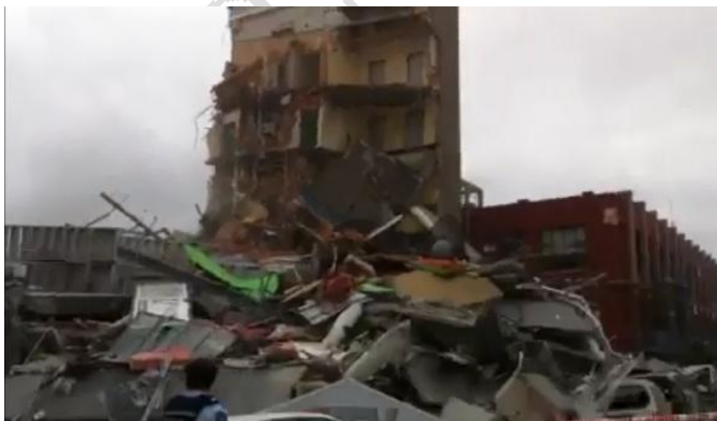
Figure 44 Corner of Cashell and Madras Street faces (Line 1/F). Fractured columns in foreground
