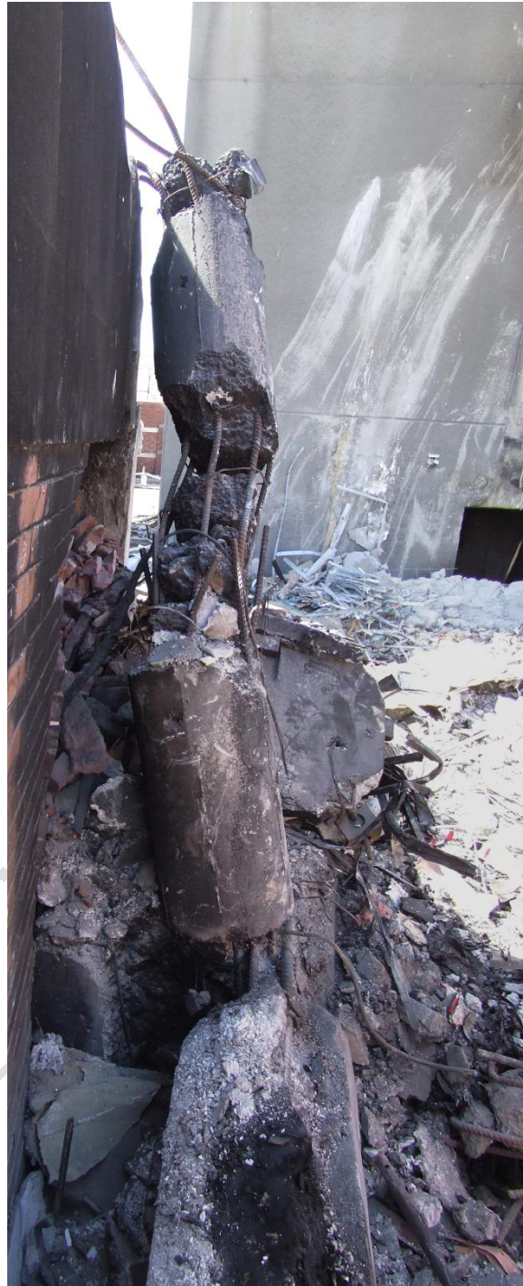
Figure 69 Line 4 / B spandrel column with B22 precast log beam in foreground and B23 shell beam at rear. No hinging is apparent at the base of the column compared to the perimeter column Item E33 (refer Site Examination and Materials Test Report)
