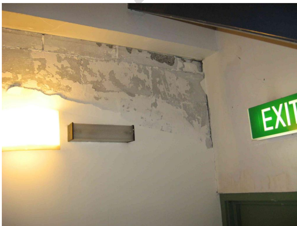
Figure 8 (Top to Bottom) a) hairline cracking in slab at Line 1 shear wall door at Level 4; b) Damage to plaster on infill blockwall at Level 1 Line 4
