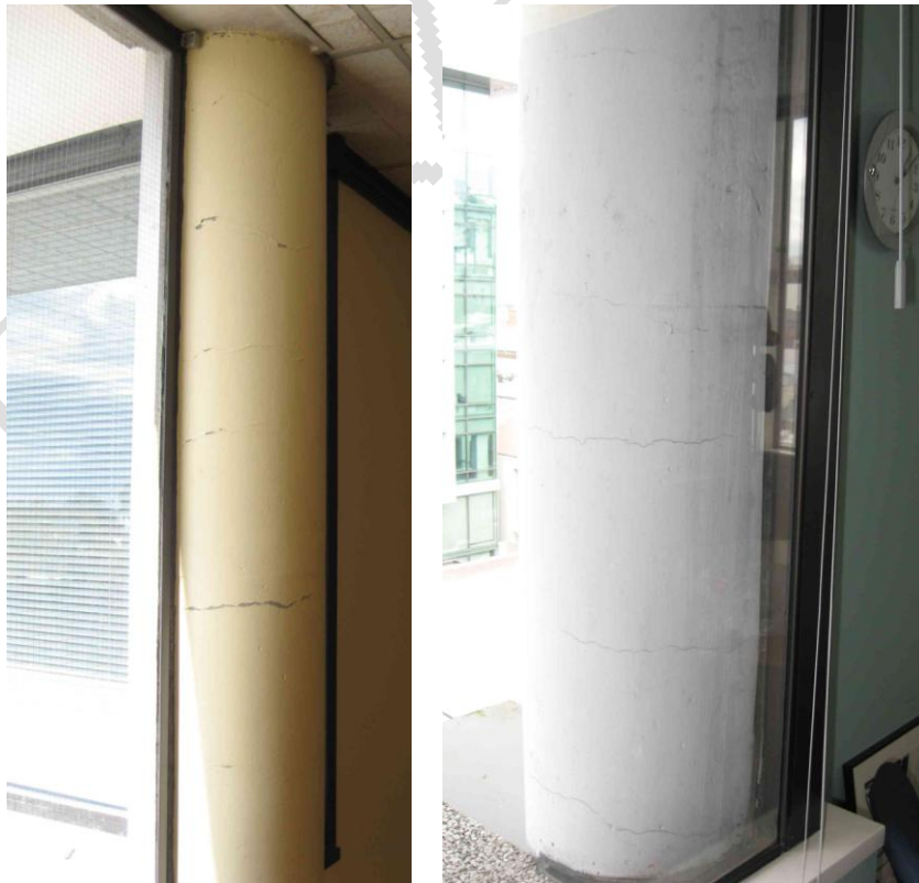
Figure 7 Level 6 400 mm diameter columns (Left to right) a) Column C18 outside lift; b) Column C3 on Line 1/A-B with hairline horizontal cracking
