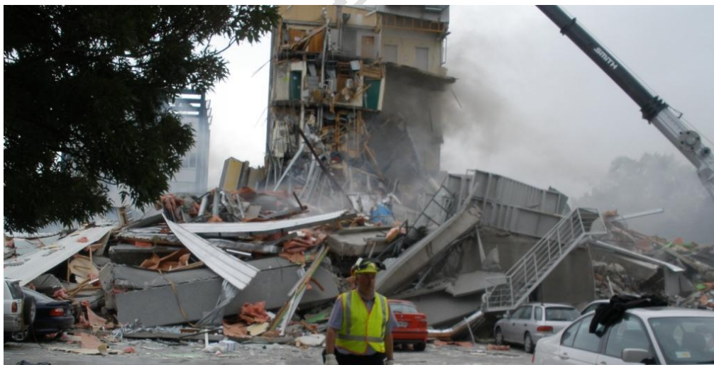
Figure 43 Western end of south face (Line 1). Collapsed Line shear wall with escape stair to the right.
