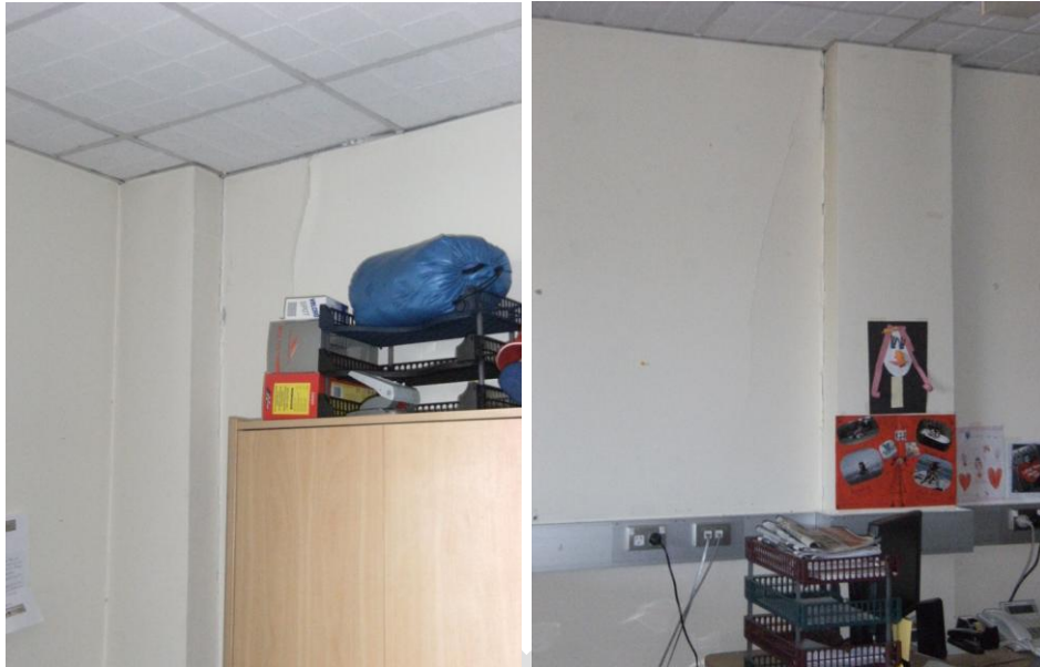
Figure 81 Inside of the west wall on Level 2 after the 4 th September earthquake shows some damage to the linings
