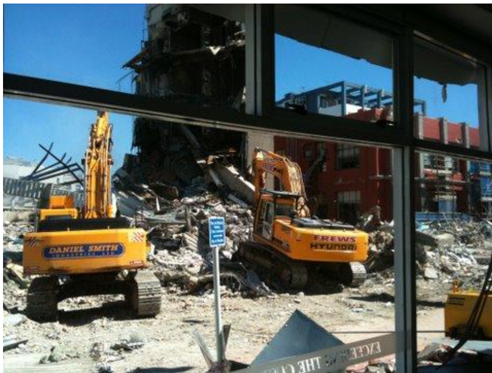
Figure 50 Debris being cleared from Madras Street face
