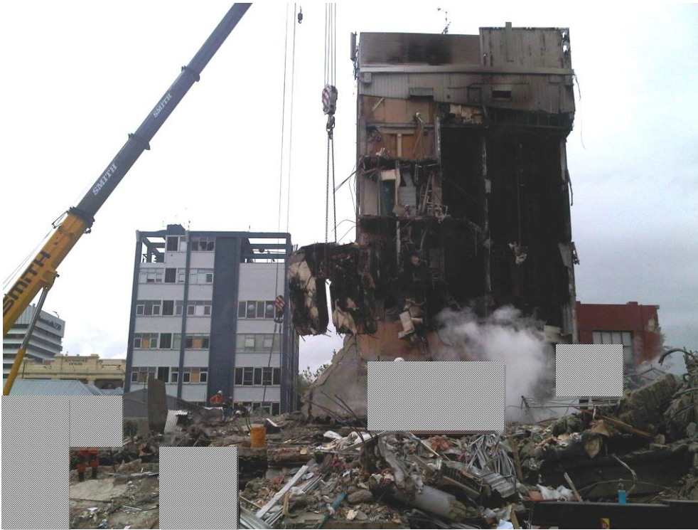
Figure 54 Portion of Line 1 shear being lifted out by crane.. The Level 6 slab in front of lift core has been removed for safety reasons.
