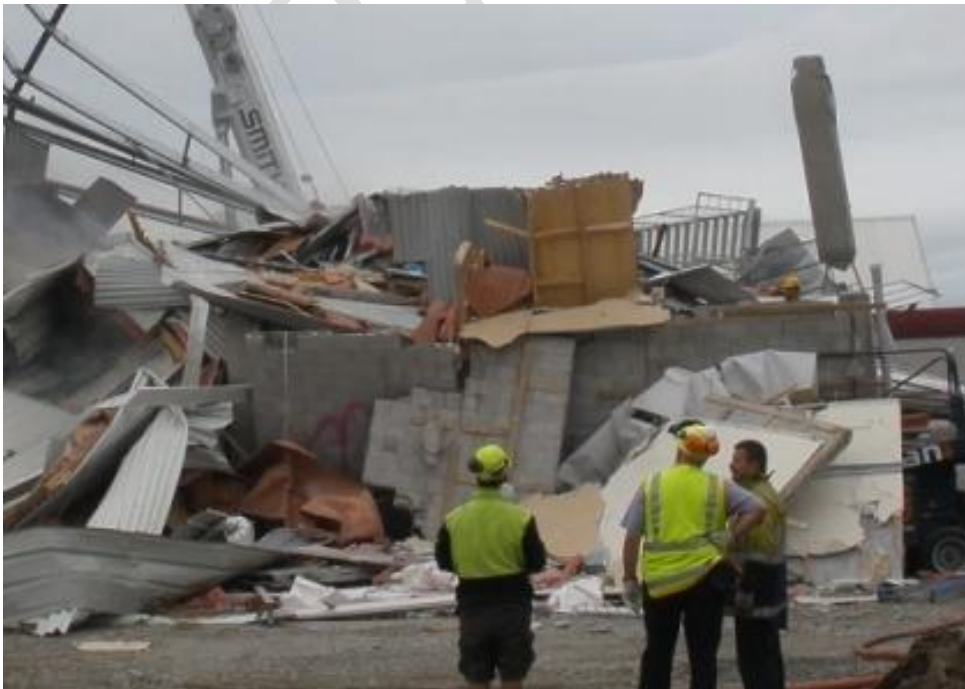
Figure 40 South west corner (Grid A/1) with corner column still standing. Collapsed work platform under wall panels.
