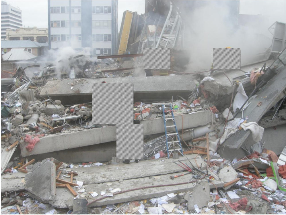
Figure 63 Concrete spandrel panels, perimeter beams and columns on Cashell Street face (Line 1 / B-D)
