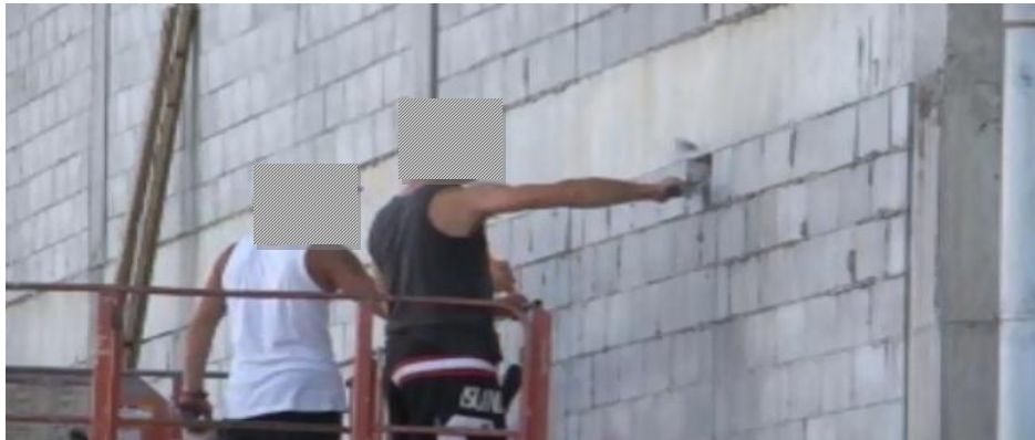
Figure 78 Workers hammering face of top course block away on west wall near Line A / I corner column
