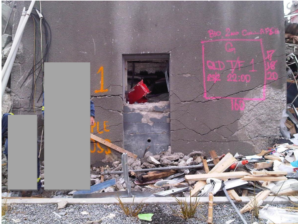
Figure 74 Line 1 shear wall at Level 1 showing masonry in-fill at door opening, in-plane flexural cracking and spalling of concrete at right (east) end
