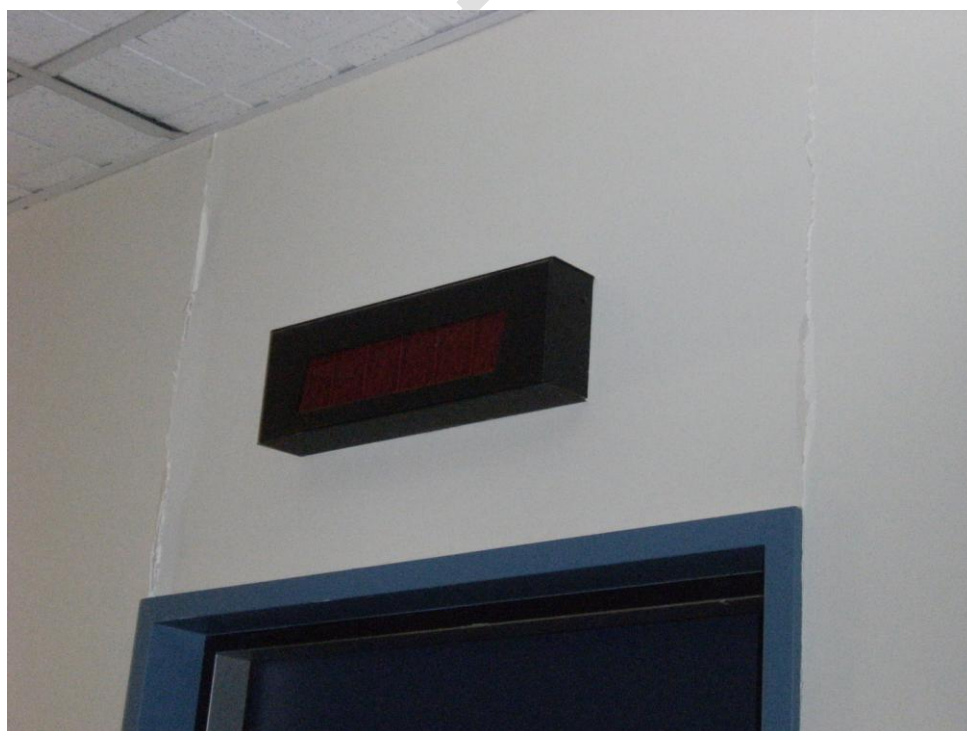
Figure 10 damage to wall Linings
