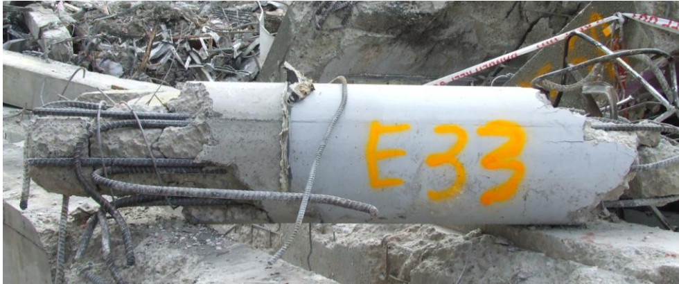
Figure 70 Perimeter 400 mm diameter column with spalled base and bar lapping zone at left unpainted portion that would have been located at spandrel panel infill areas (refer Site Examination and Materials Test Report)
