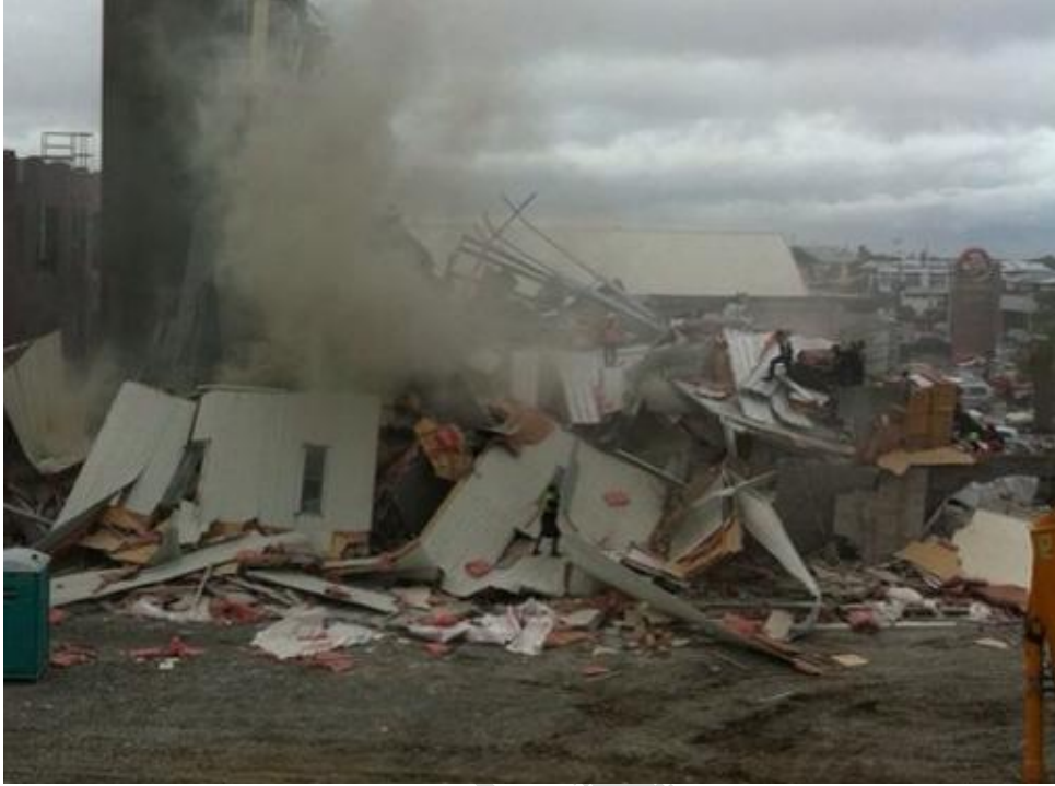
Figure 39 West side of building with lift core partially obscured by smoke, prior to heavy machinery removing debris
