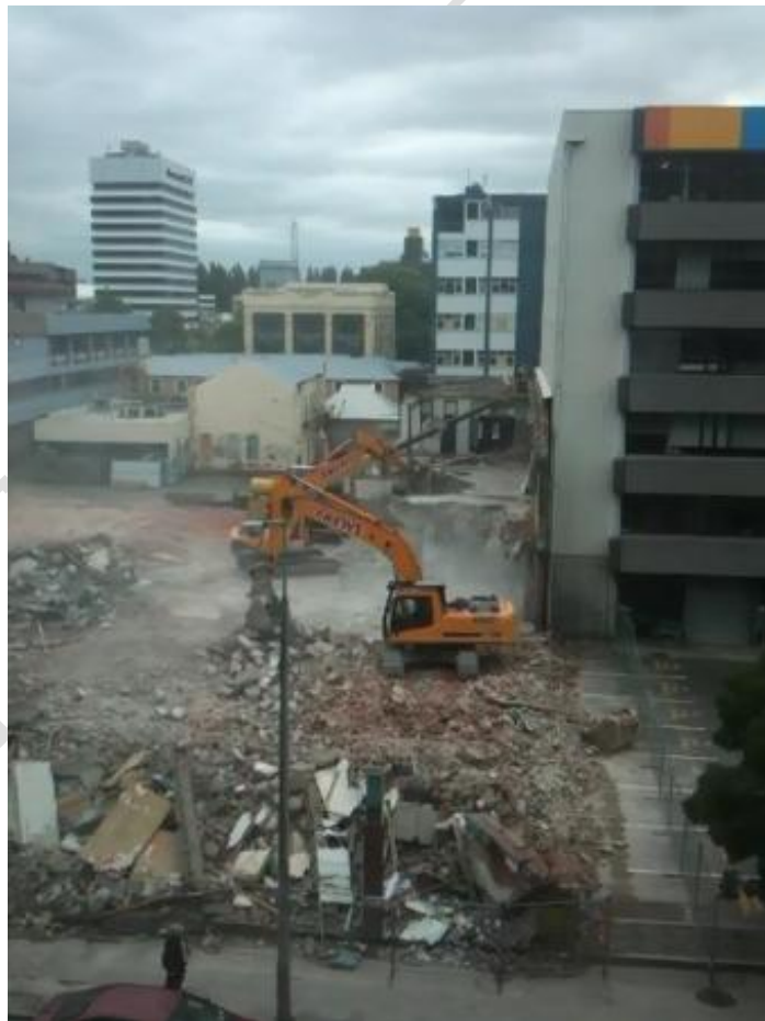
Figure 12 Heavy machinery demolishing a reinforced concrete building adjacent to the CTV Building after the 4 th September, 2010 earthquake.
