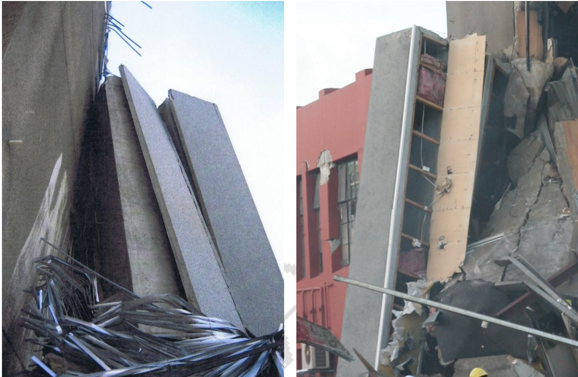
Figure 65 Line 4 / B-C spandrel panels against tower wall, showing (left to right) a) View from north face; b) View from west showing timber framing for wall linings
