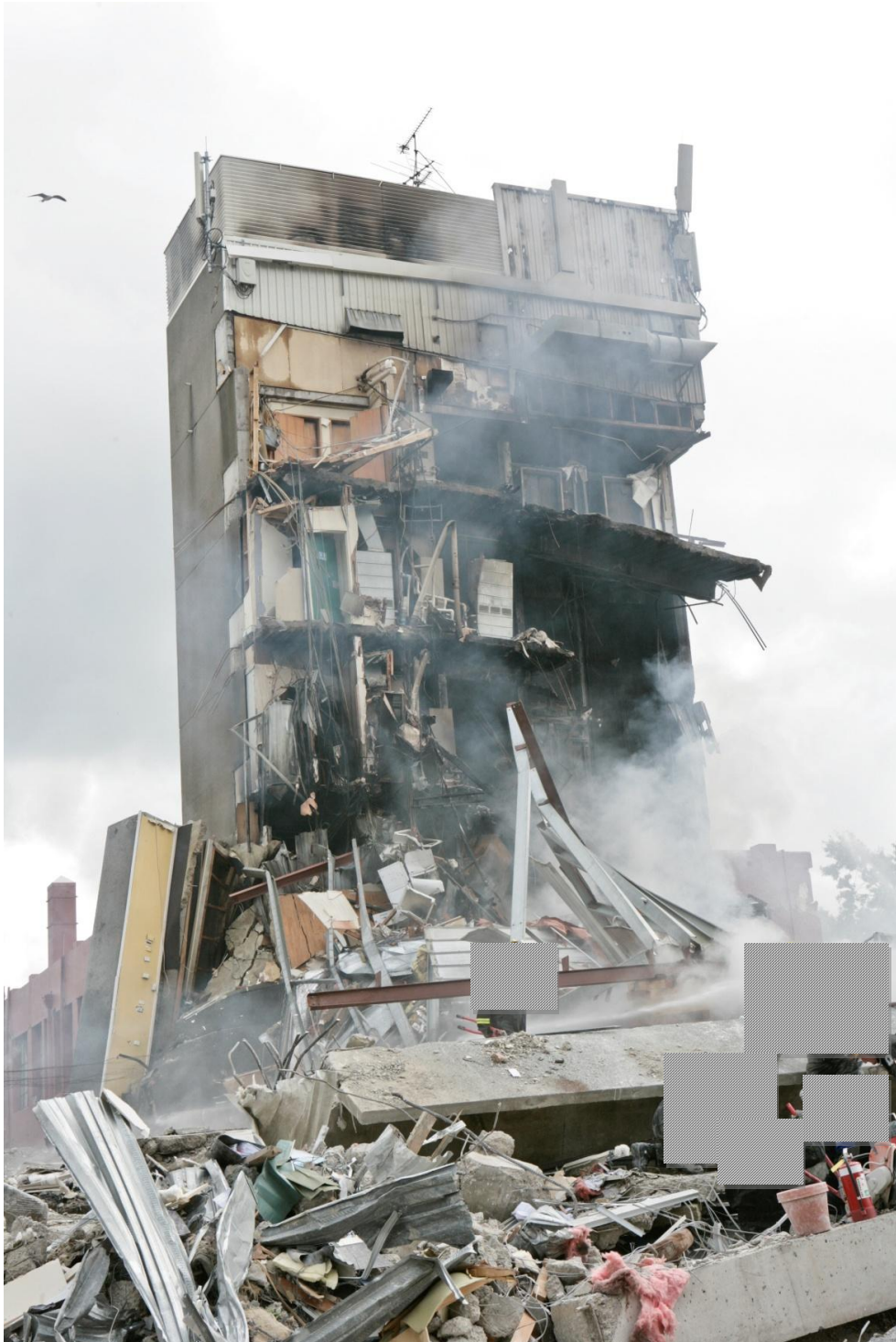
Figure 49 Spandrel panels and beams at Cashell Street Line 1 and on Line 4 in background standing vertical. Roof debris visible.
