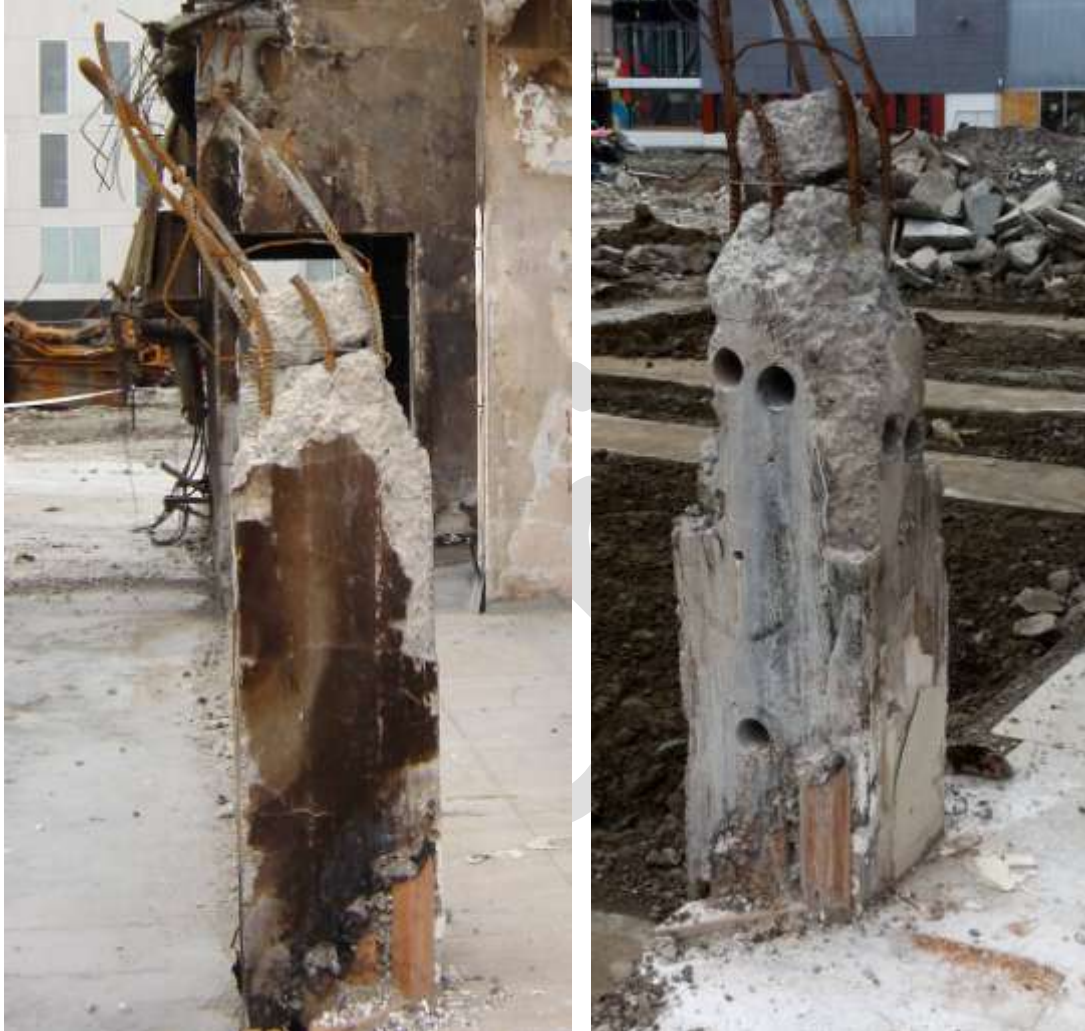
Figure 40 400 mm Square Column C18 at Grid 4/D.5 adjacent to lift core walls showing compressive failure (left to right) a) Spear head shape of failure surface indicative of compressive failure. Fire scorching to surface from smouldering fire; b) Holes showing locations of drilled cores extracted for compression testing.
