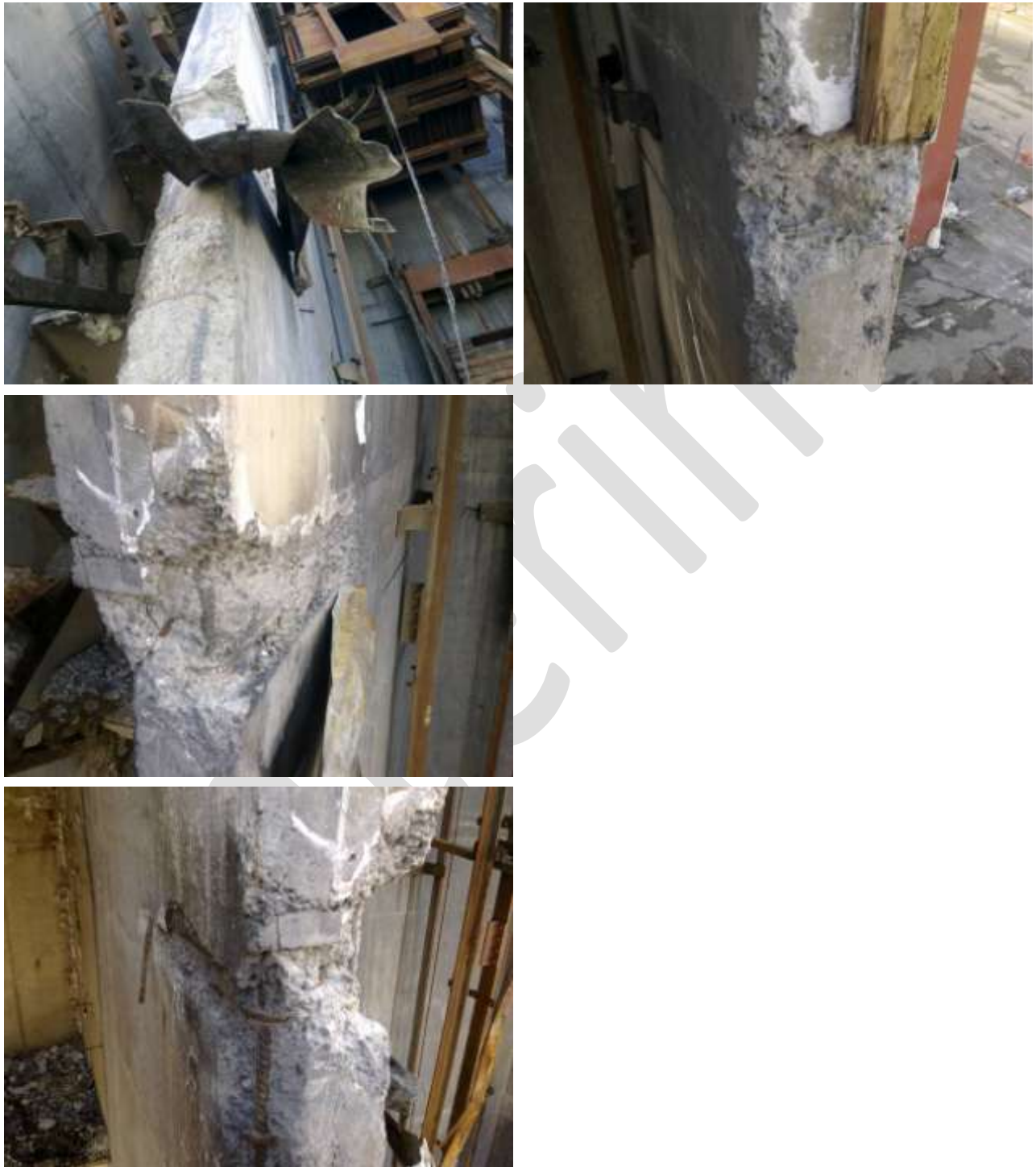
Figure 28 Level 3 Lift Well Wing Walls Grid D and D.5 (anti-clockwise from top left) a) Hi-bond decking side lapped into western Grid D wall, just hanging on; b) H12 bar necked and fractured at centre of wing wall ( indicated by chalk arrow). c) Concrete cover broken away as slab pulled southwards; d) Localised spalling of concrete. No reinforcing found connecting end of east wall with slab.
