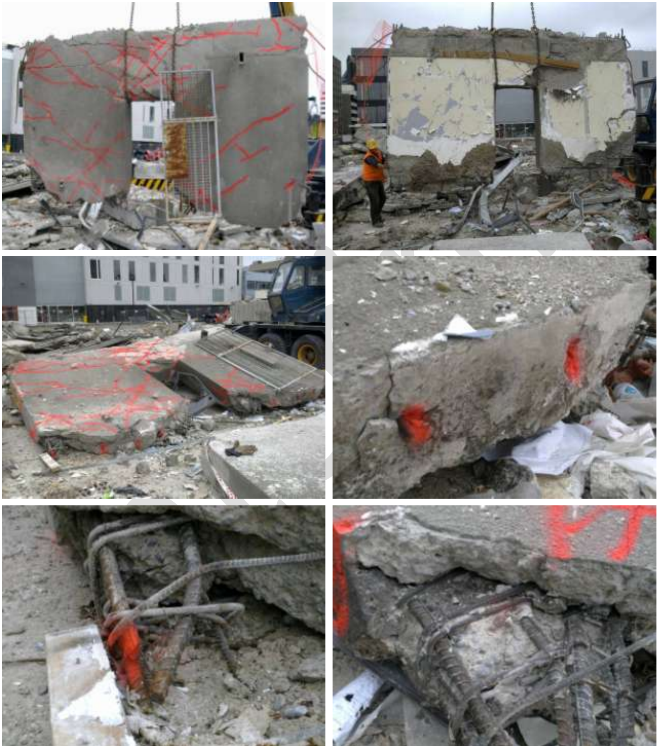
Figure 13 Line 1 Shear Wall Level 2 to Level 3 (Item E2) (clockwise from top left) a) Outside face with fire escape door attached. Cracks marked by red paint; b) Inside face of wall; c) east pier construction joint with necked and fractured bars indicated by red paint; d) Escape door edge of east pier showing thick cover concrete to reinforcing; e) Outer edge of west pier showing necked and fractured bar indicated by red paint others were cut; f) Outer face of wall with cracks and fractured bars marked.
