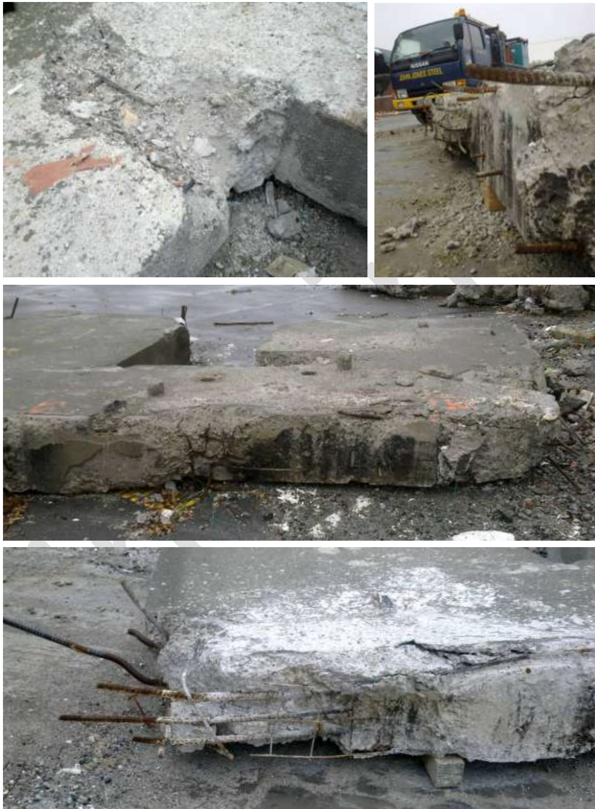
Figure 16 Line 1 Shear Wall Level 5 to Level 6 (Item E5) (clockwise from top left) a) Crumbly concrete at door edge of west pier able to be dislodged by boot; b) Smooth and charred construction joint on top west surface looking east; c) Charred construction joint above west pier. Door sill on left; d) Top east corner with fractured top 3-H24 bars. Floor 664 mesh exposed.
