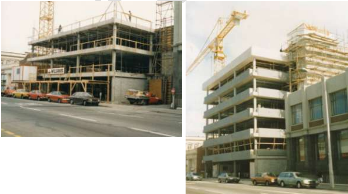
Figure 41 CTV Building under construction (left to right) a) May 1987 with floors cast up to Level 4; b) October 1987 with roof on and pre-cast spandrel panels attached; Columns C21 to C23 had not been built at that time in the northeast corner closest to camera.
