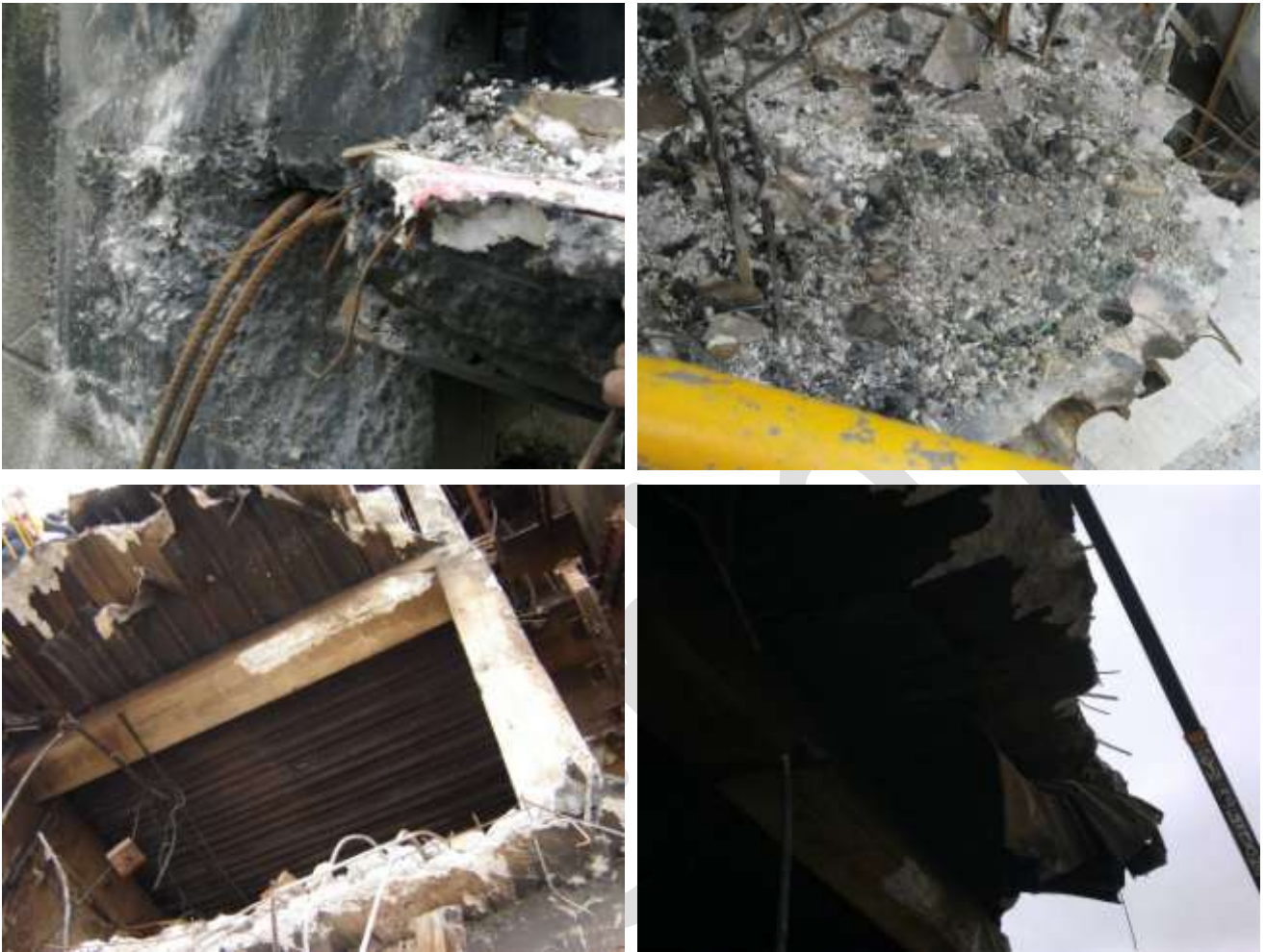
Figure 23 Line 4 Core Walls Level 3 slab remnants (clockwise from top left) a) Connection of shell beam to wall with two fractured H24 top bars and two de-bonded top bars. No bottom bars from shell beam embedded in wall but imprints from bars evident (DENG B23 Dwg S18 (Figure 59), Detail 5 S19 (Figure 64)), corresponding to the bent back bottom steel in shell beam Item E23 (Figure 6). b) Ash on slab. Cored holes at fractured edge. c) Torn Hi-bond sheeting de-bonded from slab but still fixed in at pre-cast beam support (DENG B24 Dwg S18 (Figure 59)). d) Hi-bond deck and slab from below supported on beam B24
