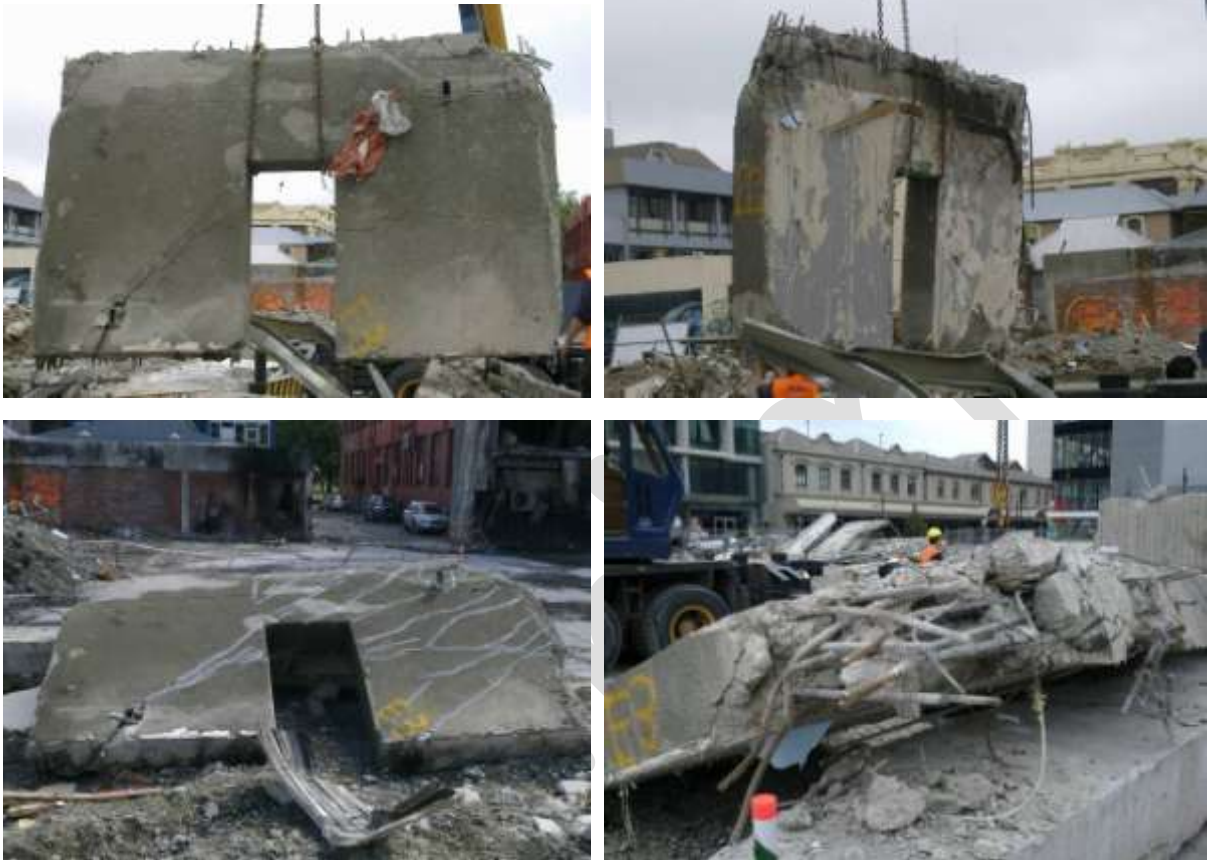
Figure 14 Line 1 Shear Wall Level 3 to Level 4 (Item E3) (clockwise from top left) a) Outer face; b) Inner face; c) Damaged top east corner; d) One way diagonal cracks running from bottom west to top east side marked by paint on outer face.
