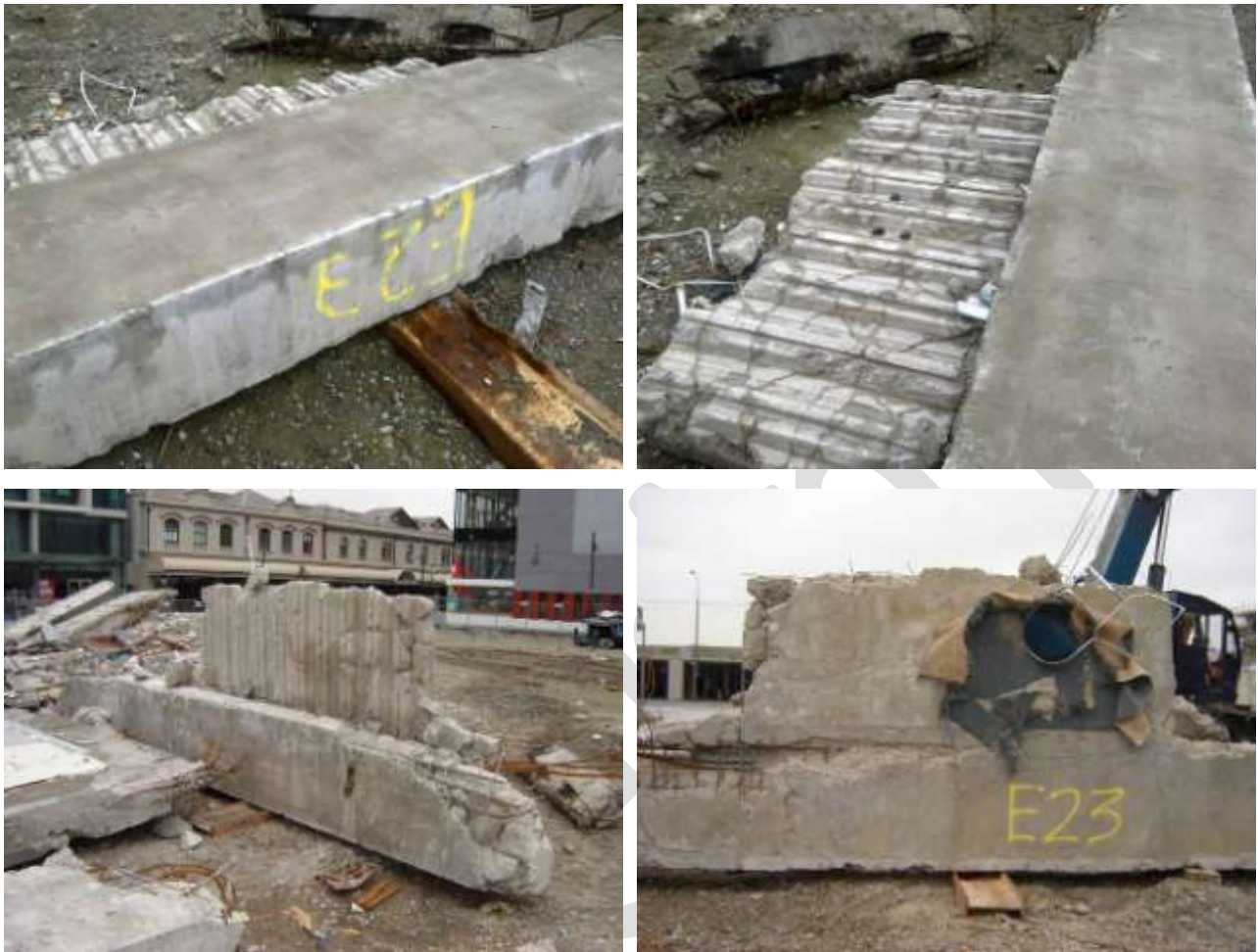
Figure 6 Edge Shell Beam (Item E23) from Line 1 or 5. (Clockwise from top left) a) Underside and outer face; b) Underside showing 1200 mm slab outstand with metal decking pulled away and diagonal cracking indicating shear in diaphragm; Holes are where concrete cores were taken for testing c) Carpet remnant on top of slab; d) Damaged shell beam.
