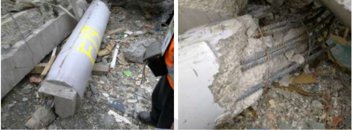
Figure 7 400 mm diameter column Item E19. (Left to right) a) Level 6 to Roof, likely location Grid F (Figure 57) based on roof steelwork hold down attachment detail; b) Flexural fracture at base in lap zone of vertical reinforcing steel. R6 spirals at 250 centres can be seen (Figure 61).
