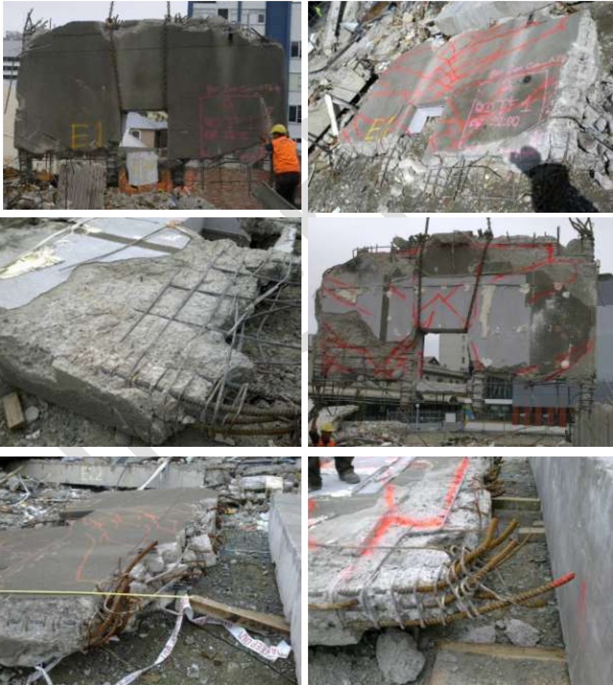
Figure 12 Line Shear Wall (Item E1) (clockwise from top left) a) Outer face of wall with lower portion of concrete removed during deconstruction exposing the reinforcing steel; b) Outer face with cracks highlighted by red paint; c) Inside face with cracks highlighted by red paint; c) Top west corner; d) Top east corner; e) Inside face of east pier
