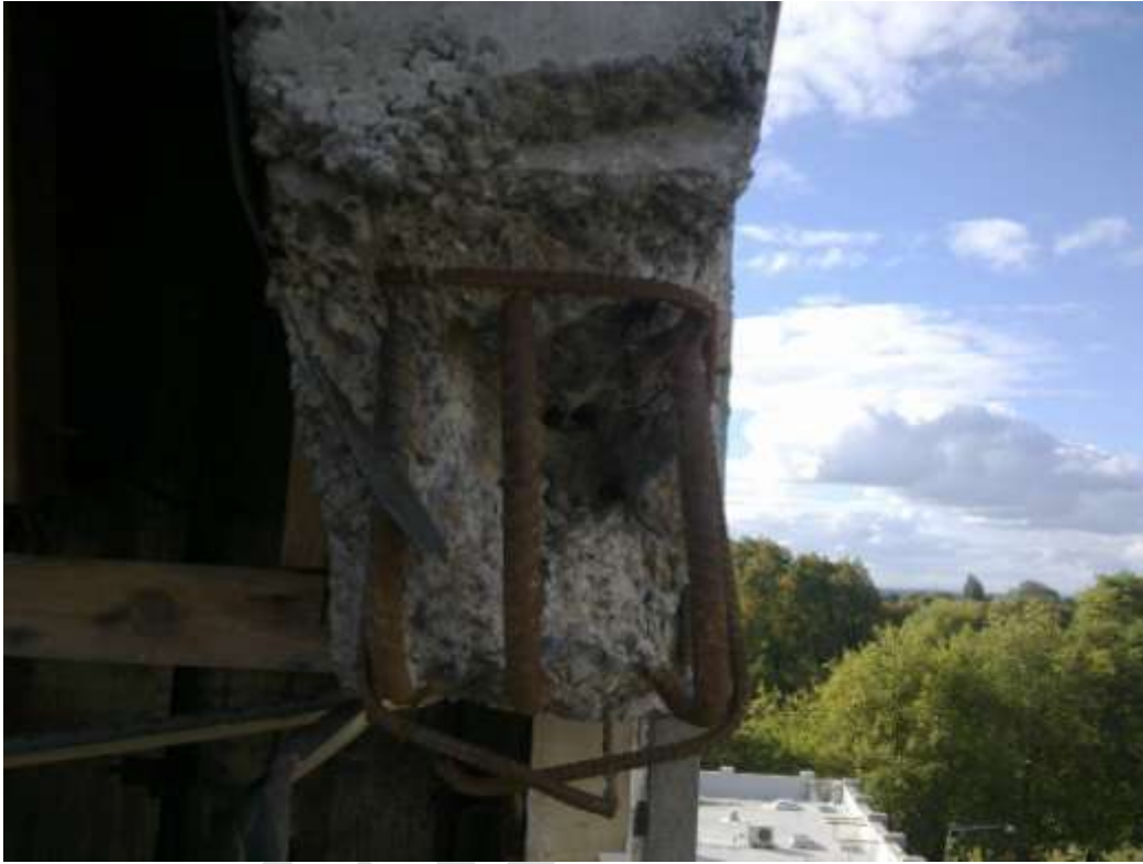
Figure 33 Lift Well Wing Wall D.5: Column C18 Connection (DENG Dwg S14 (Figure 61)); 3 x 20 to 24 mm diameter holes can be seen where reinforcing bars from column have pulled out. The drawing shows that 4-H20 bars were required to be bent in to the wall.
