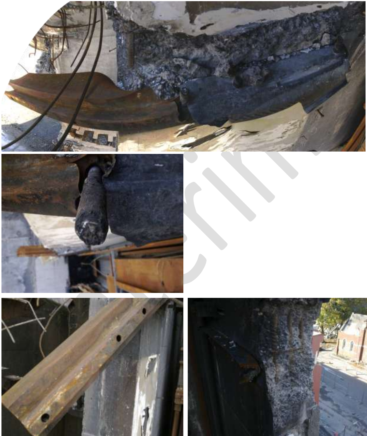
Figure 31 Level 5 Lift Well Wing Walls Grid D and D.5 (anti-clockwise from top) a) 150x150x10 L with 50 x 3 SHS; 4-M24 bolts into wall and 6 –M20 bolts 350 mm long bolted through the slab at Hi-bond rib with epoxy grout around bolt; Three M20 bolts remaining in the Grid D drag bar have fractured in tension-shear at the underside of the bolt at the slab surface. The 50 x3 SHS has fractured in bending and tension at the bolt hole adjacent to last bolt into wall and twisted with the slab. b) Epoxy grout around bolt through slab; c) Holes for 3 M20 bolts through slab in twisted drag bar; d) 150x80x10 L drag bar with 5 M24 bolts into wall D.5. End of bar has been gas cut during de-construction.
