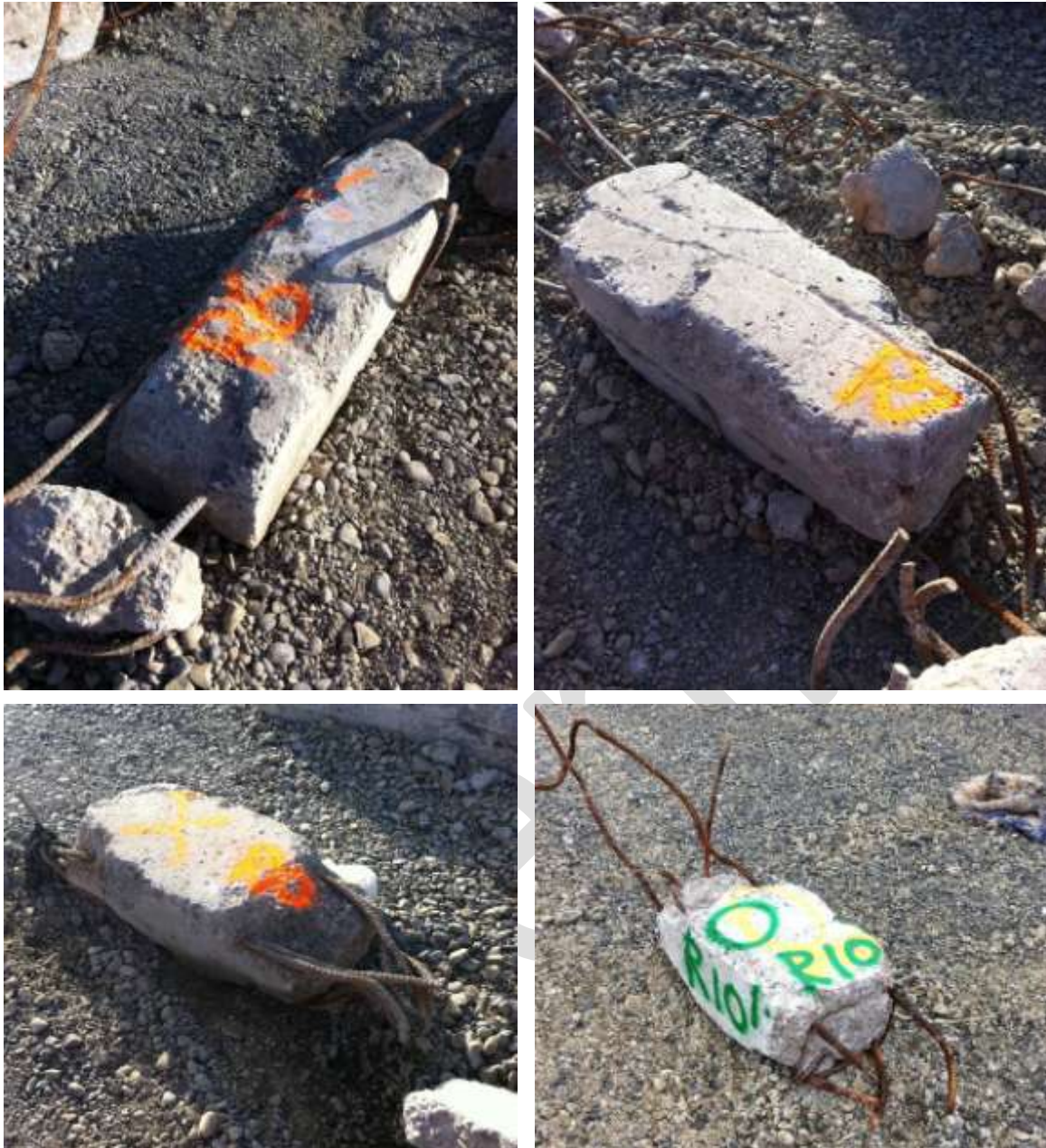
Figure 49 400 x 300 mm Rectangular Columns (from left to right and top down) a) R6 base at far end connected by reinforcing to b) R7 below, with beam-column joint failure; c) R10 remnant; d) R10' remnant.
