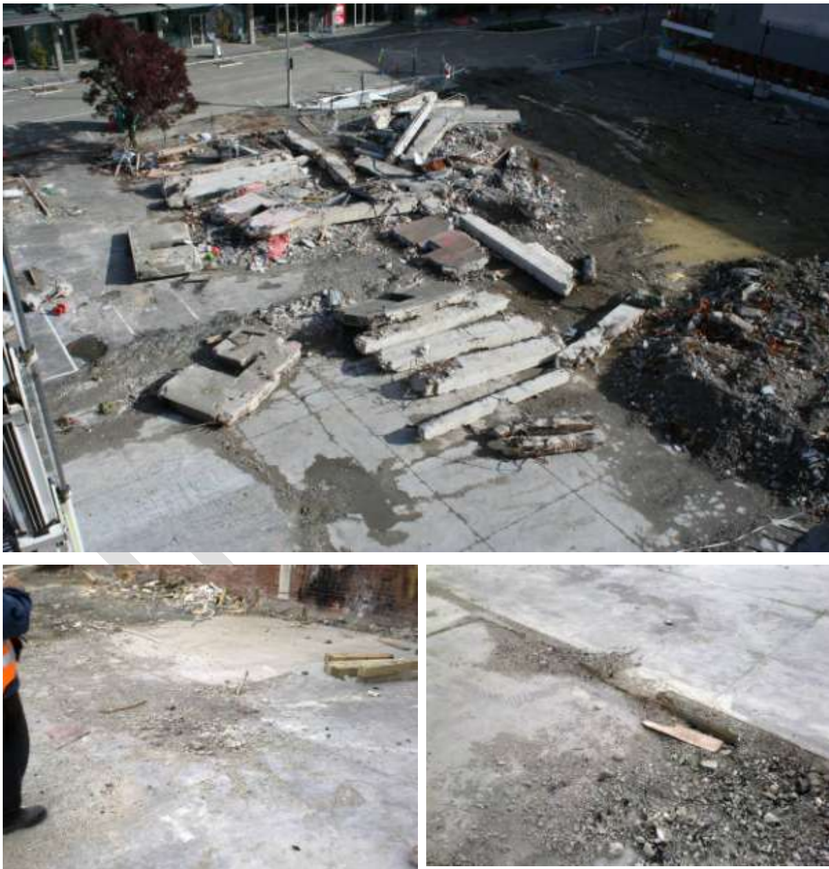
Figure 2 Ground floor Level 1 slab on grade (clockwise from top) a) View from Fire Service snorkel of debris and western portion of Level 1 slab on grade. b) Slab in northwest corner with column reinforcing protruding; c) Ramp formed in concrete overlay in front of Line 4 lift core walls.
