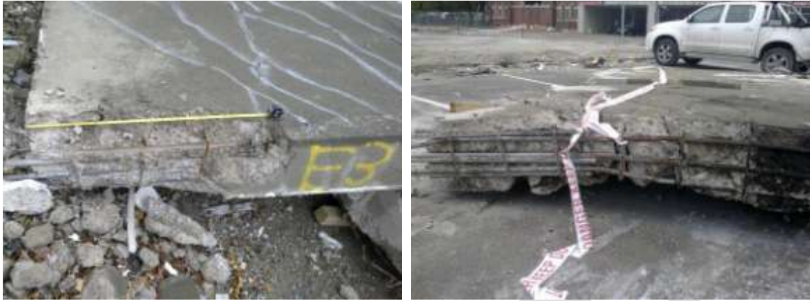
Figure 36 Locations of H24 reinforcing bar samples (left to right) a) East end of Line 1 wall item E3, one cut from lower 1050 mm of wall; b) Two lapping bars from lower E3 wall item taken from east end of wall item E4
