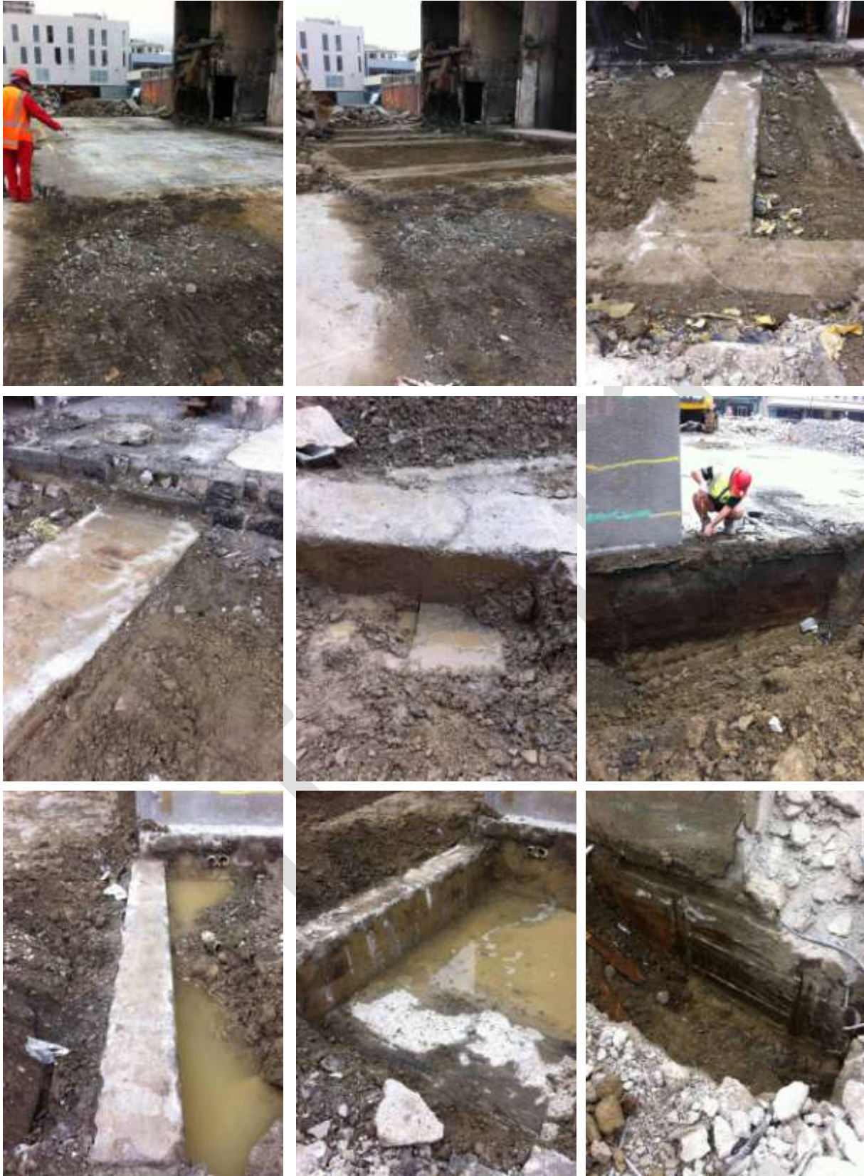
Figure 53 Foundation Inspection (From left to right in rows from top) a) P947; b) P948; c) P968; d) P971; e) P960; f) P903; g) P964; h) P919; i) P993
