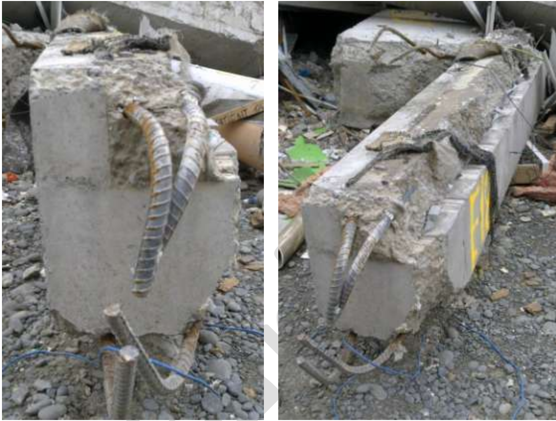
Figure 11 Item E18 Pre-cast edge beam north-west corner (DENG B22 Dwg S18 (Figure 59)) (from left to right) a) Smooth form finish at attachment to column 4A (DENG Detail 1 Dwg S19 (Figure 63)); b) No starters from pre-cast beam into slab to prevent the Hi-bond slab pulling away (DENG Section 4 Dwg S15 (Figure 58))
