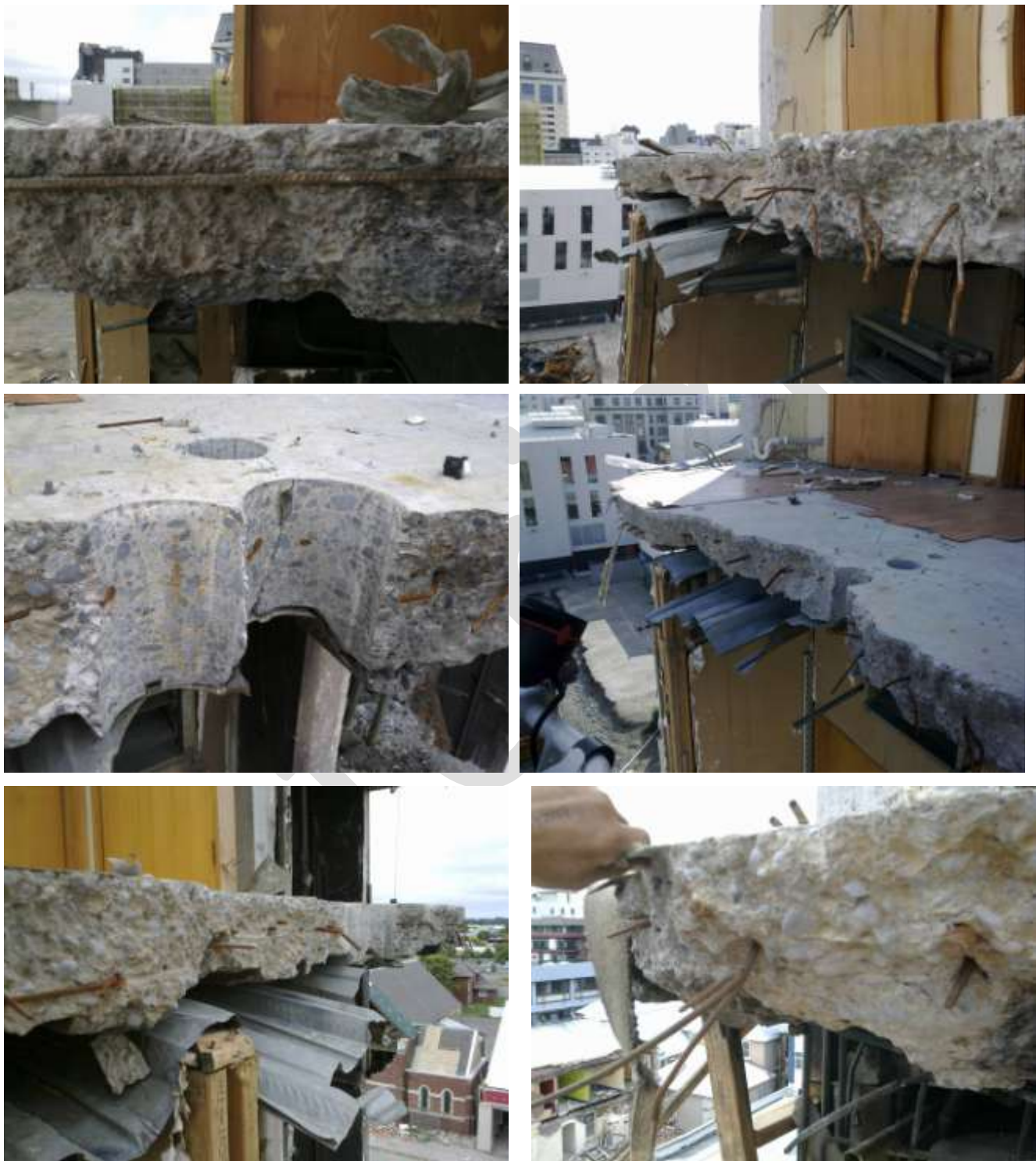
Figure 20 Line 4 Core Wall Slab Remnant at Level 6 amenity area (clockwise from top left) a) Slab edge on stairwell wall looking west with H12 saddle bar exposed and ends of mesh below it; b) Vertical concrete fracture surface with reinforcing mesh fractured; c) Slab looking west with cores cut in floor for amenities; d) Fractured mesh angled downwards; e) Fractured slab edge looking east. Torn metal decking aligned approximately with concrete fracture edge; mesh at varying height within slab; f) Cores for amenities at fracture edge.
