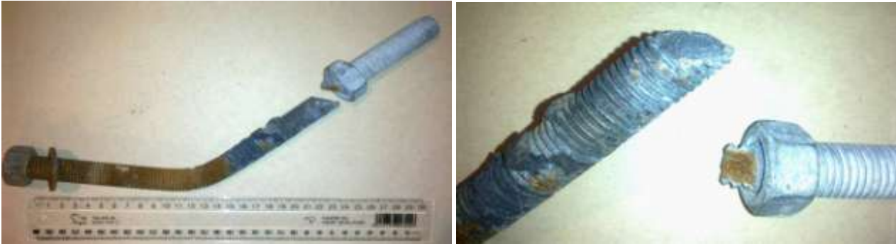
Figure 30 M20 Drag Bar Bolt (left to right) a) Rusted portion had been through underside of steel drag bar. Grey portion with epoxy residue had been in slab; Diagonal fracture surface immediately below nut. (Portions shown are from two different bolts). b) Smooth diagonal surface to left indicative of tensile fracture in combination with some shear. Necked and dimpled fracture surface at underside of bolt (to the right) typical of direct tensile fracture in threaded rods.
