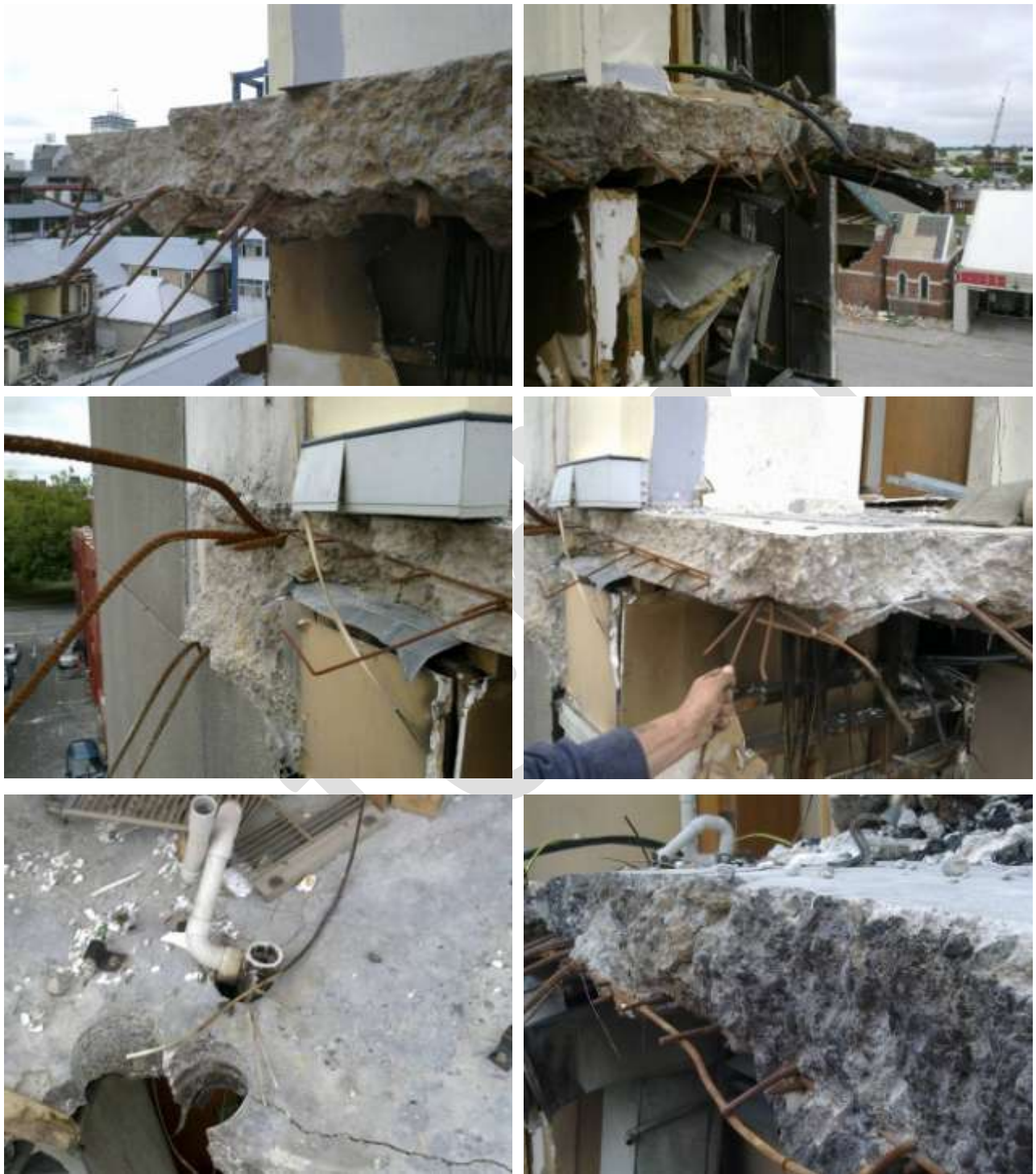
Figure 21 Line 4 Core Wall Slab Remnants Level 5 (clockwise from top left) a) West end with H12 bar ends and mesh at bottom of slab above ribs. It was required on eth drawings to be located near the top surface (DENG Dwg S16 (Figure 68)); (b) Looking east. Reinforcing angled down. c) Slab edge on Grid C west end. Mesh angled down in bottom of slab on top of ribs. d) Fire charred vertical fractured slab edges adjacent to stair well. Mesh located low down in slab at top of slab ribs. Edge of mesh sheet with closely spaced parallel wires exposed. Fractured wires can be seen from the lapped mesh below. e) Cracking in slab running from cored holes; f) Connection of shell beam to wall with two fractured H24 top bars and two de-bonded top bars. No bottom bars from shell beam embedded in wall (DENG B23 Dwg S18 (Figure 59), Detail 5 S19 (Figure 64)), corresponding to the bent back bottom steel in shell beam Item E23 (Figure 6).
