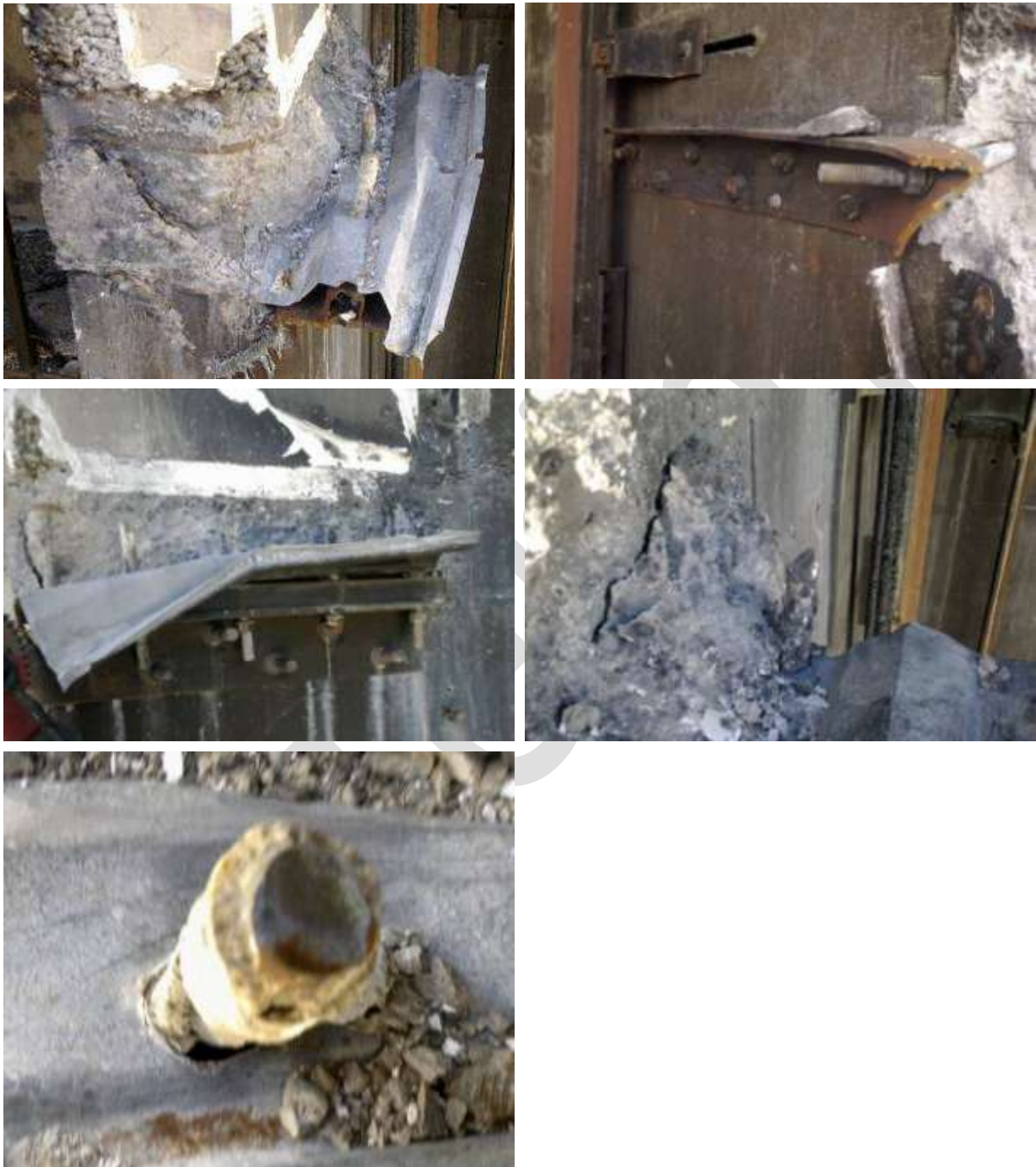
Figure 32 Level 6 Lift Well Wing Walls Grid D and D.5 (anti-clockwise from top left) a) 150x150x10 L with 50 x 3 SHS into west wall on Grid D, similar to Level 5 and 4 drag bars; 6-M24 bolts into wall; The remaining 4 –M20 bolts 350 mm long had been bolted through the slab at the Hi-bond rib with epoxy grout around bolt; These have fractured in tension-shear at the underside of the bolt at the slab surface and were measured with 110 mm stick-out above the item. The 50 x3 SHS has fractured in bending and tension at the bolt hole adjacent to last bolt into wall and the bar has twisted with the slab. b) Side view of drag bar remnant showing deck uplift at end bolt; c) Fracture surface of M20 bolt with smooth diagonal face indicative of tension-shear fracture; Epoxy grout around bolt through slab. f) End bolt with diagonal fracture and slab concrete remains; e) 150x80x10 L drag bar with 7- M24 bolts into east wall D.5. End of bar has been gas cut during de-construction.
