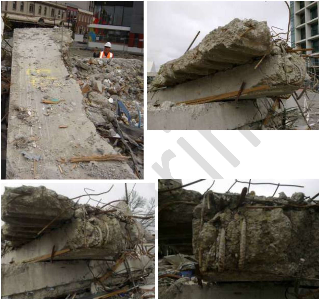
Figure 5 Pre-cast shell beam (Item E14) from northern face Grid 4, west side of lift core (DENG B23 Dwg S18 (Figure 59)). (clockwise from top left) a) Top face with slab fracture along edge of shell beam, extending out further at far end adjacent to lift core attachment; b to d) Fractured slab outstand remnant at east end from which slab concrete cores were extracted. The bottom H24 bars from shell beam have been turned back into the concrete infill rather than embedded in shear wall as specified (DENG Detail 5 Dwg S19). Refer also bar imprint on wall at the connection seen in Figure 22 at Level 4 and Figure 23 at Level 3.
