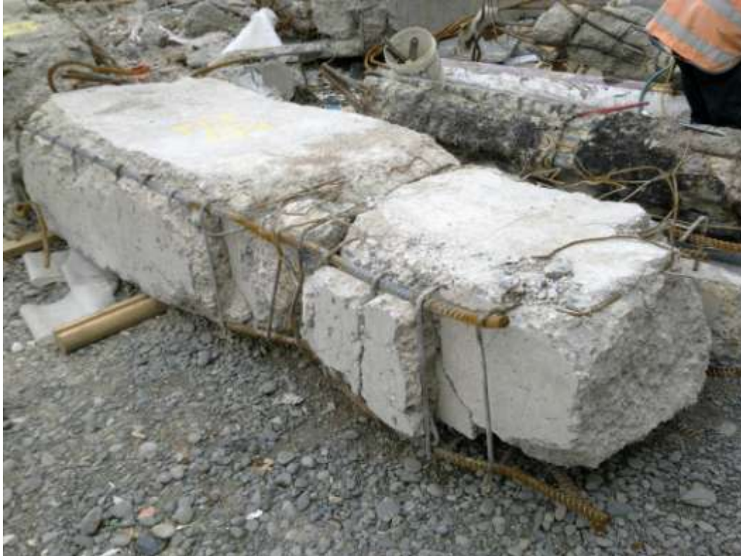
Figure 4 Edge shell beam Item E6 showing unreinforced concrete infill and smooth interface between shell beam and in-fill. The DENG Specification Precast Concrete cl 3.12 required roughened interface surfaces (Figure 71).
