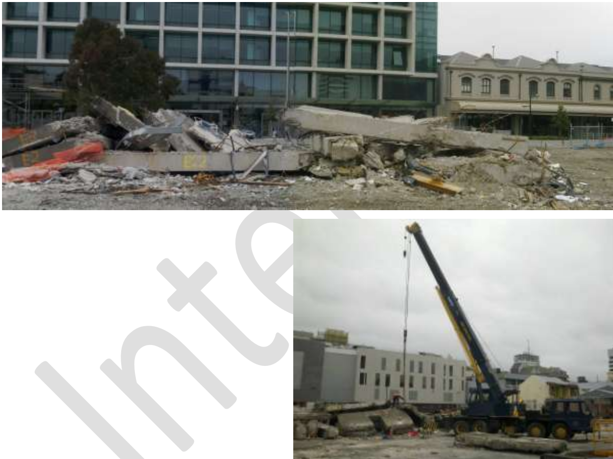
Figure 1 USAR structural debris pile on CTV site (top to bottom) a) At start of site examination; b) Crane used to move debris remnants for examination
