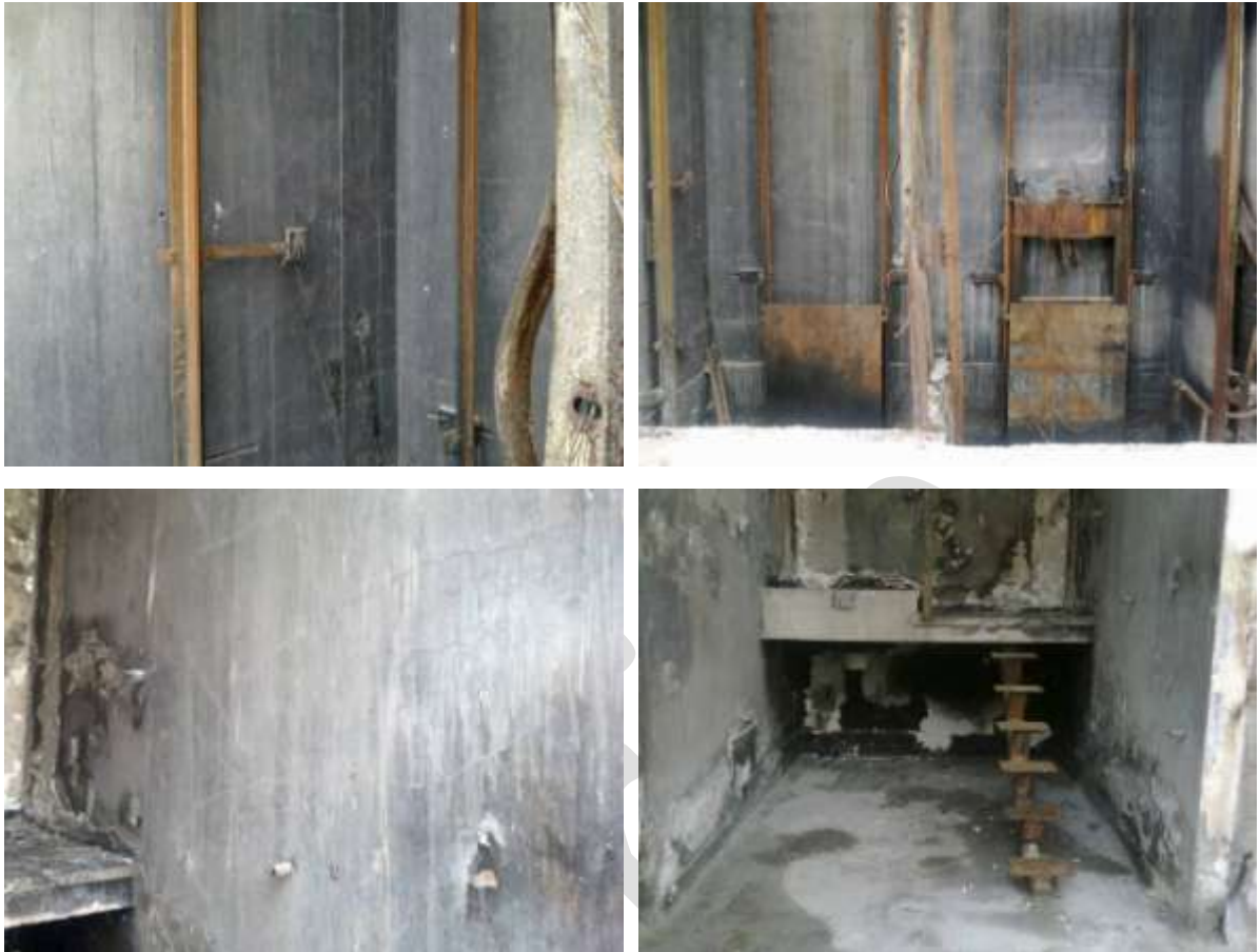
Figure 19 Lift and Stair well wall cracking Level 1 to Level 2 (clockwise from top left) a) Lift wall face of Line D wall with fine diagonal shear cracking in both directions; b) Lift wall face of Line 5 wall with fine diagonal cracking in both directions; c) Stairwell area with steel stair stringer where concrete cores were extracted; d) Stair well face of Line D wall with fine diagonal cracking in both directions.
