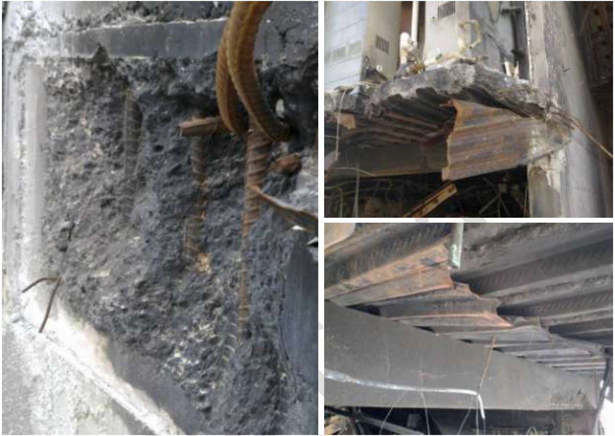
Figure 22 Line 4 Core Walls Level 4 slab remnants (top to bottom) a) Connection of shell beam to wall with two fractured H24 top bars and two de-bonded top bars. No bottom bars from shell beam embedded in wall but imprints from bars evident (DENG B23 Dwg S18 (Figure 59), Detail 5 S19 (Figure 64)), corresponding to the bent back bottom steel in shell beam Item E23 (Figure 6). b) Fractured vertical face of slab at stairwell wall, with fractured slab support beam (DENG B25 Dwg S18 (Figure 59)) top bar and charred fracture surface. c) Torn Hi-bond sheeting de-bonded from slab but still fixed in at pre-cast beam support.
