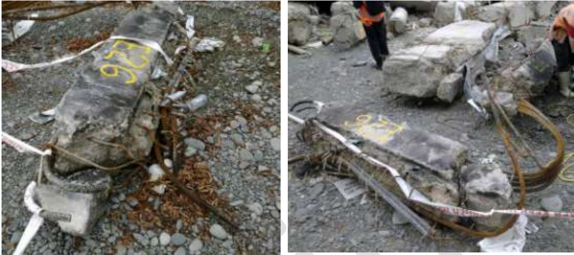
Figure 9 Interior Pre-cast Log Beam from Line 2 and 3 (DENG Section 3 Dwg S15 (Figure 58)) (left to right) a) Diagonal shear damage at end and smooth formed surface at beam-column joint; b) Mid-portion of beam concrete has broken away and stirrups are pulled apart.
