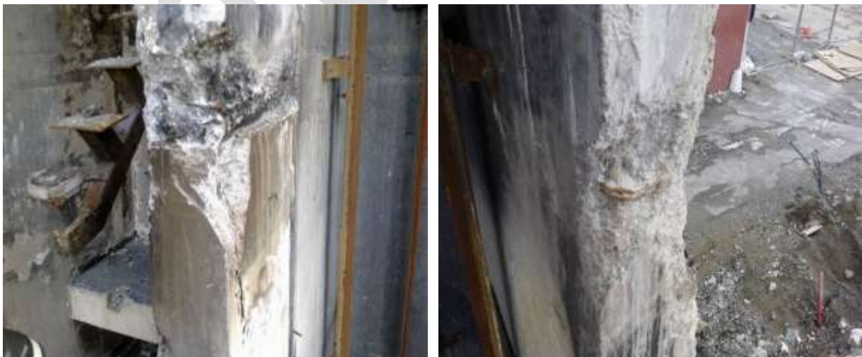
Figure 27 Level 2 Lift Well Wing Walls Grid D and D.5 (left to right) a) 20 mm hole in end where a reinforcing bar has pulled out of wall. 200 mm thick construction joints in wall at slab level. b) No reinforcing steel attachment into the east wing wall at Level 2
