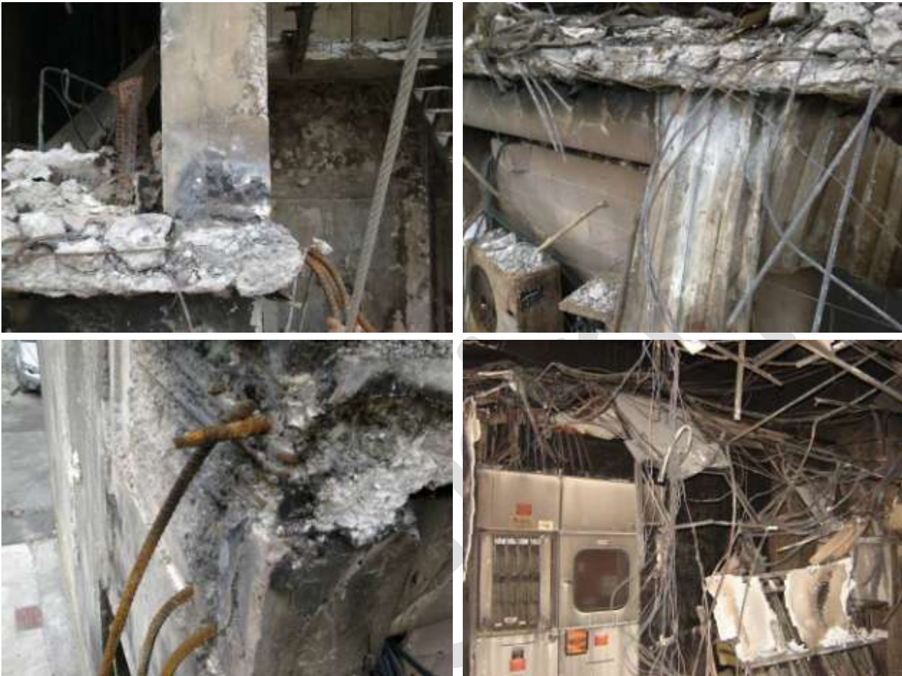
Figure 24 Line 4 Core Walls Level 2 slab remnants (clockwise from top left) a) Slab edge broken back during de-construction adjacent to stairwell wall; b) Broken back slab with H12 saddle bars exposed. Masonry wall with separation along top course; c) Switch room under Level 2 slab; d) Connection of shell beam to wall with two fractured H24 top bars and one de-bonded top bars. Bottom bars from shell beam have been embedded in wall as specified (DENG B23 Dwg S18 (Figure 59), Detail 5 S19 (Figure 64)). Some diagonal beam-wall joint zone shear cracking can be seen in the wall end.
