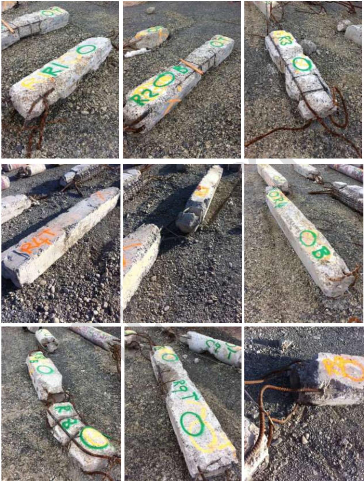
Figure 48 400 x 300 mm Rectangular Columns (Left to right, top down) a) R1 beam-column joint failure at base, mid-height failure; b) Level 6 to Roof base or beam-column joint failure; c) R 3 failure base and top; d) R4 Level 6 to Roof with beam-column joint failure, still connected by rebar to e) R4' below which also f) indicates beam-column joint failure at R4' base (near camera); g) R8 with damage from mid-height still connected to R9 above h) with beam-column joint failure with i) underside of R9 smooth.
