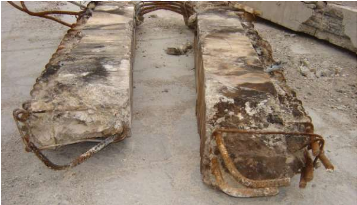
Figure 10 Interior Pre-cast Log Beams from Line 2 and 3 (DENG Section 3 Dwg S15 (Figure 58)) showing smooth concrete formed for beam-column joint and bottom hooked bars that have pulled out of beam-column joints without any obvious straightening; metal decking has pulled away from slab seating; no slab remains attached to the beams
