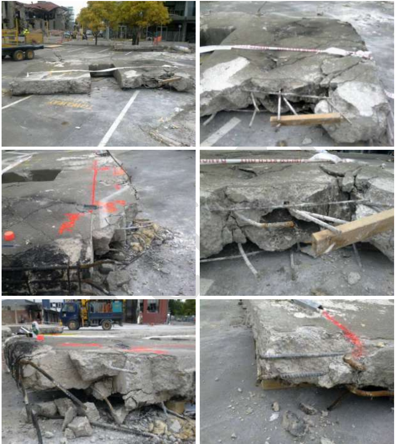
Figure 15 Line 1 Shear Wall Level 4 to Level 5 (Item E4) (clockwise from top left) a) Outer face with east pier on right with severe shear damage, and timber formwork remnant; b) and c) Charring on fractured concrete surfaces prior to deconstruction; d) Top west corner showing saw-cut on top edge from deconstruction; e) Top east corner showing smooth construction joint at interface with pre-cast beam B15 (DENG Dwg S18 (Figure 59)) and fire charring to spalled eastern edge; f) View from east to west of top east corner construction joint notch.
